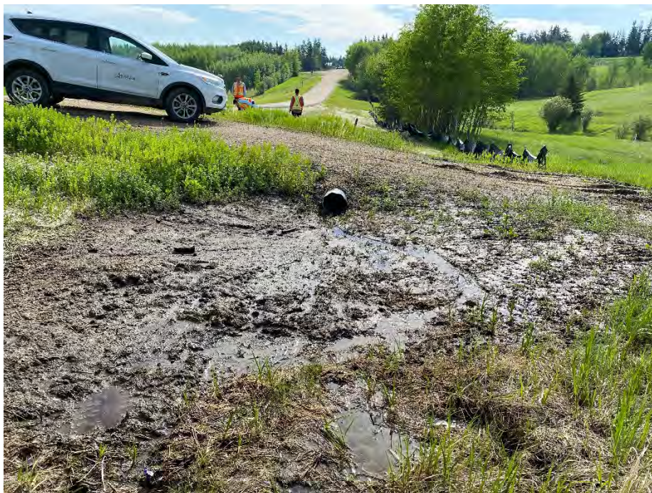
Photo 6: Wet ground and erosion at west end of culvert across property access road. Looking east.
