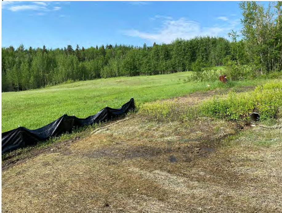
Photo 5: Wet ground and erosion at east end of culvert across property access road. Looking southwest.
