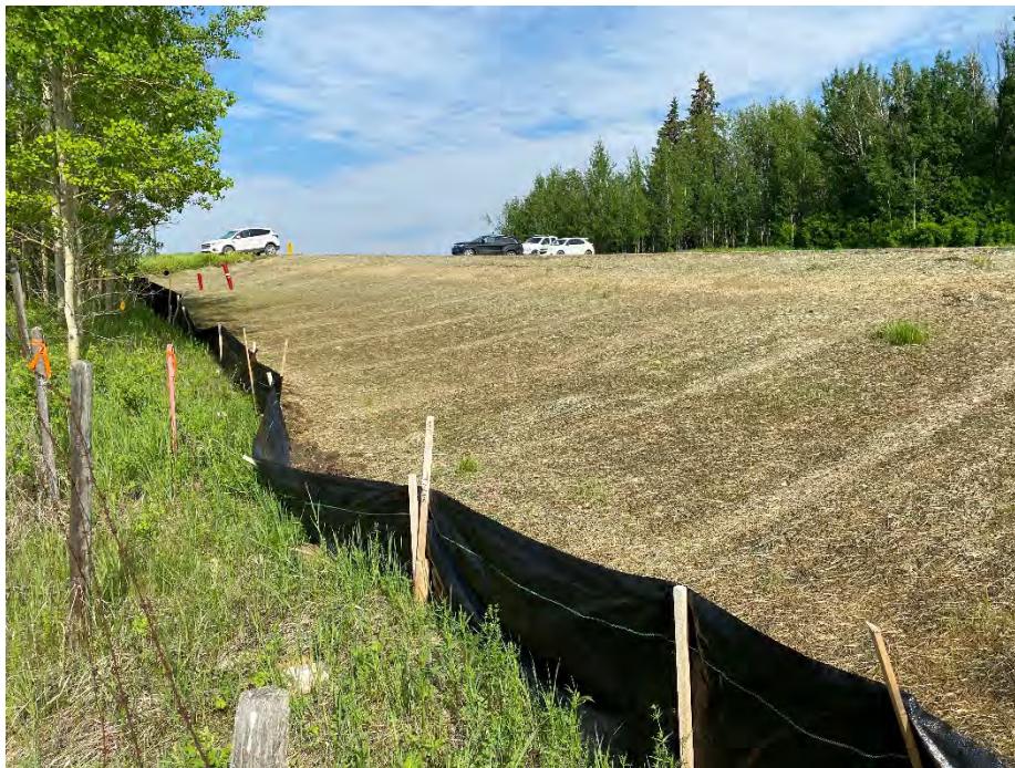
Photo 8: Upslope from previous location of exposed Telus cable. Looking northwest.
