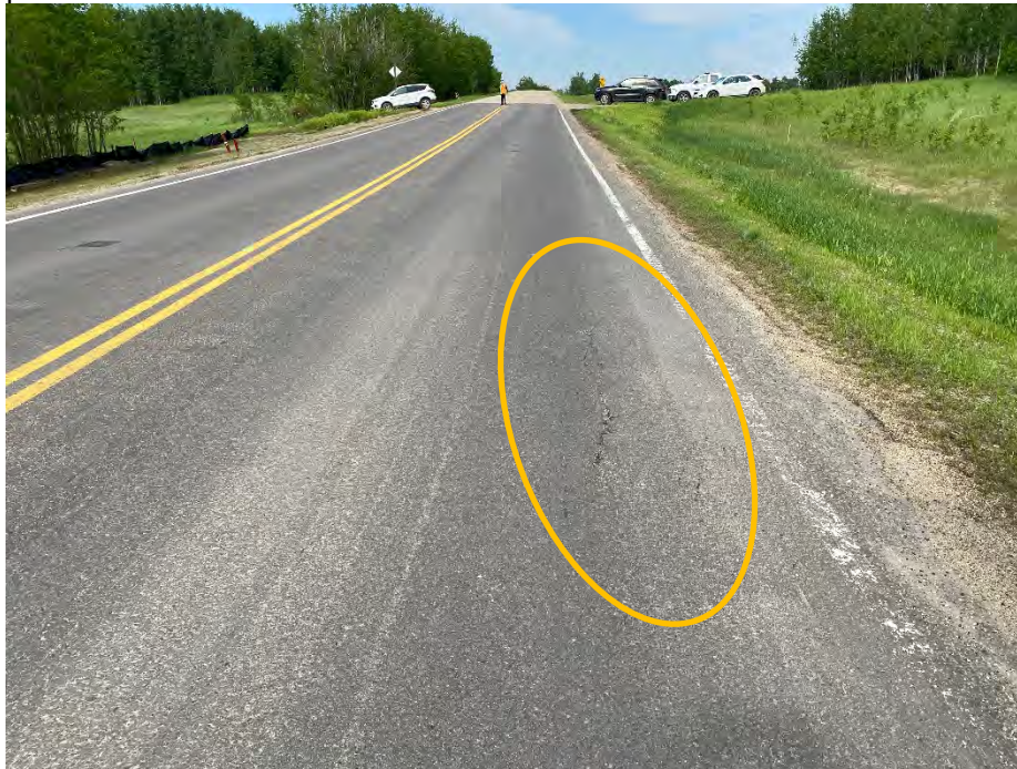
Photo 3: Pavement cracking in westbound lane. Looking west.
