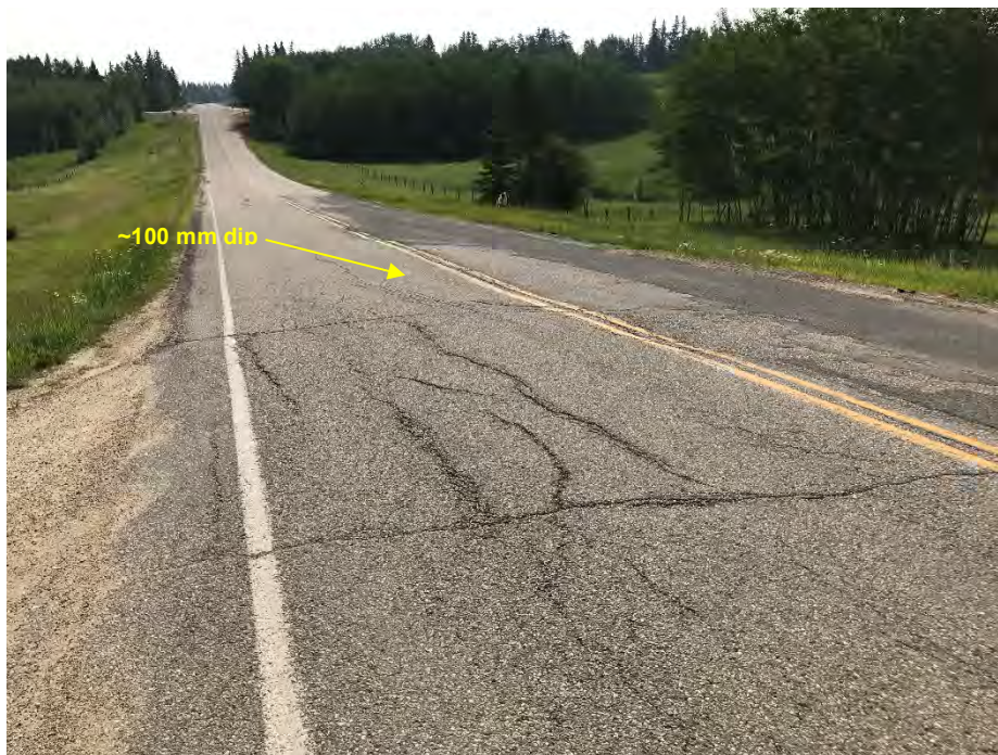
Photo 2: Pavement cracking along Highway 16A. Patch placed on eastbound lane. Looking north.
