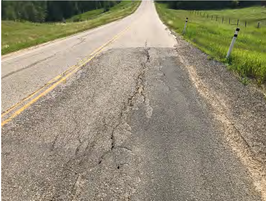
Photo 3: Pavement cracks at east limits of patch. Looking east.
