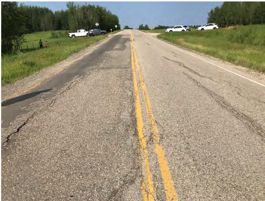
Photo 4: Pavement cracks at east limits of patch. Looking west.
