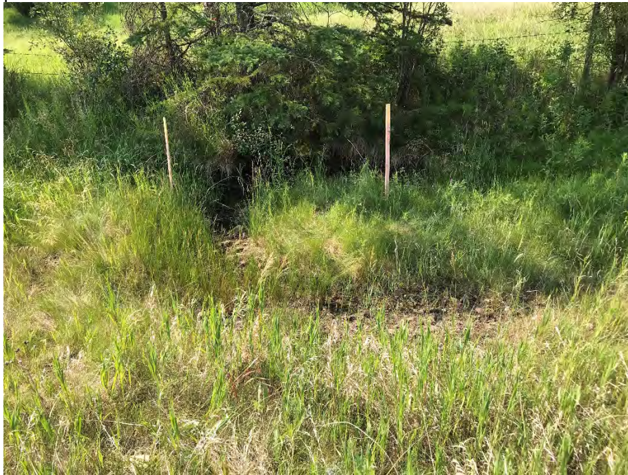
Photo 5: Erosion upslope from exposed Telus cable. Looking south.
