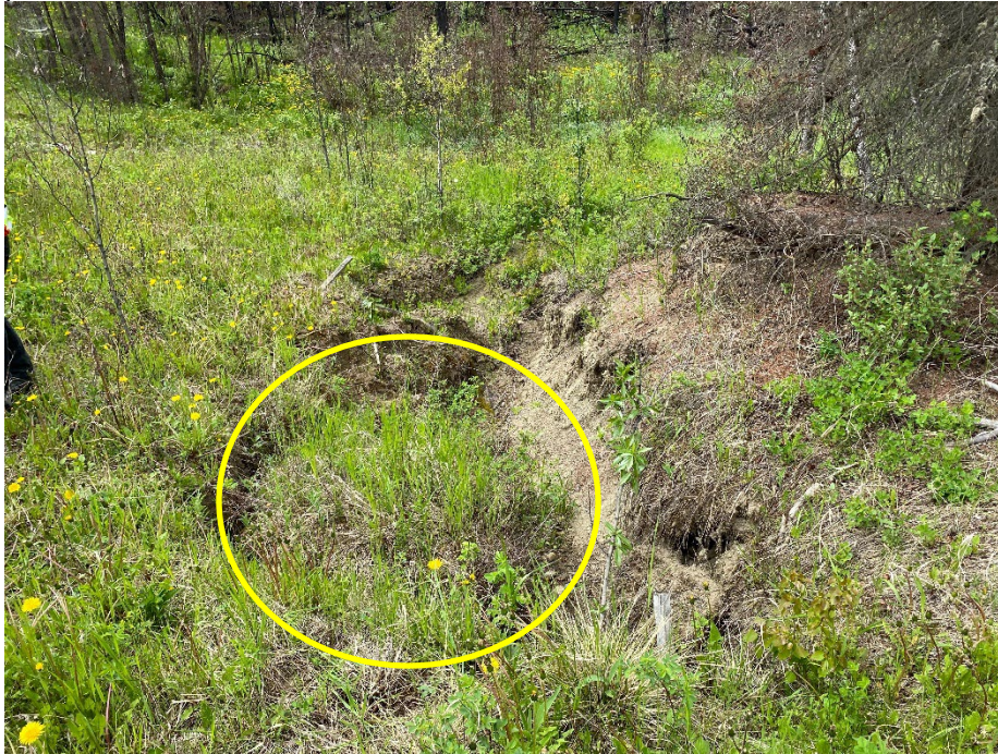
Photo 5: Erosion gully north of 1200 mm diameter culvert inlet. Portion of slope has slid into gully. Looking southwest.
