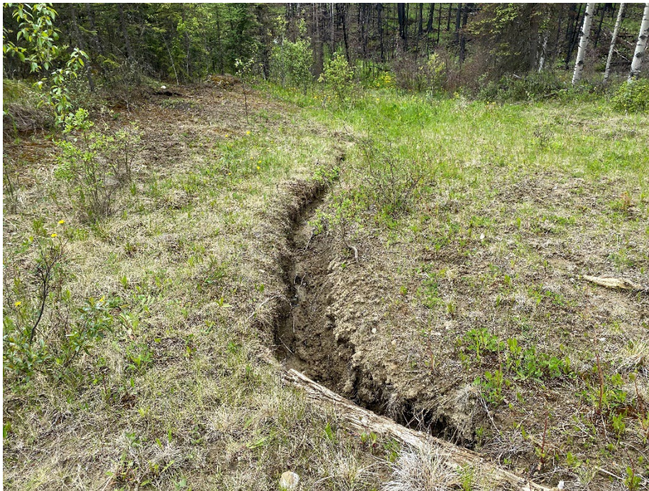
Photo 6: Erosion gully leading to old gully shown in Photo 5. Looking southwest.
