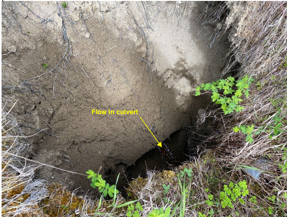
Photo 3: Scour hole exposing 90 mm separation in 760 mm diameter culvert. Looking west.
