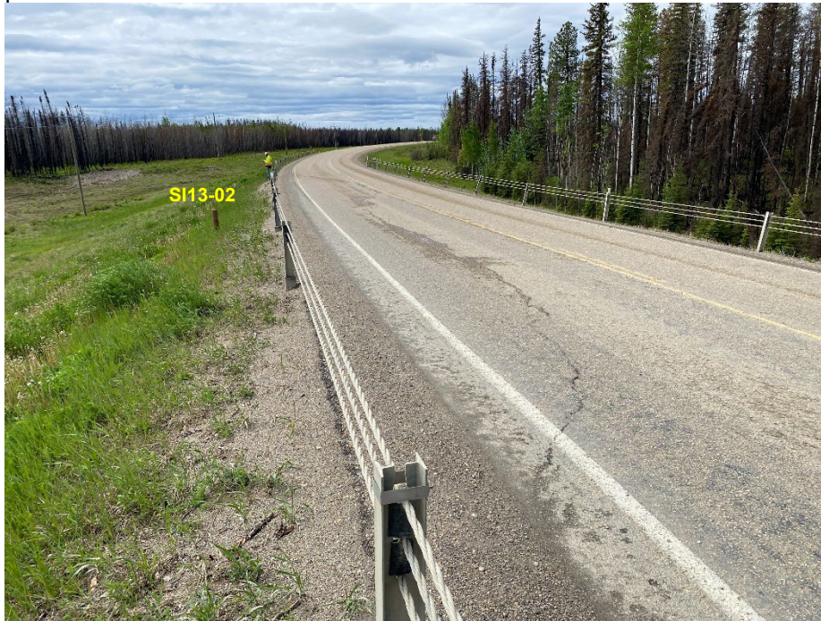
Photo 1: Arched crack near SI13-02. Looking southwest.
