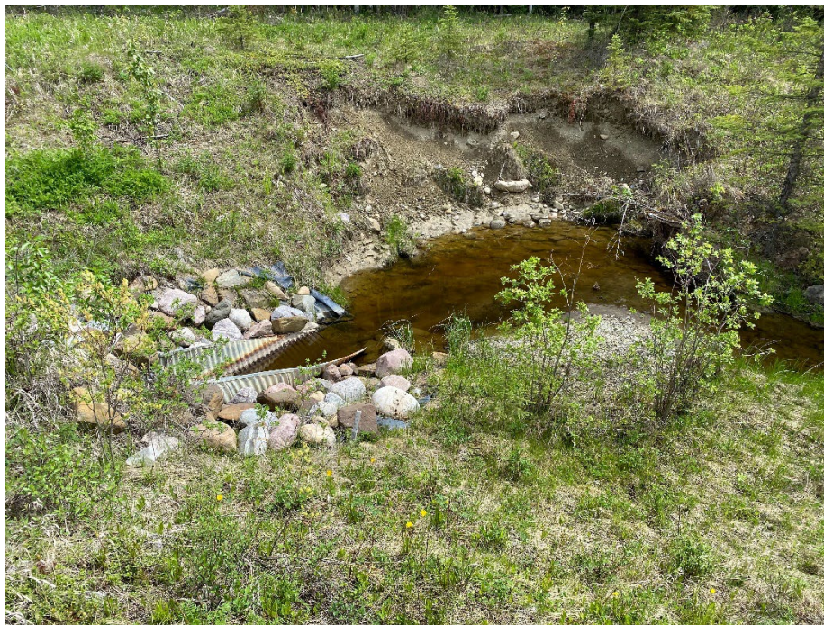
Photo 4: Retrogressing slump/erosion at outlet of 1200 mm diameter culvert. Looking east.
