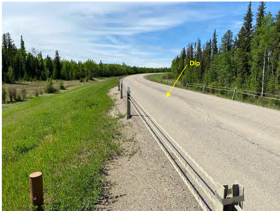
Photo 2: Pavement dip near south end of overlay. Looking southwest.
