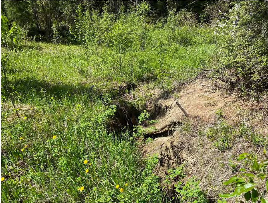
Photo 5: Erosion gully north of 1200 mm diameter culvert inlet. Looking southwest.
