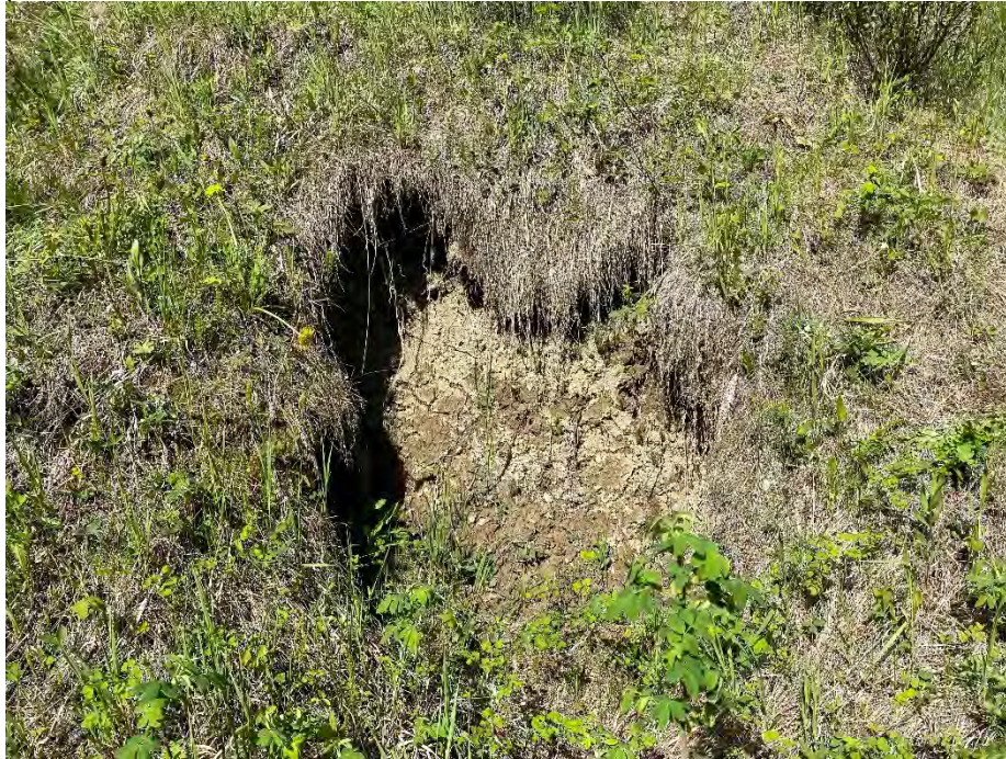
Photo 3: Scour hole above 760 mm diameter culvert. Looking west.
