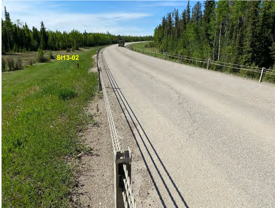
Photo 1: Arched crack near SI13-02. Looking southwest.
