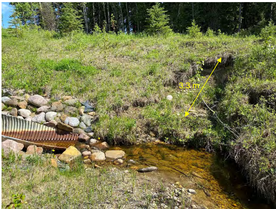
Photo 4: Slump/erosion at outlet of 1200 mm diameter culvert. Looking east.
