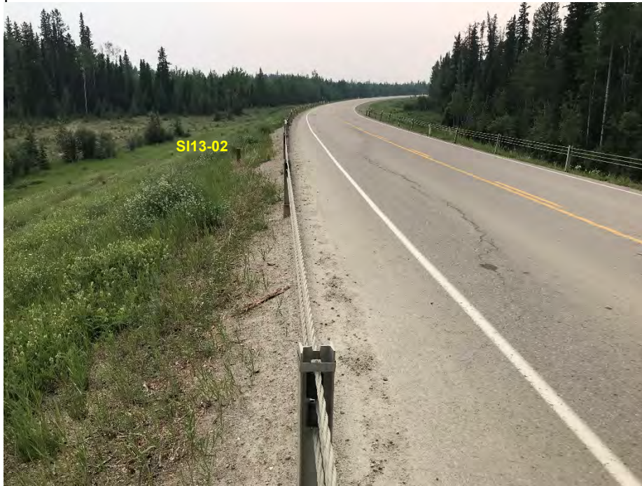
Photo 1: Arched crack near SI13-02. Looking southwest.
