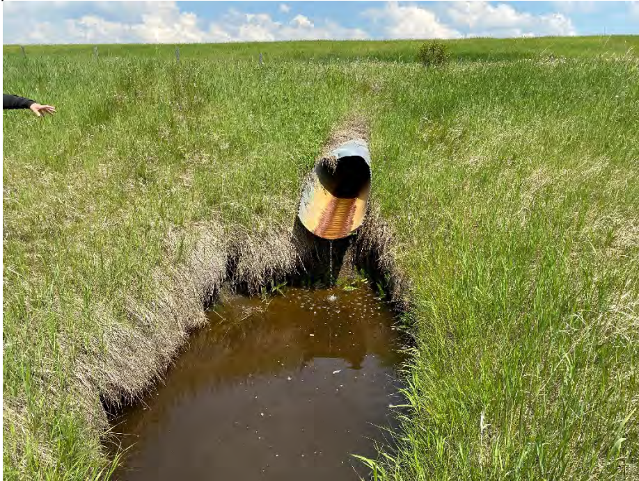
Photo 7: Eroded channel at culvert outlet southeast of SI14-27 filled with water. Looking northeast.
