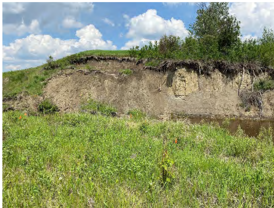
Photo 2: Bank erosion progressing east from westbound bridge. Looking north.
