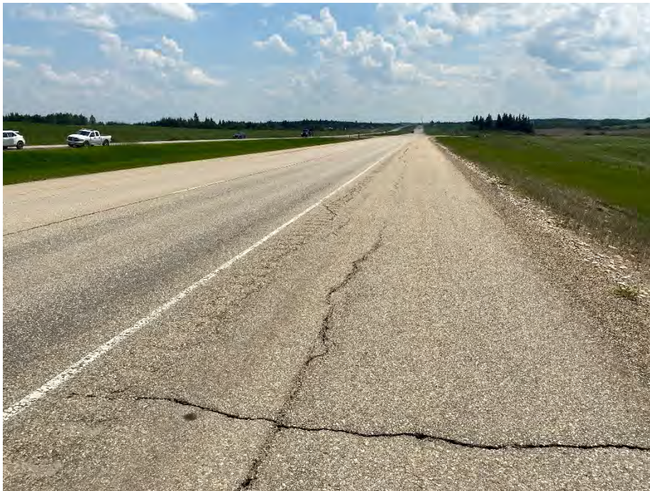
Photo 6: Pavement cracks, southwest of SI14-26. Looking southeast.
