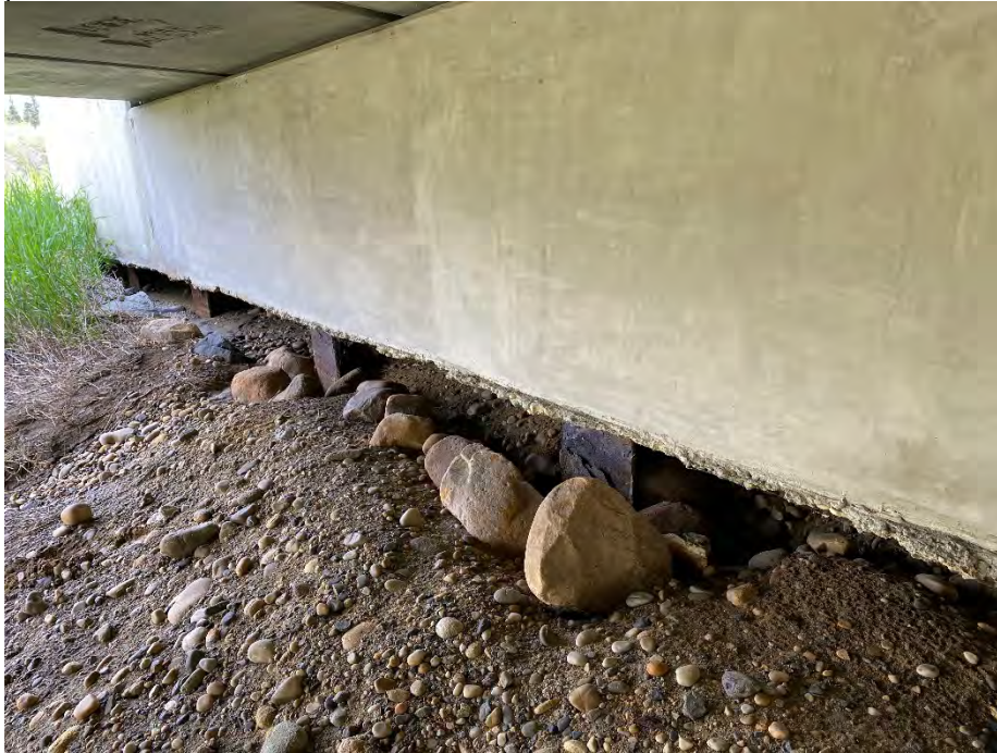
Photo 3: Corrosion on exposed H-piles under south abutment of westbound bridge. Looking east.
