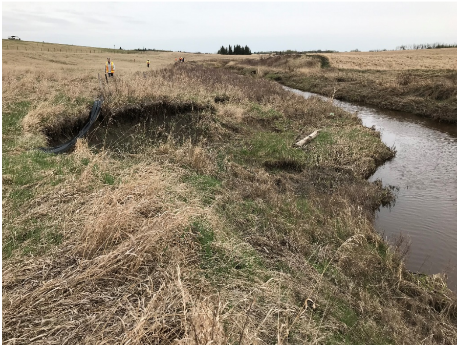
Photo 3: Retrogressing scarp along well vegetated slope and banks. Looking southeast.
