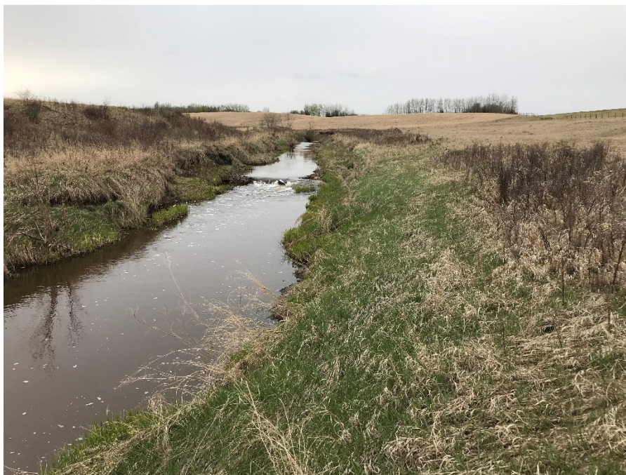
Photo 6: River bank erosion and slumping along. Looking northwest.
