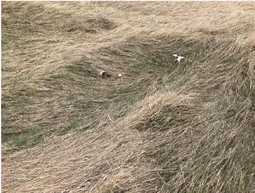
Photo 7: Low spot at subdrain outlet. No water observed at outlet. Looking southeast.
