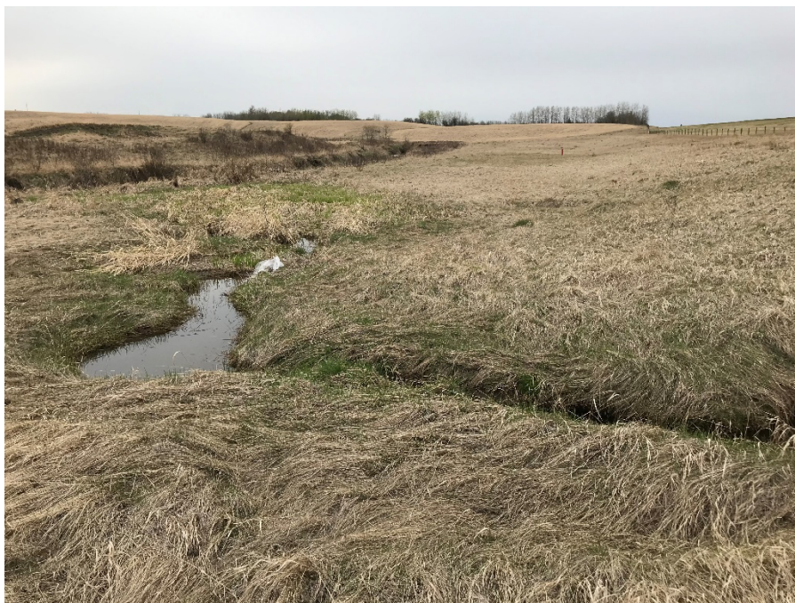
Photo 2: Eroded channel at culvert outlet southwest of SI14-27 filled with water. Looking west.
