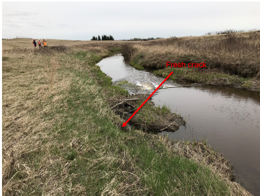
Photo 5: Slumping along southeast meander. Some fresh cracks visible. Looking southeast.
