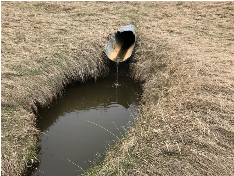
Photo 1: Eroded channel at culvert outlet southwest of SI14-27 filled with water. Looking northeast.
