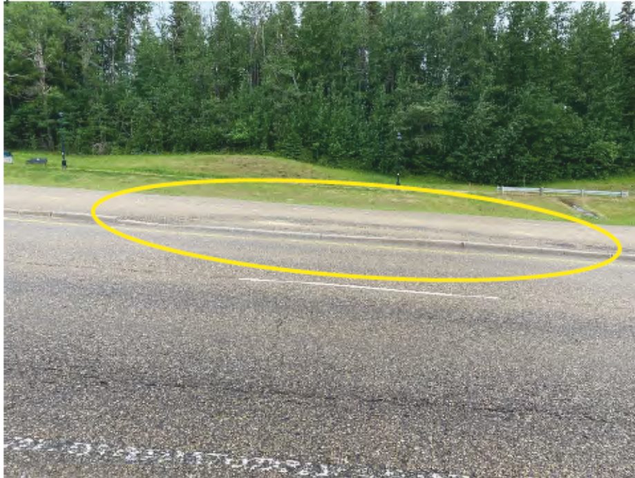
Photo 3: Visible dip in median at approximately STA 1+845. Looking southwest.
