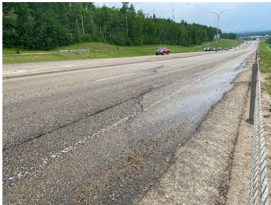
Photo 2: West crack at approximately STA 1+850. Cracking on westbound lane reflecting through 2014 overlay. Looking west.
