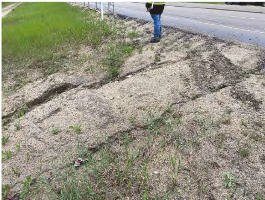
Photo 4: Erosion gullies at approximately STA 1+750. Looking southeast.
