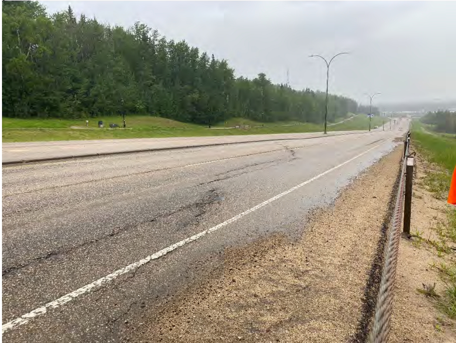
Photo 1: East crack at approximately STA 1+920. Looking west.
