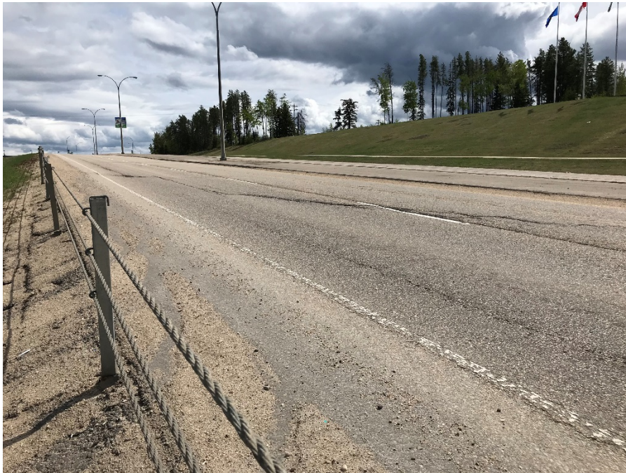
Photo 1: East crack at approximately Sta 1+920. Looking west.
