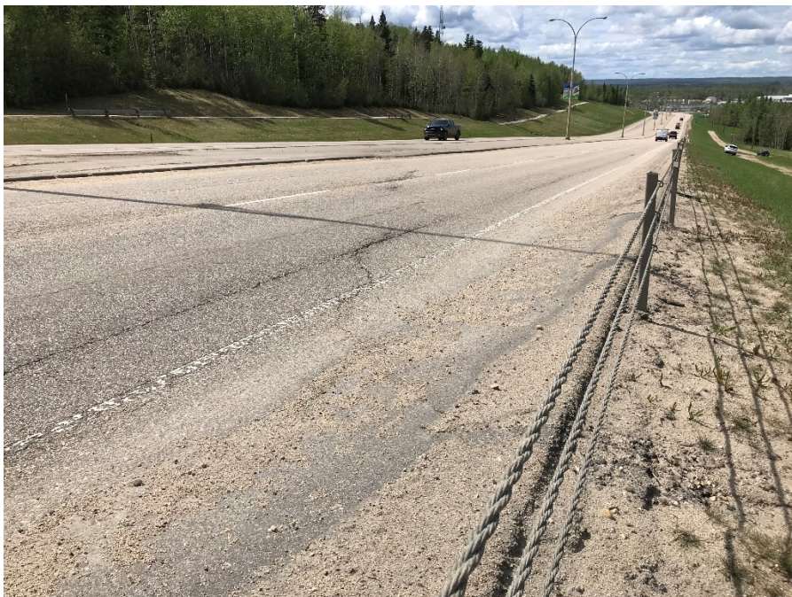
Photo 2: Approximately Sta 1+850. Cracking on westbound lane reflecting through 2014 overlay. Looking west.
