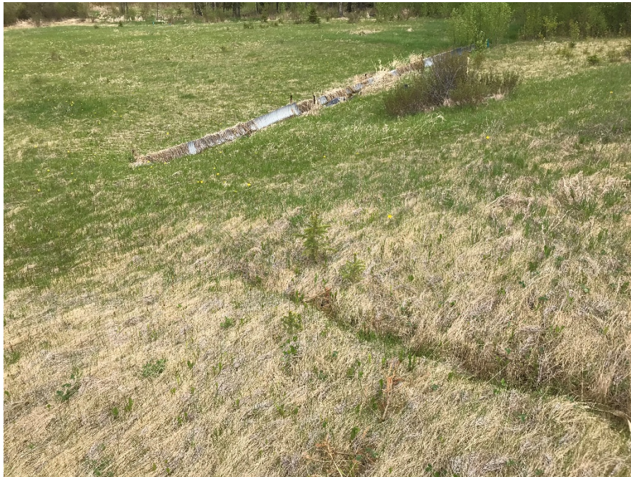
Photo 5: Erosion gully upslope from half-culvert. Looking east.
