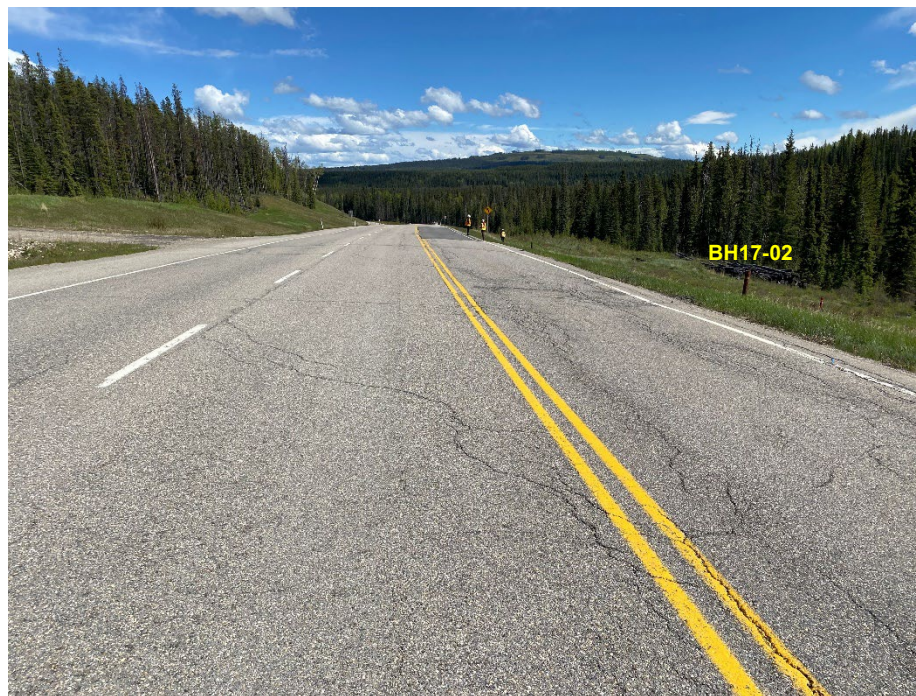
Photo 2: Pavement cracking on highway near BH17-02. Looking southeast.
