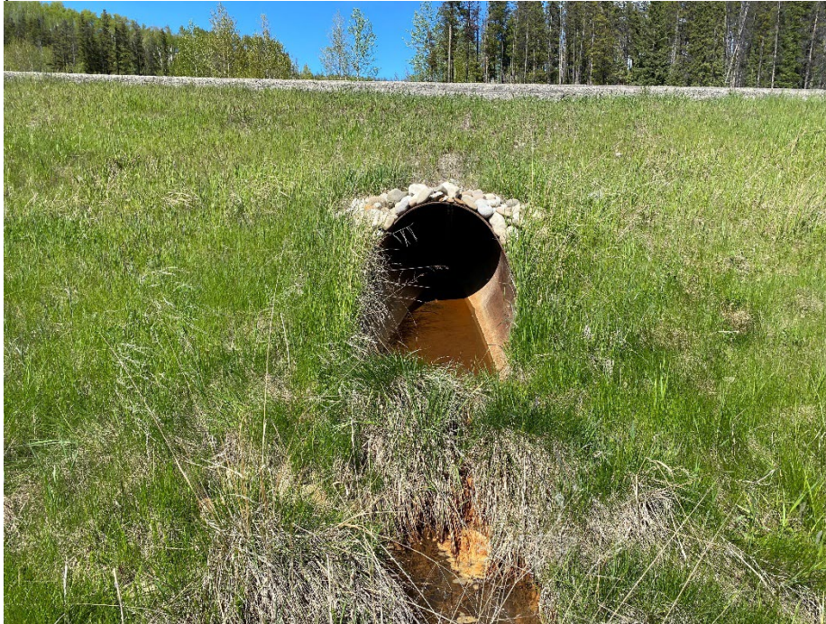
Photo 7: Vegetation blocking C/L culvert outlet. Looking northeast.
