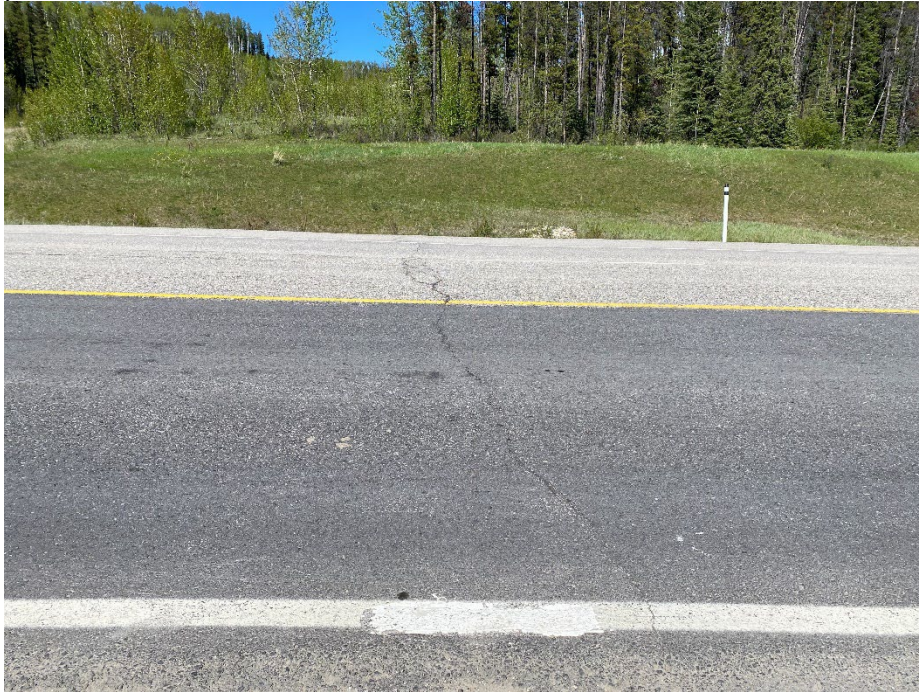
Photo 5: Pavement crack along C/L culvert alignment. Looking northeast.
