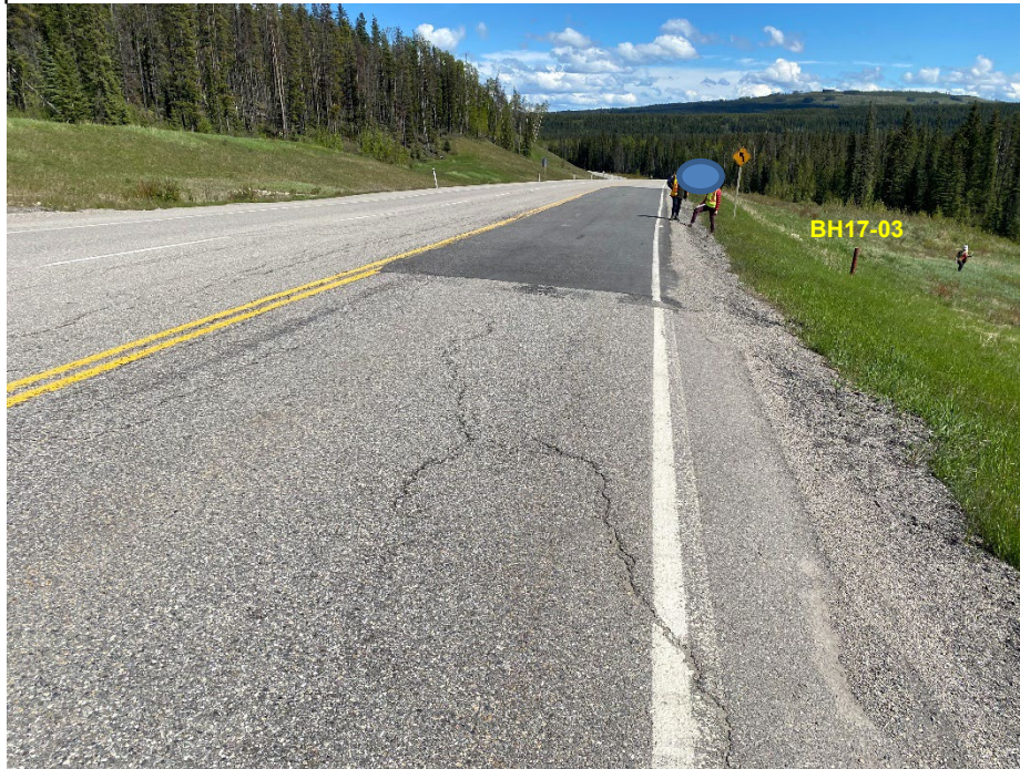
Photo 3: Pavement cracking in SBL between BH17-02 and BH17-03. SBL milled and filled. Looking southeast.
