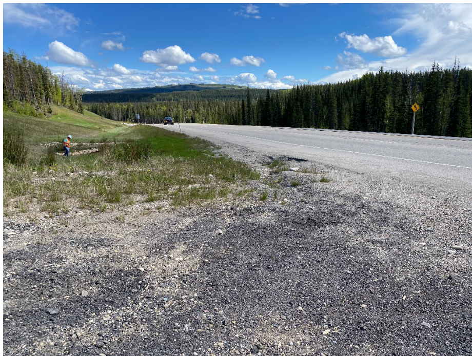
Photo 4: Minor erosion at edge of pavement at east corner of entrance to gravel pit. Looking southeast.
