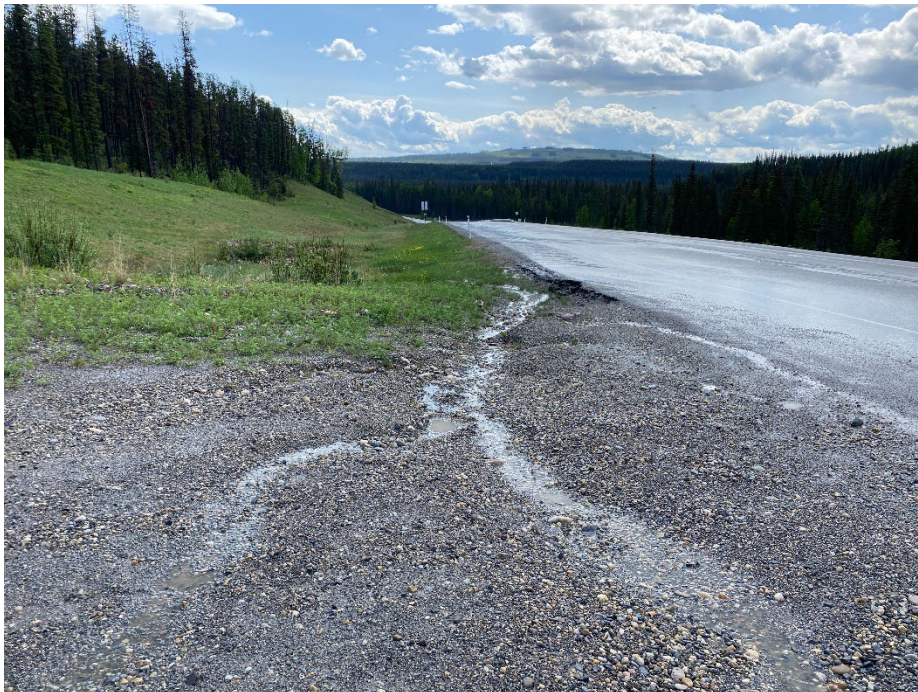
Photo 4: Surface water eroding gravel and edge of pavement at east corner of entrance to gravel pit. Looking southeast.
