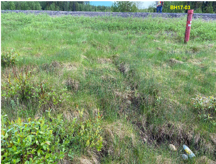
Photo 8: Seepage in vehicle track. 300 mm deep track. Looking northeast.
