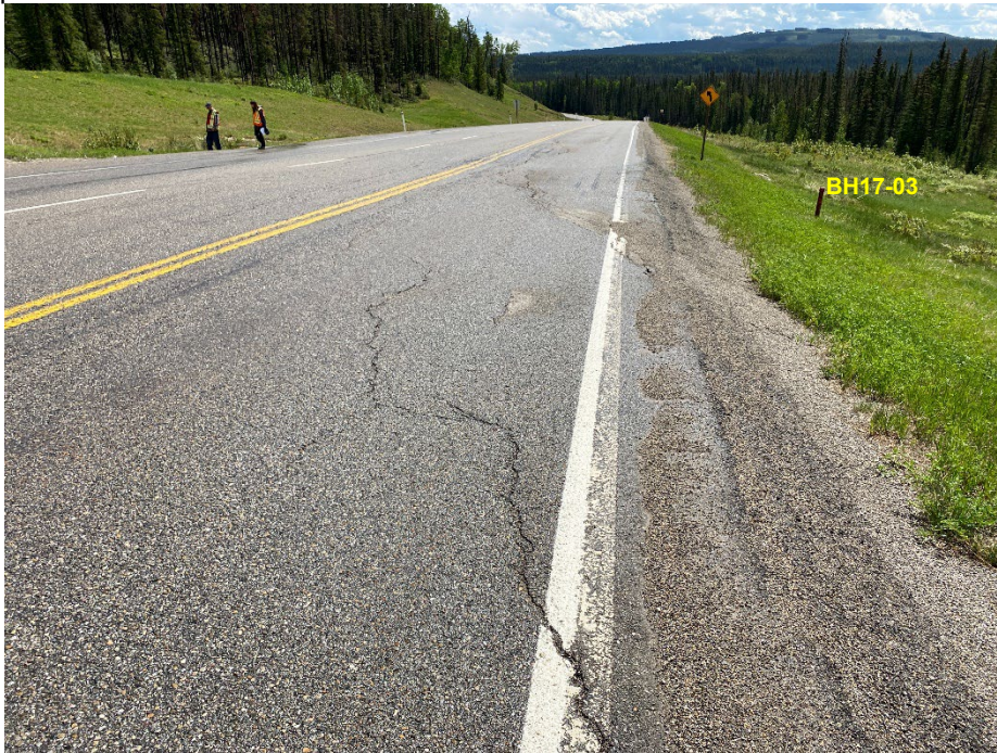
Photo 3: Pavement cracking in SBL between BH17-02 and BH17-03. Looking southeast.
