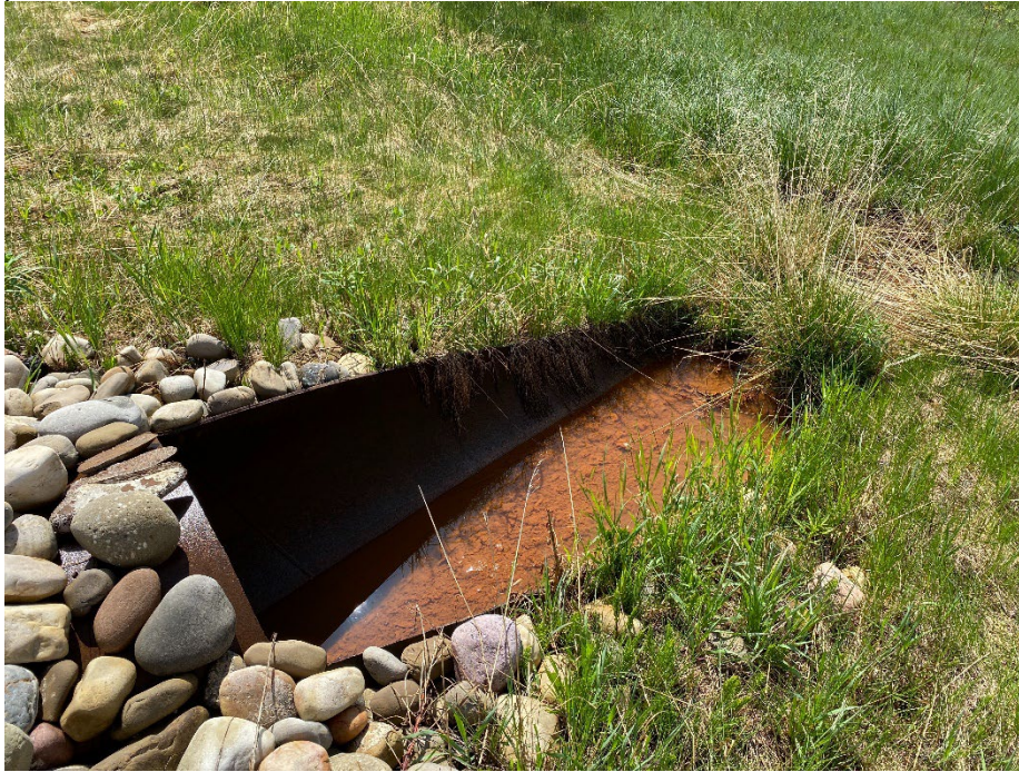
Photo 7: Vegetation blocking C/L culvert outlet. Looking southeast.
