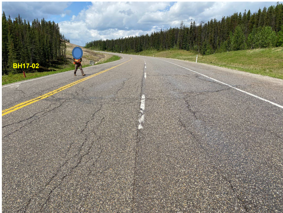
Photo 2: Pavement cracking in NBL near BH17-02. Looking northwest.
