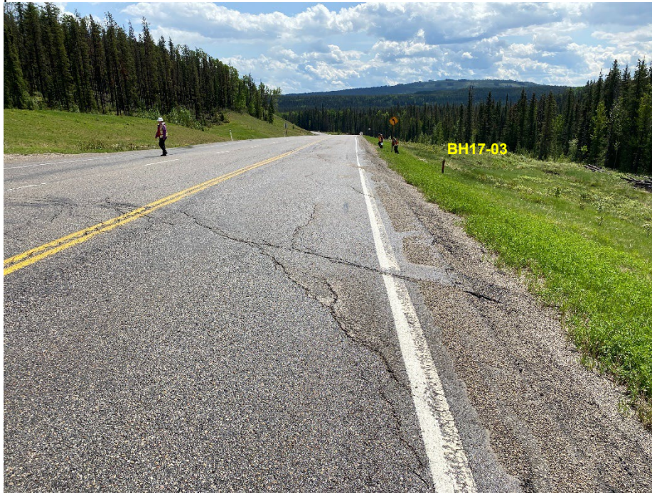
Photo 1: Pavement cracking in SBL near BH17-02. Looking southeast.
