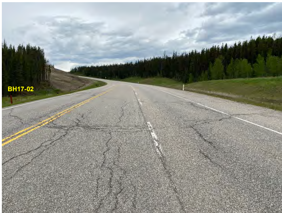
Photo 2: Pavement cracking near BH17-02. Looking northwest.
