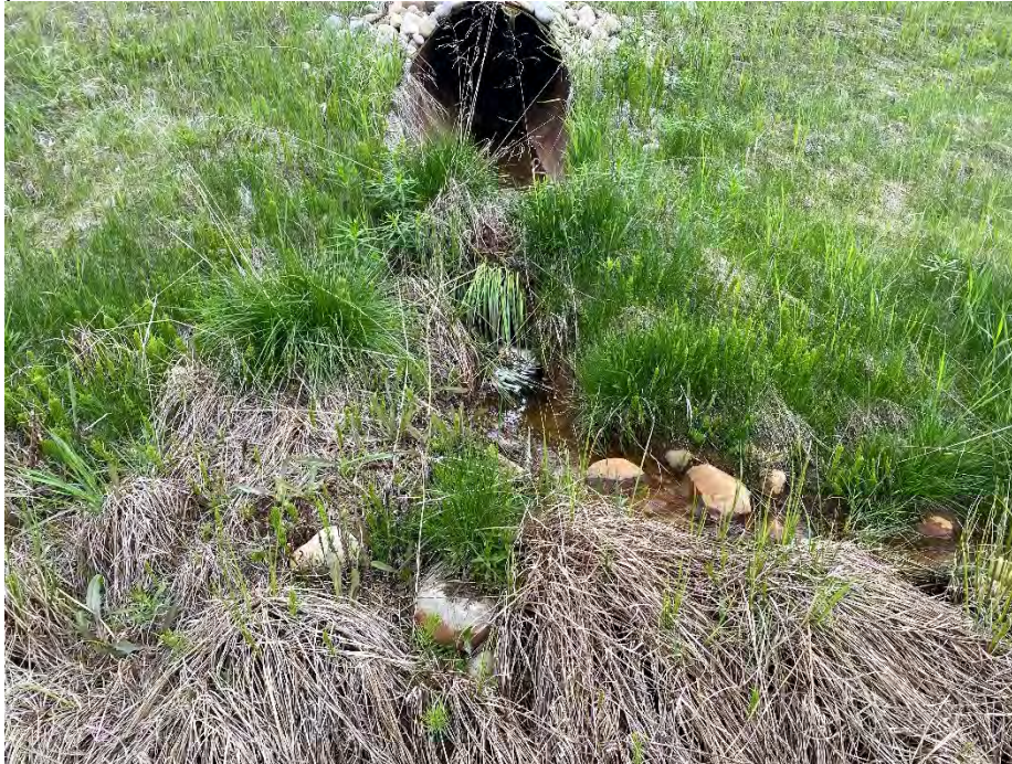
Photo 5: Erosion at C/L culvert outlet. Looking northwest.
