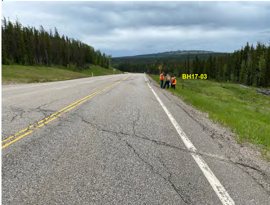
Photo 1: Pavement cracking in SBL. Looking southeast.
