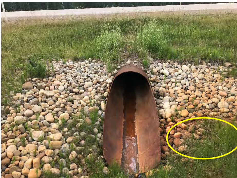
Photo 4: North ditch at C/L culvert inlet. Seepage location circled. Looking southwest.
