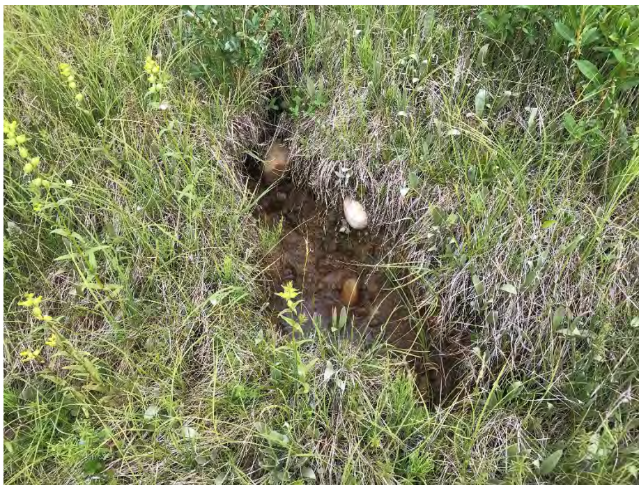
Photo 6: Seepage in vehicle track. 300 mm deep track. Looking down.
