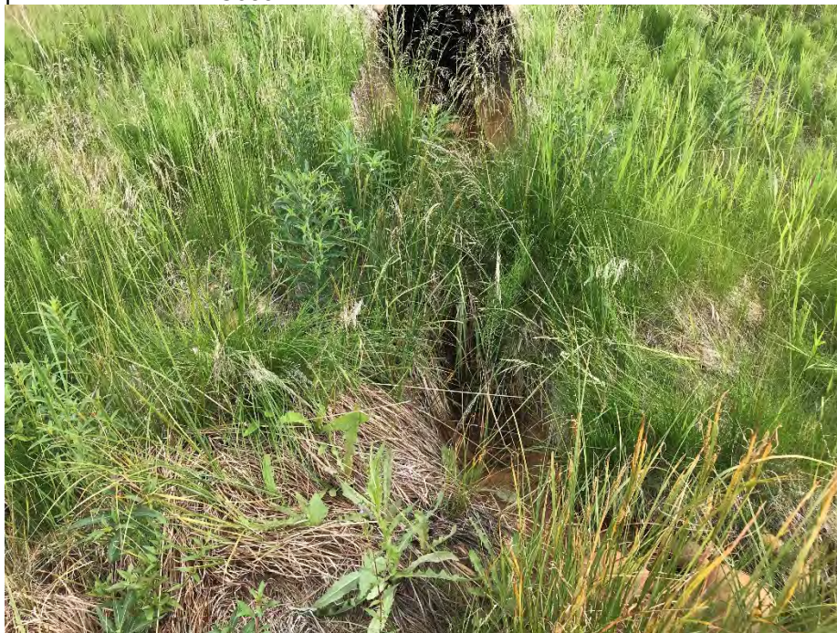
Photo 5: Erosion at C/L culvert outlet. Looking northwest.
