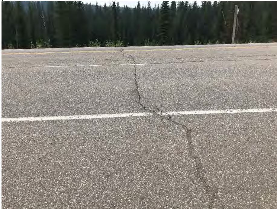
Photo 3: Pavement crack along C/L culvert alignment. Looking southwest.
