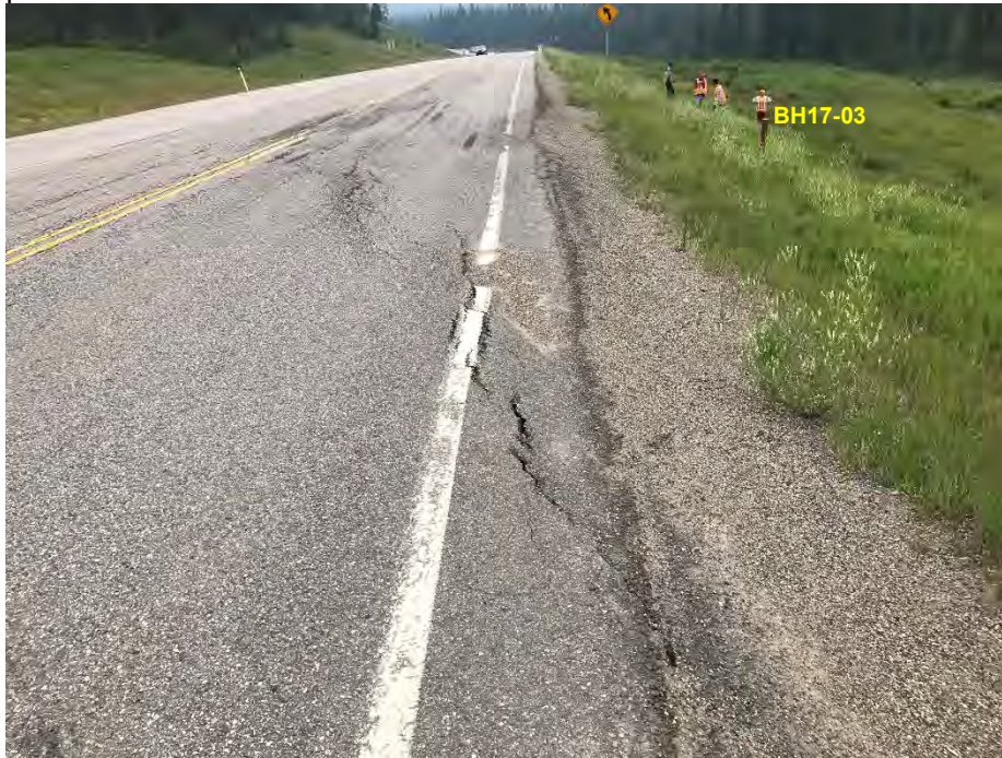
Photo 1: Pavement cracking at shoulder of SBL. Note tire marks just past the crack. Looking southeast.
