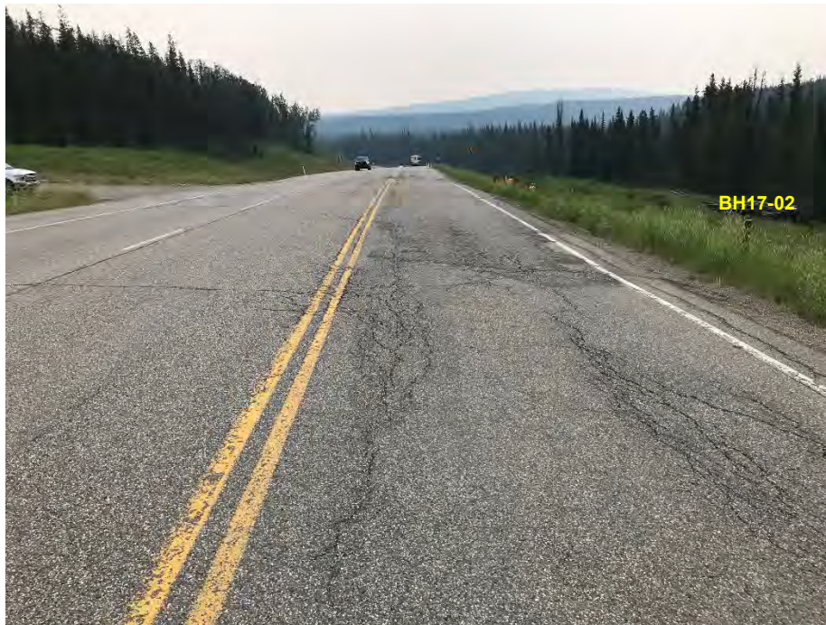
Photo 2: Pavement cracking near BH17-02. Looking southeast.
