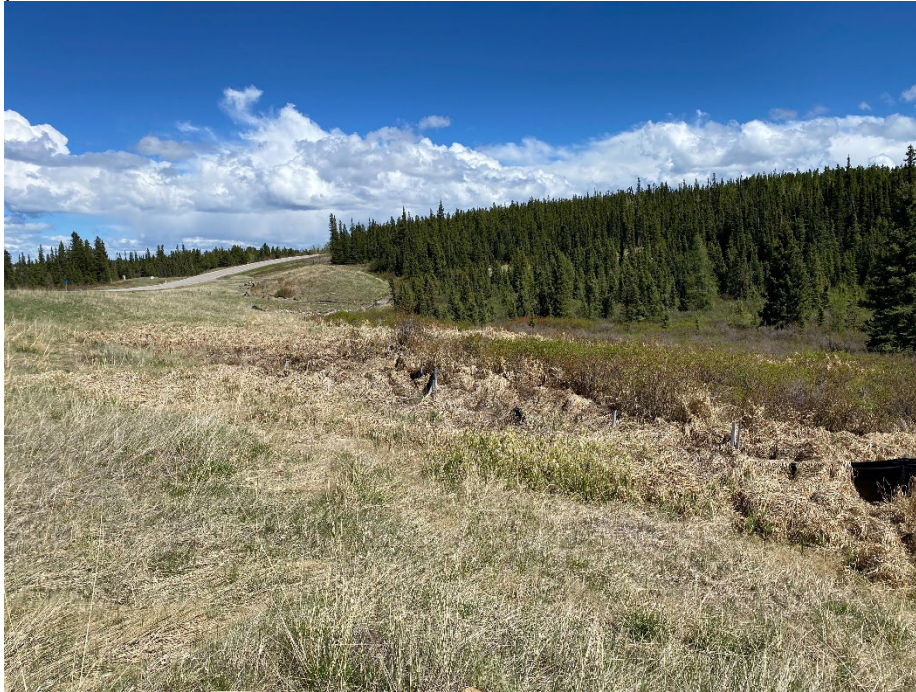
Photo 5: Previous areas of seepage were dry. Silt fence remains on site. Looking east.
