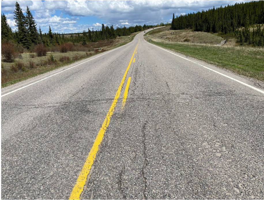
Photo 3: Pavement cracks at east end of patch. Looking east.
