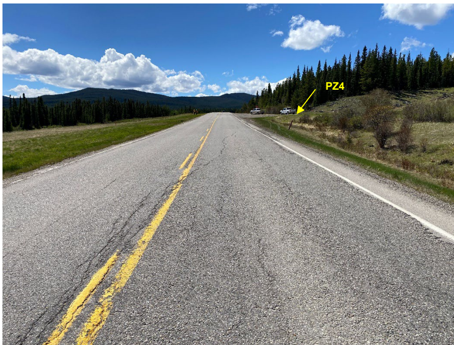
Photo 2: Pavement cracking east of PZ4. Looking west.
