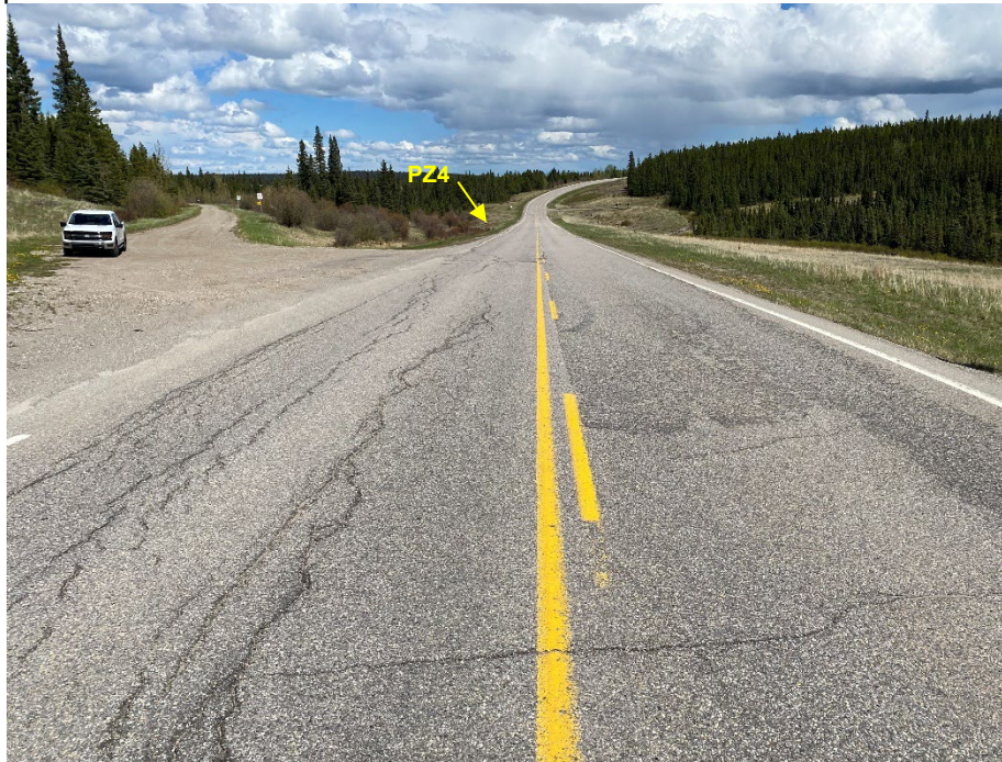
Photo 1: Pavement cracks in front of access road. Looking east.
