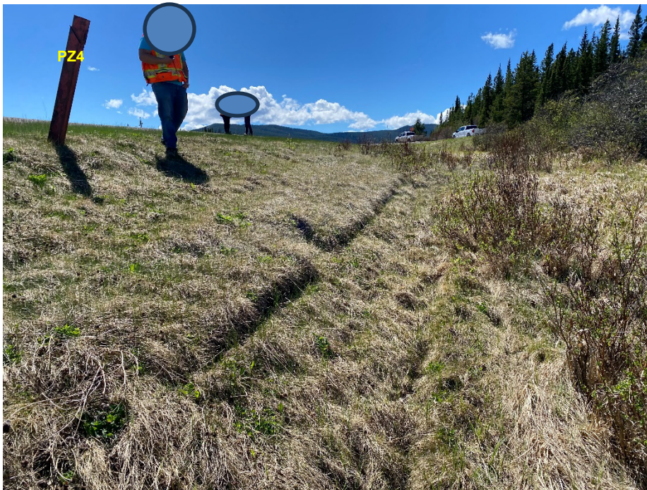
Photo 6: Ground crack in north ditch, near PZ4. Looking west.
