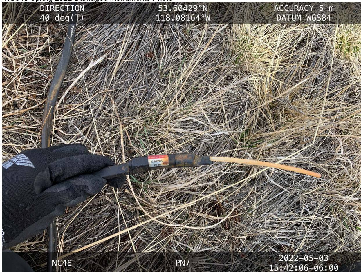
PZ7 Piezometer tubing was damaged.
