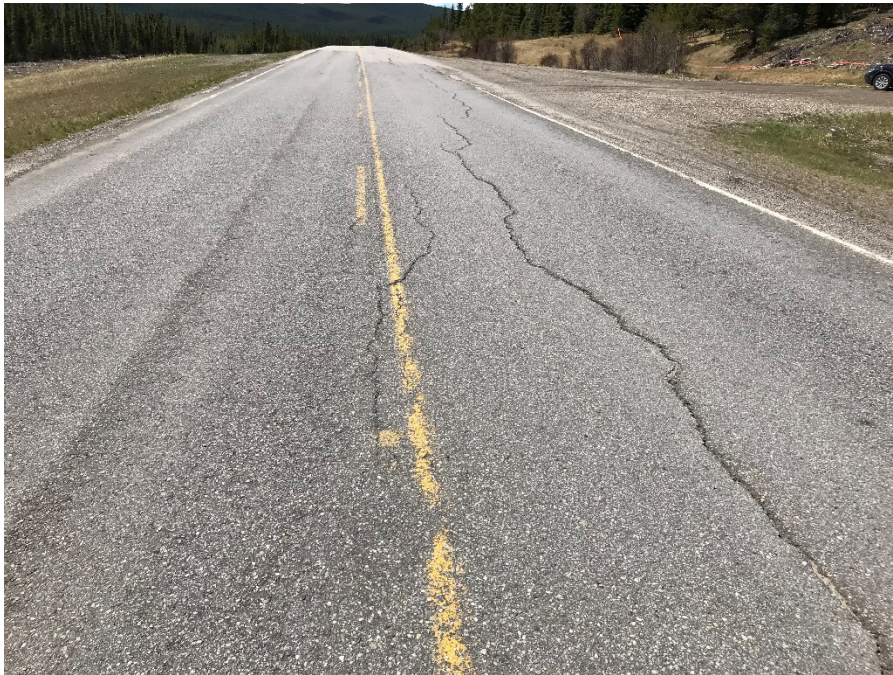
Photo 1: Pavement cracks in front of access road. Looking west.
