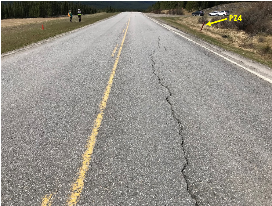
Photo 3: Pavement cracking east of PZ4. Looking west.
