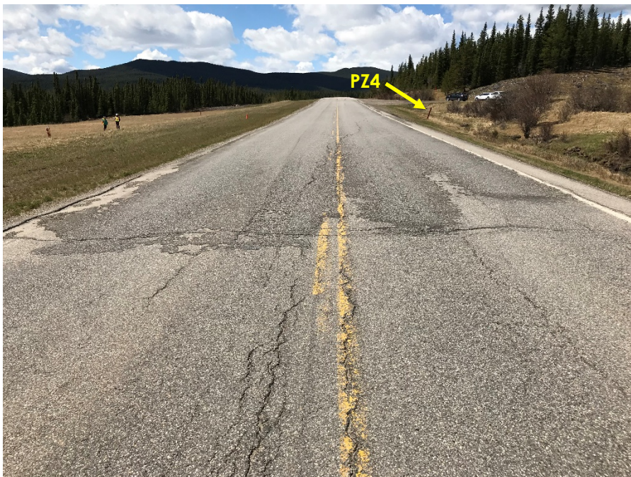
Photo 4: Pavement cracks at east end of patch. Looking west.
