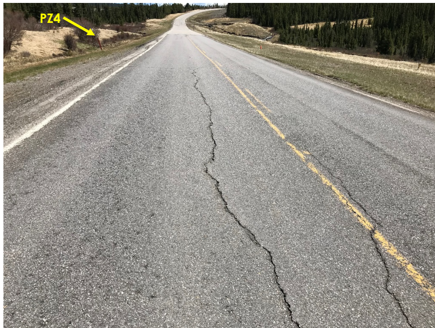
Photo 2: Pavement cracks reflecting through patch in front of access road. Looking east.
