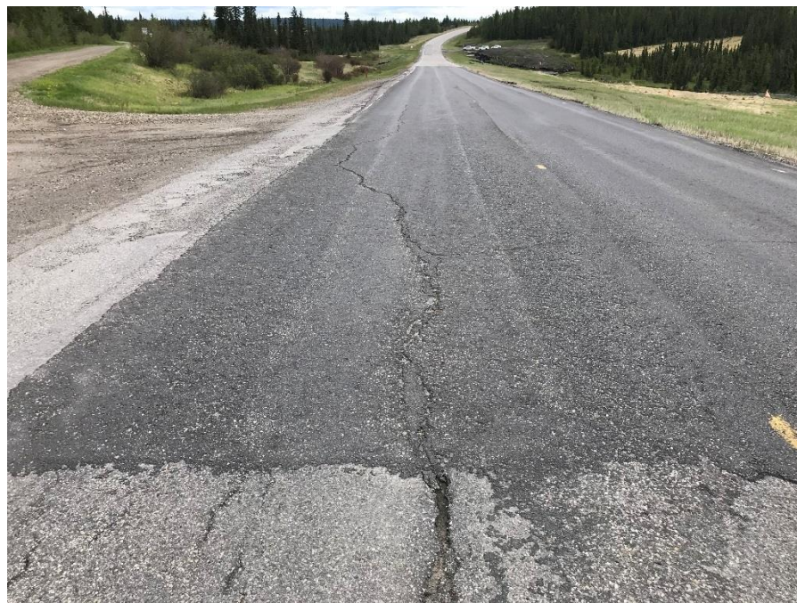
Photo 2: Pavement cracks reflecting through new patch in front of access road. Looking east.
