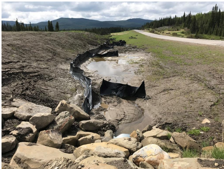
Photo 8: Erosion along drainage ditch east of culvert BF76754. Looking west.
