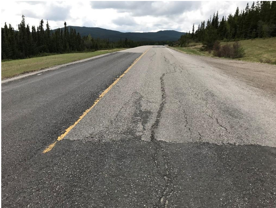
Photo 1: Pavement cracks reflecting through 2014 patch in front of access road. Looking west.
