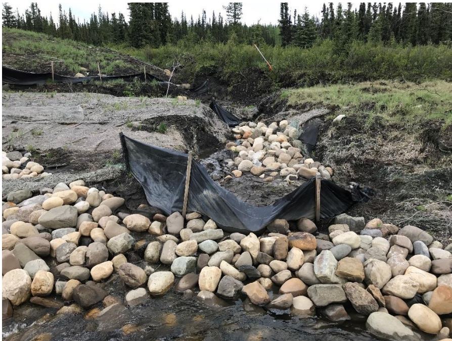
Photo 9: Rip rap to the south of BF76754 poorly placed. Erosion channel leading into culvert inlet.
