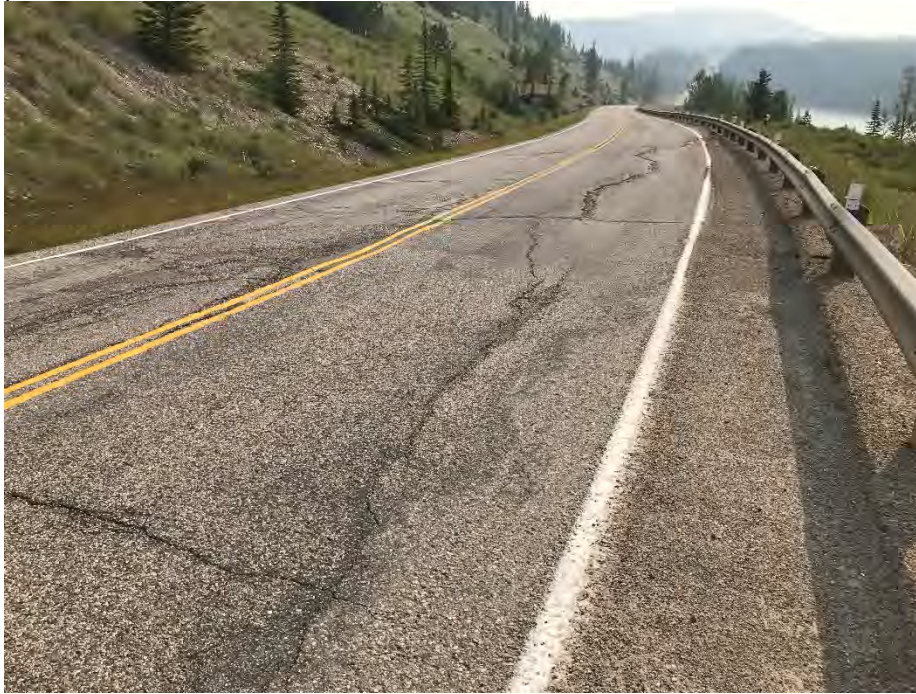
Photo 1: Pavement cracking at west extent. Looking east.
