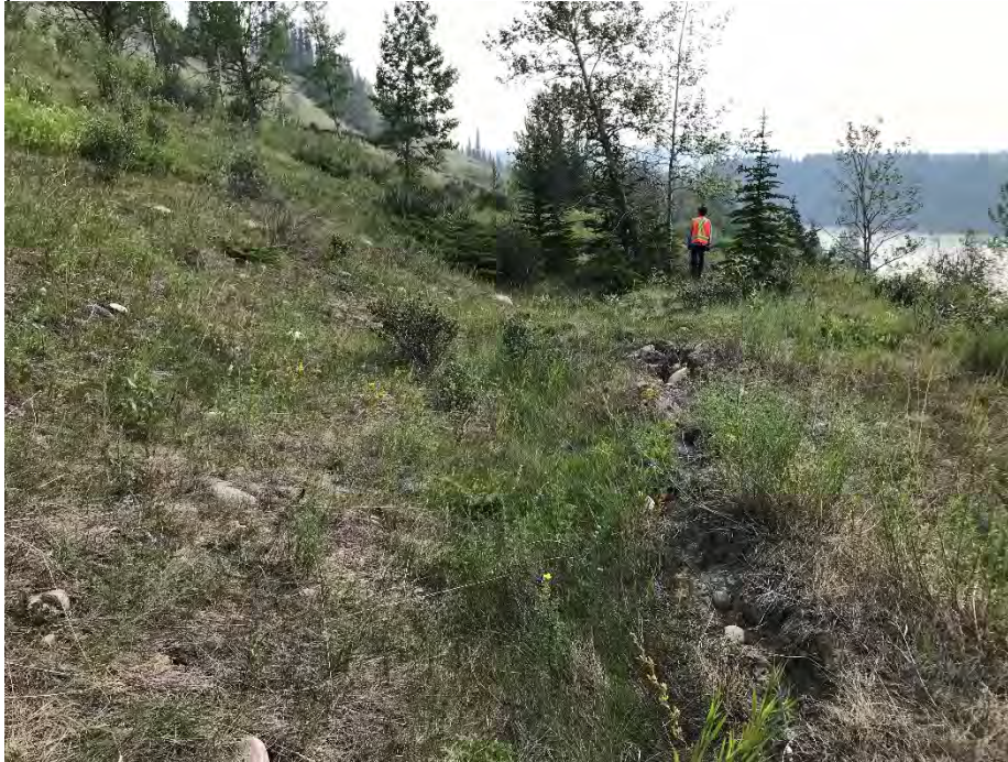
Photo 5: Ground crack at ridge location at the west extent of the west landslide. Leaning trees in background. Looking northeast.
