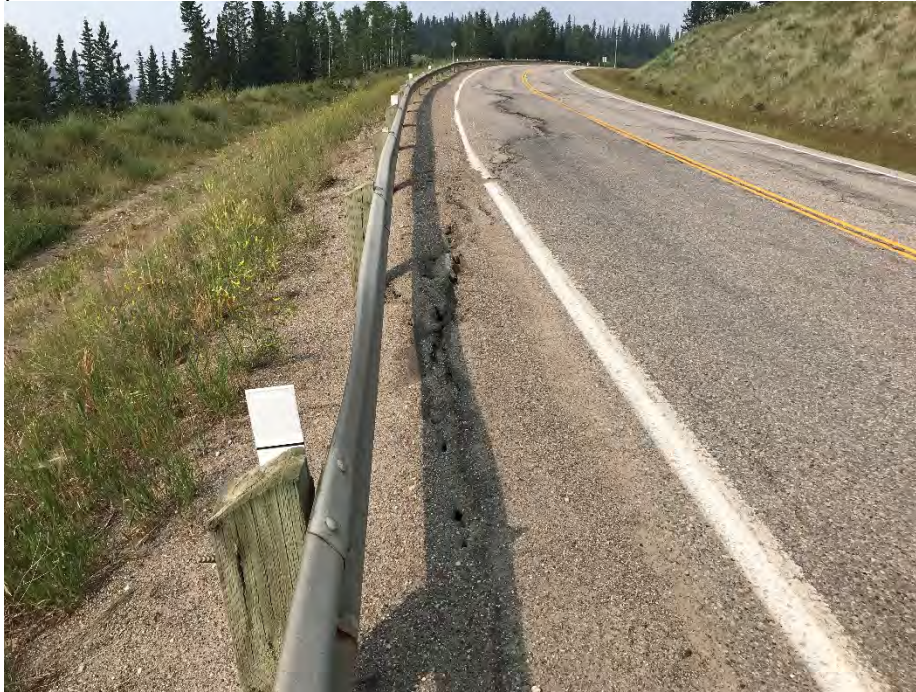
Photo 3: Pavement crack at east extent. Looking west.
