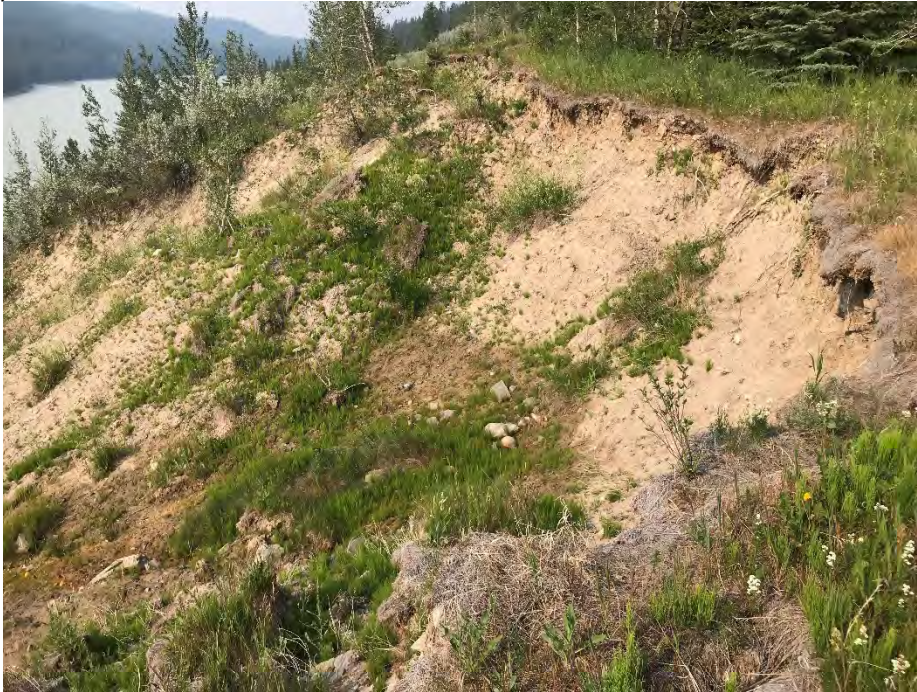
Photo 7: Seepage in east portion of east landslide. Looking west.
