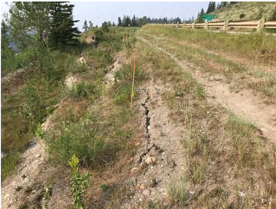
Photo 8: Tension crack behind south shoulder scarp. Distance to guardrail about 5.2 m. Looking southwest.
