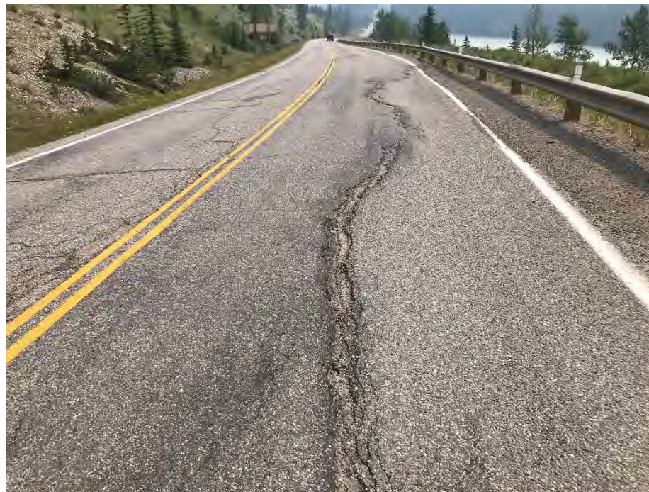
Photo 2: Pavement cracking approximately at midpoint. Looking east.
