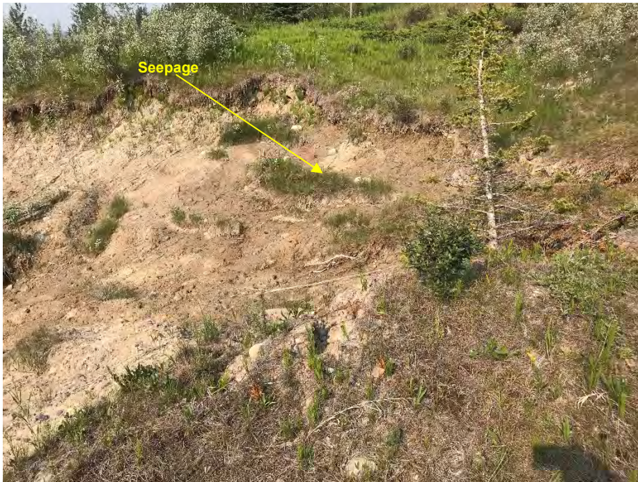
Photo 6: Seepage in west portion of east landslide. Looking northwest.
