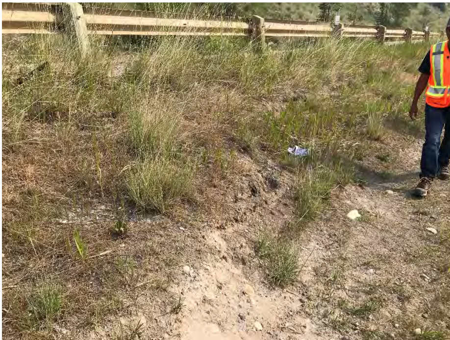
Photo 10: West extent of new scarp near “Hinton Entrance” sign. Looking northeast.
