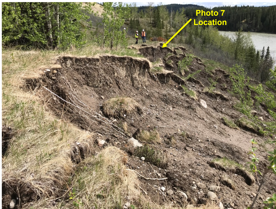
Photo 9: Series of retrogressive slides downslope from scarp near Highway 40. Looking east.
