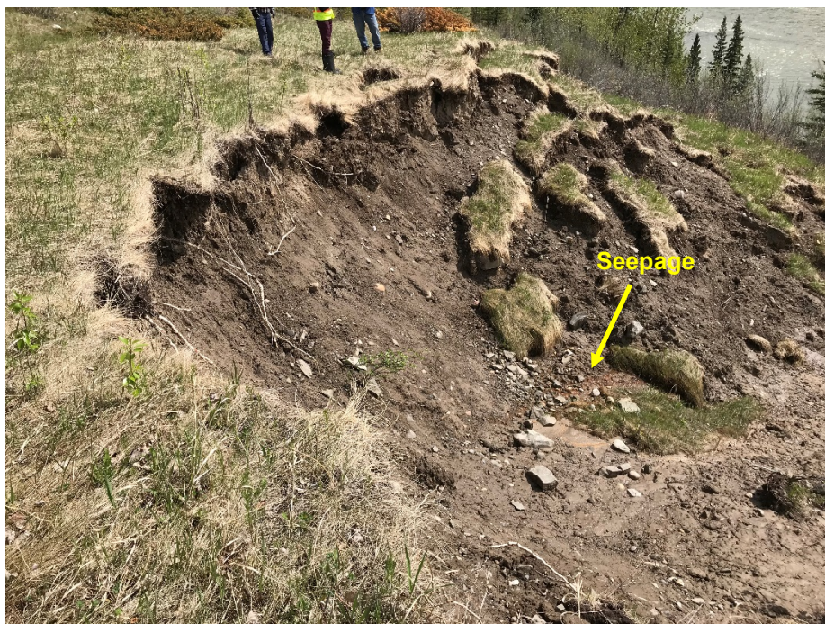
Photo 10: Seepage at base of scarp. Looking east.
