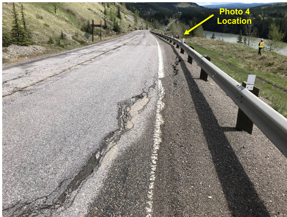
Photo 3: Pavement cracking. Looking northeast.
