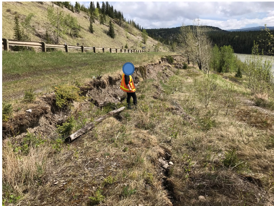
Photo 4: West end of scarp near highway. Looking northeast.
