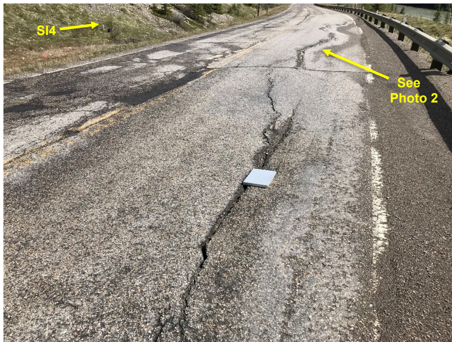
Photo 1: Pavement cracking. Looking northeast.
