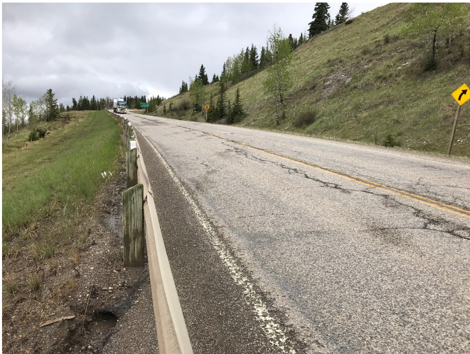
Photo 8: Highway 40 upslope from scarp. Looking west.
