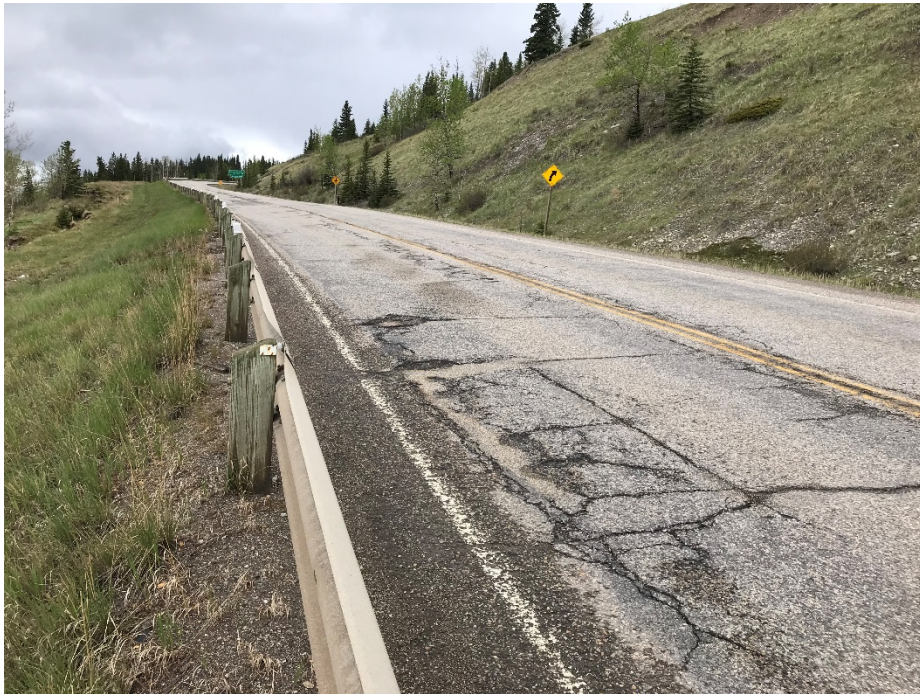
Photo 7: Highway 40 upslope from scarp. Looking west.
