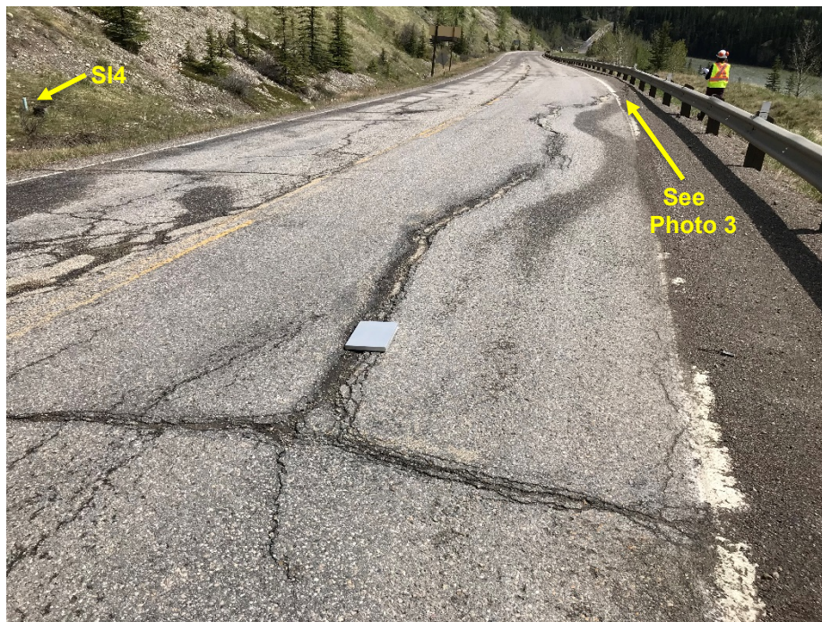
Photo 2: Pavement cracking. Looking northeast.
