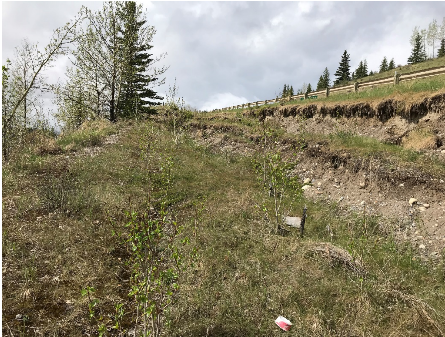
Photo 5: West end of scarp near highway. Looking southwest.
