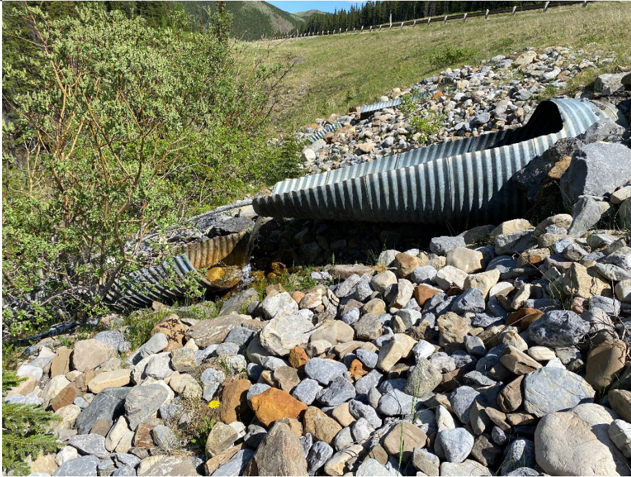
Photo 9: Water undermining culvert. Looking east.
