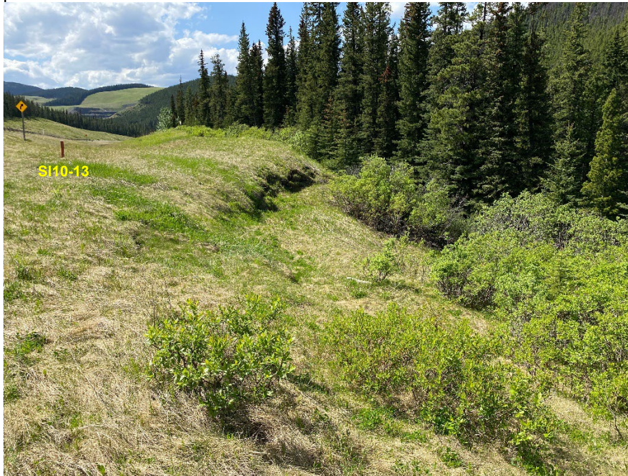
Photo 1: Retrogressive scarp on the north side of the pile wall, looking west.
