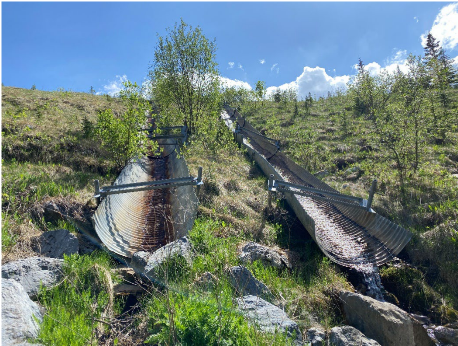
Photo 10: Twisted bracing along half-round culverts. Looking southwest.
