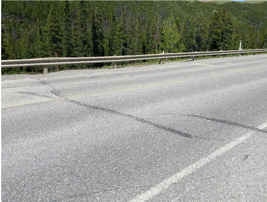
Photo 5: Pavement crack west of C/L culvert at pile wall site. Looking northeast.
