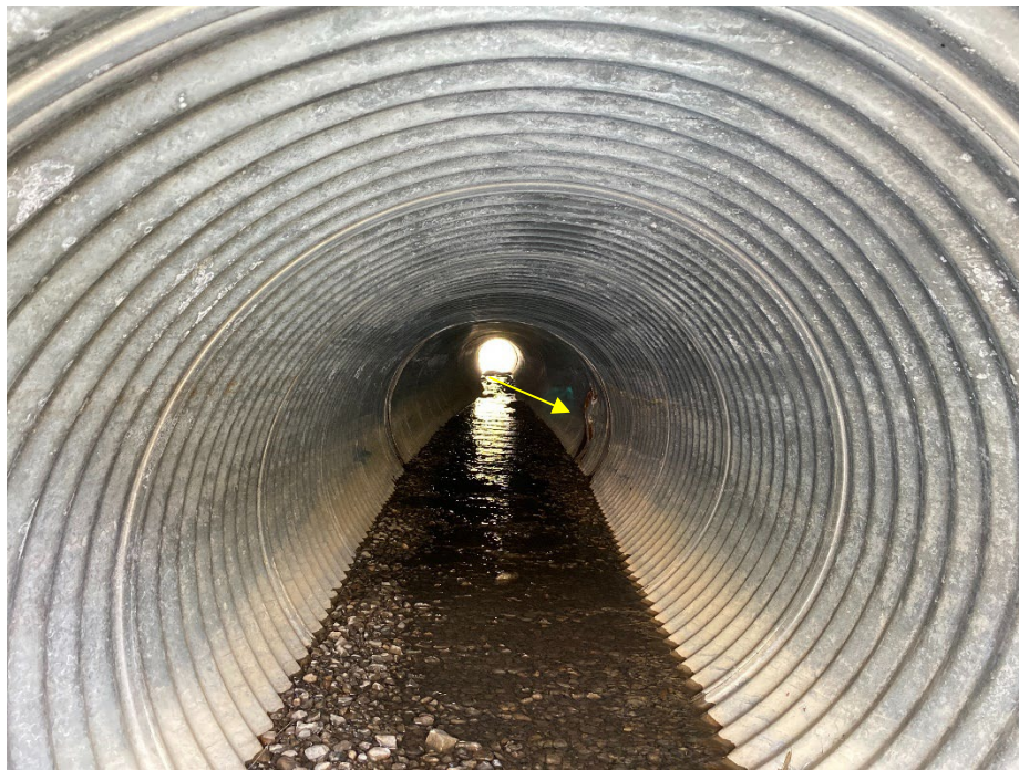
Photo 4: Bulge in west sidewall of C/L culvert. Looking south.
