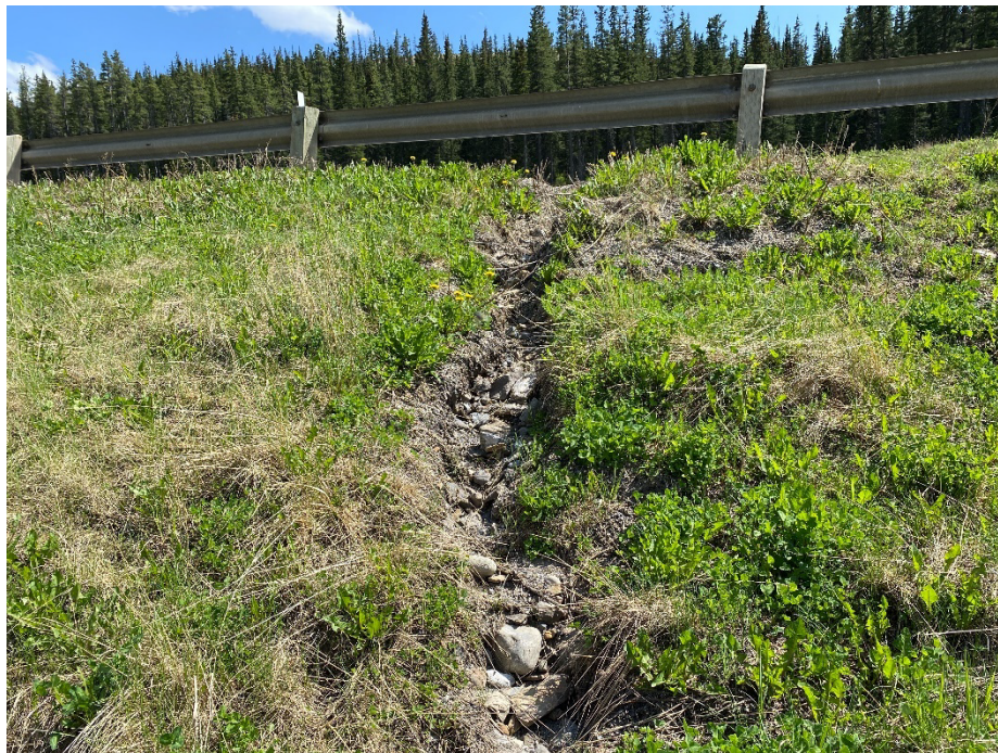
Photo 2: Gully on north side of the highway, to the west of the C/L culvert. Looking south.
