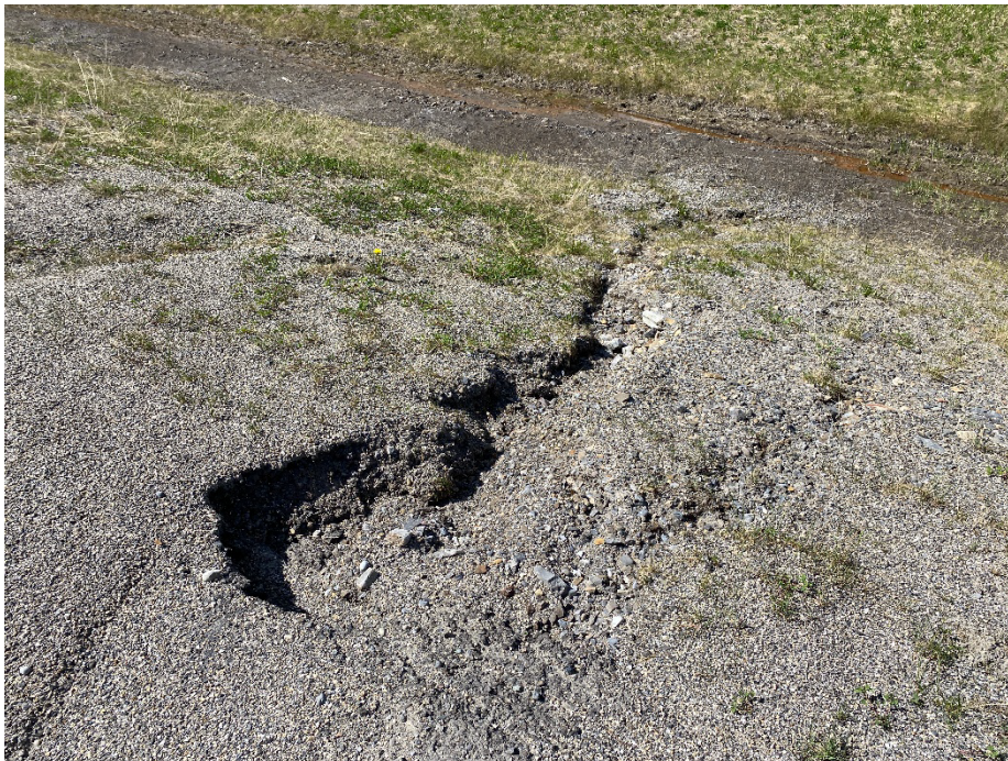
Photo 6: Seepage along north ditch between pile wall site and culvert site with erosion rills and gully on the north ditch highway shoulder. Looking northwest.
