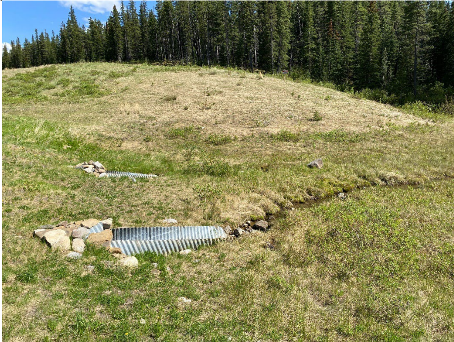
Photo 11: Culvert inlets on south side of highway at culvert site, looking southeast.
