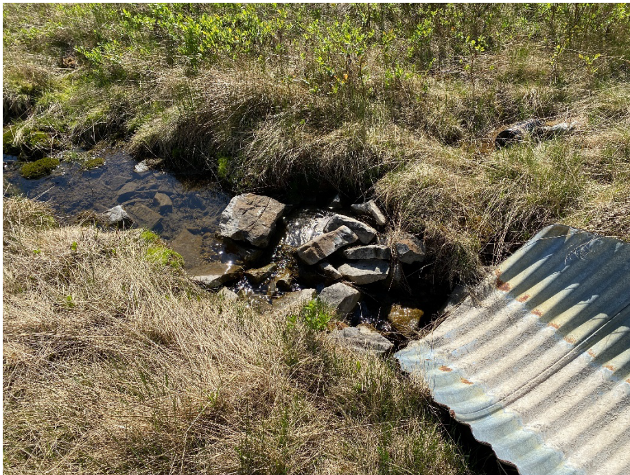
Photo 12: Water undermining the west culvert inlet at the culvert site. Looking west.
