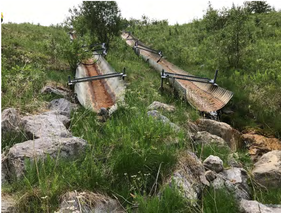
Photo 8: Twisted bracing along half-round culverts. Looking southwest.
