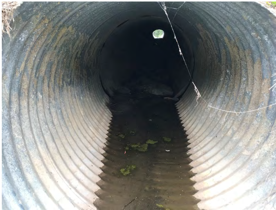
Photo 2: Separation between first and second segment of C/L culvert at inlet. Looking north.
