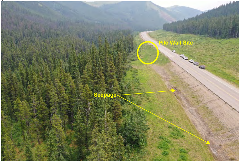
Photo 5: Seepage along north ditch between pile wall site and culvert site. Multiple erosion rills along shoulder visible. Taken with drone looking east.
