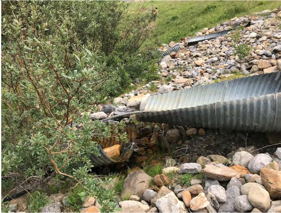
Photo 7: Water undermining culvert. Looking east.
