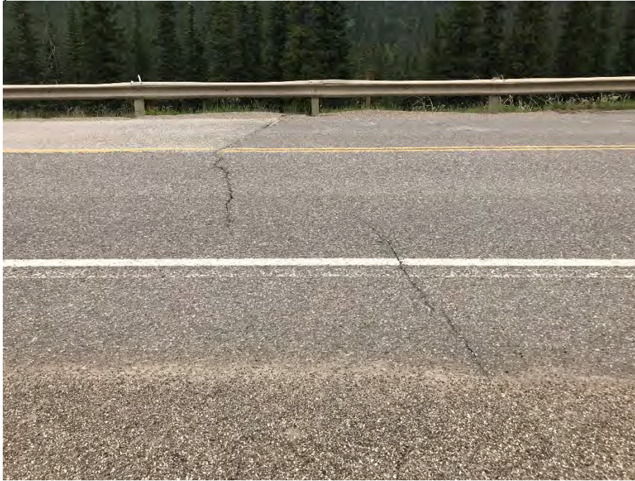
Photo 3: New pavement crack west of C/L culvert at pile wall site. Looking north.
