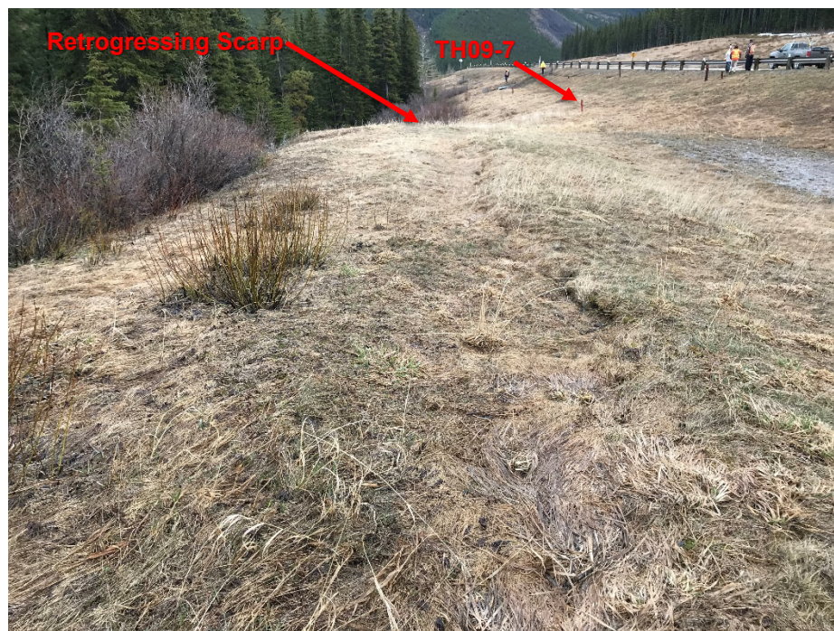
Photo 2: New ground cracks west of retrogressing scarp in Photo 3. Looking west.
