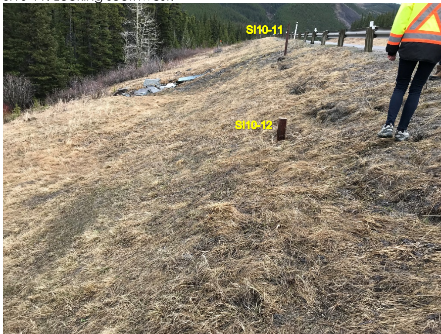
Photo 8: Ground cracking along approximate pile wall location. Looking east.
