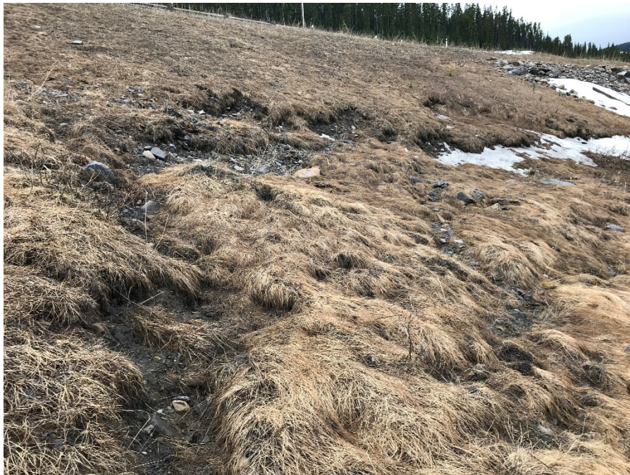
Photo 10: Highest scarp east of the half-round culverts. Looking west.
