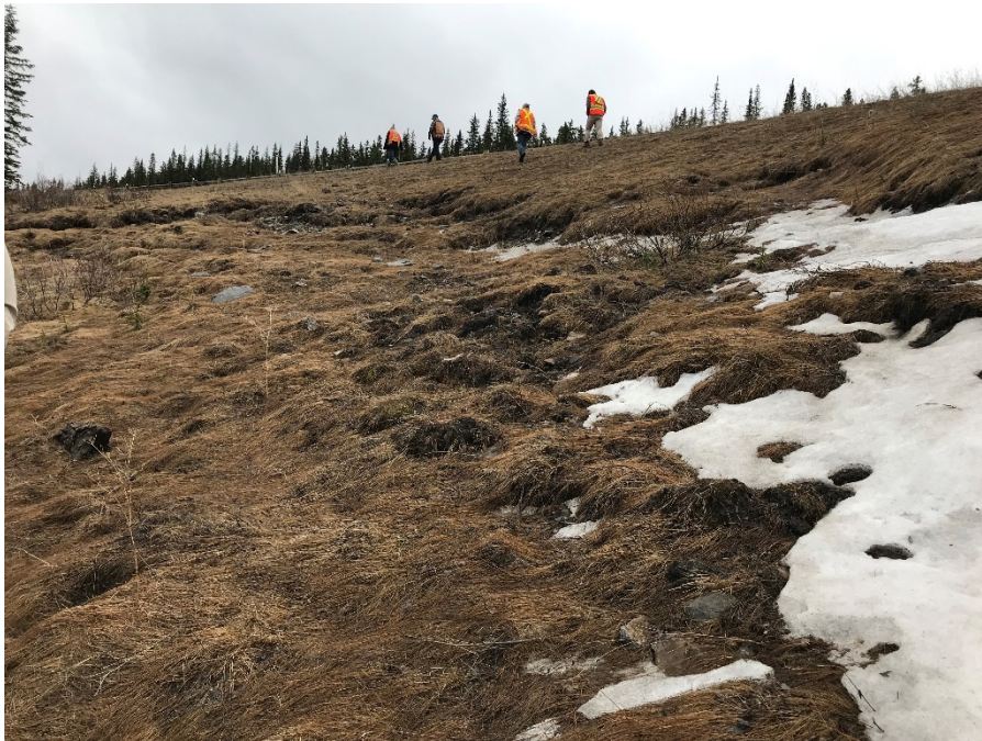
Photo 11: Highest scarp east of the broken culvert. Looking southeast.
