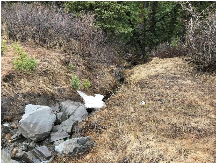
Photo 6: Erosion gully beyond the rip rap channel at the culvert outlet. Vegetation growing into gully. Looking north.
