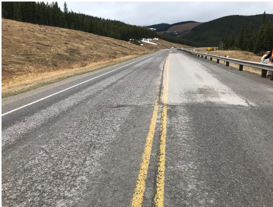
Photo 1: Previous asphalt patch south of pile wall appears unchanged. Cracking along pavement joints. Looking west.
