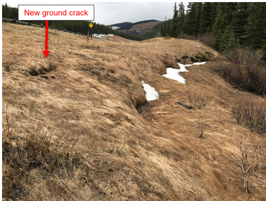
Photo 3: Retrogressive scarp from 2015 with vegetation growing in. New ground crack developing left of centre. Looking west.
