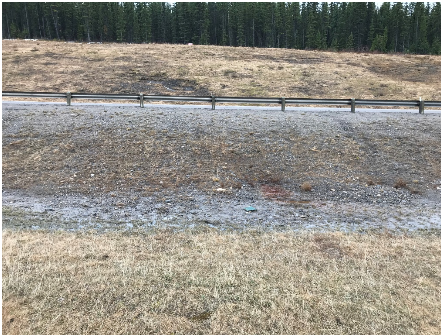
Photo 4: Soft saturated ground with minor erosion leading from culvert site to pile wall site. Orange seepage. Looking south.
