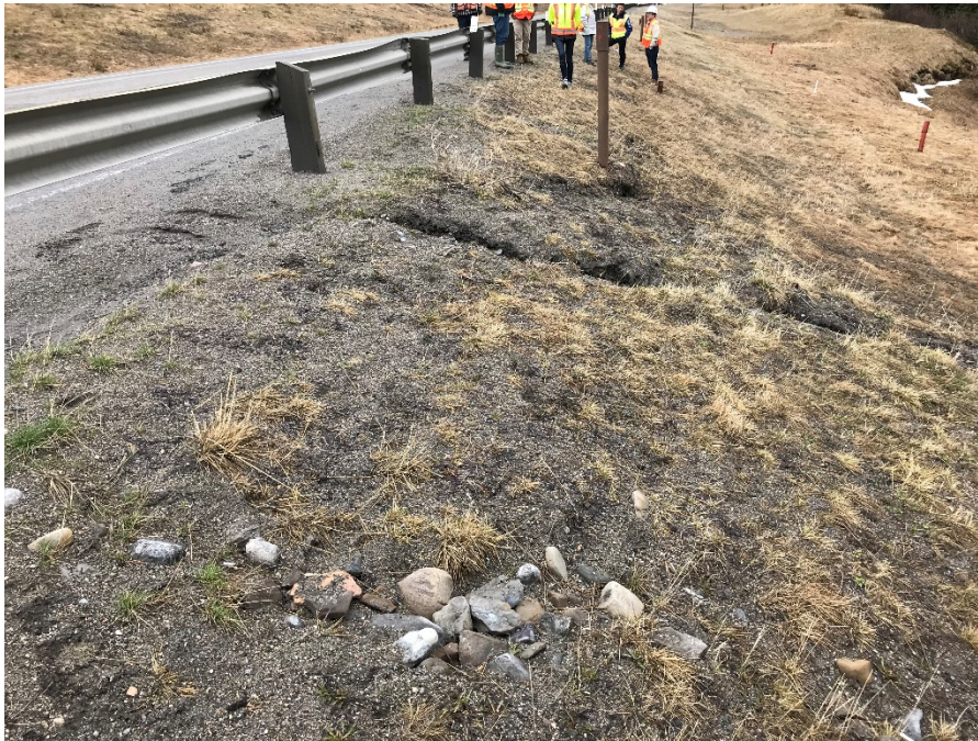
Photo 7: Erosion gully east of SI10-11. Slump/crack feature at base of SI10-11. Looking southwest.
