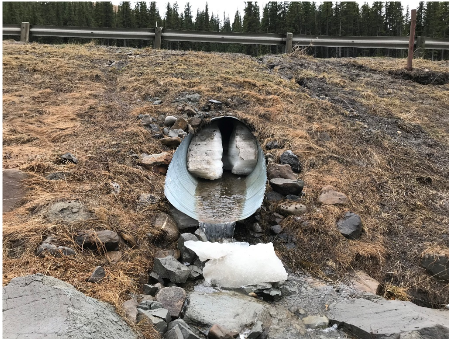
Photo 5: Culvert east of SI10-11 in flowing and in good condition. Ice in culvert. Slump at base of SI10-11 in top right about 300 mm high. Looking north.
