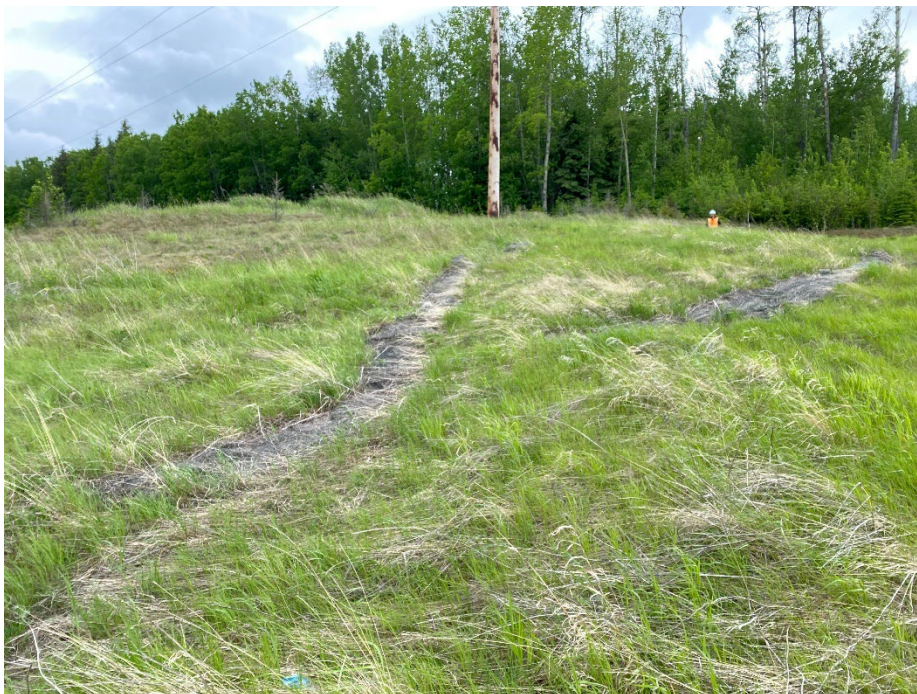
Photo 8: Repaired and vegetated south slope with bunched erosion control matting at approx. STA 34+950. Looking southeast.
