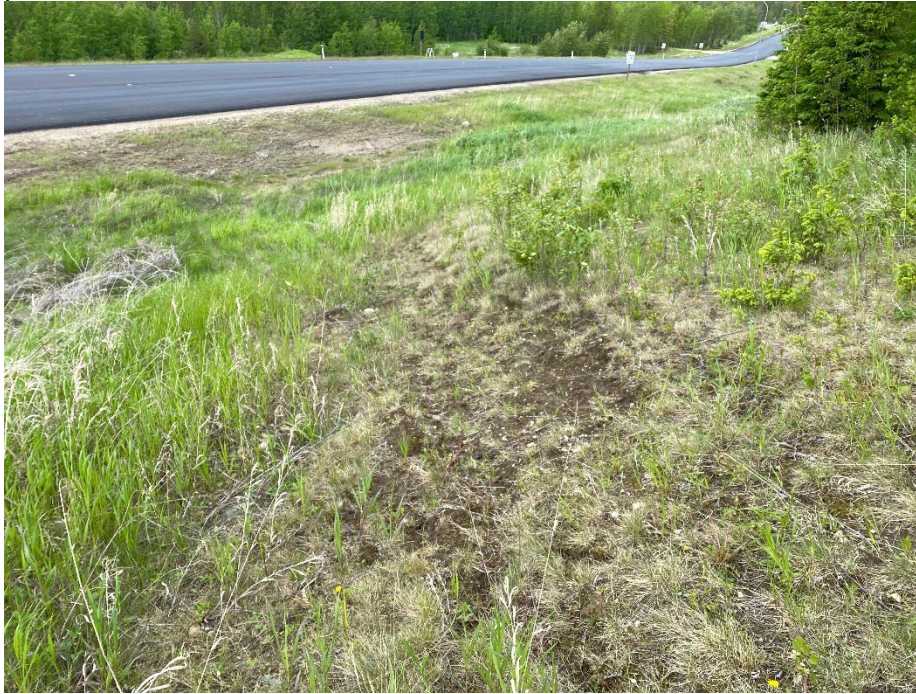
Photo 5: Old ground crack due to silt fence removal at approx. STA 34+960 not visible. Looking northeast.
