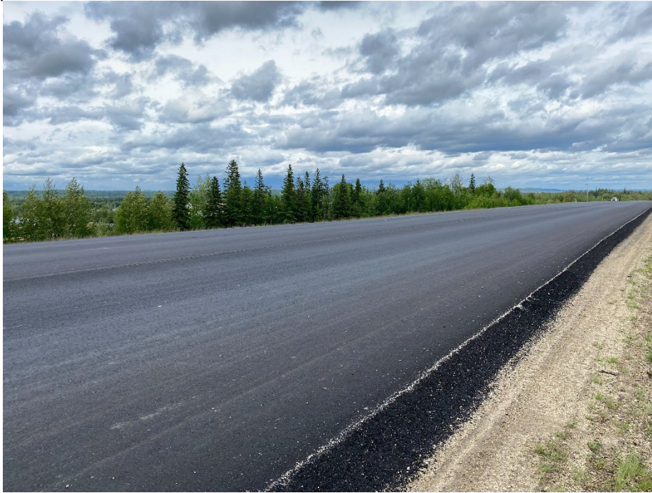
Photo 17: Pavement condition in WBL at approximately 34+575. Looking northeast.
