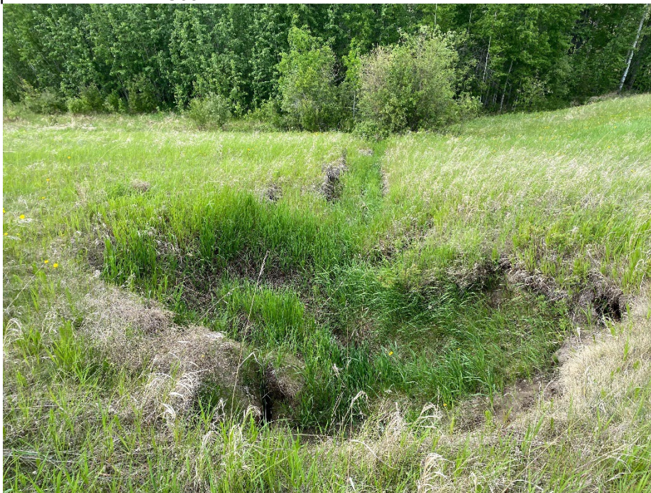
Photo 15: Sinkhole and gully directly upslope from the west culvert. Looking north.
