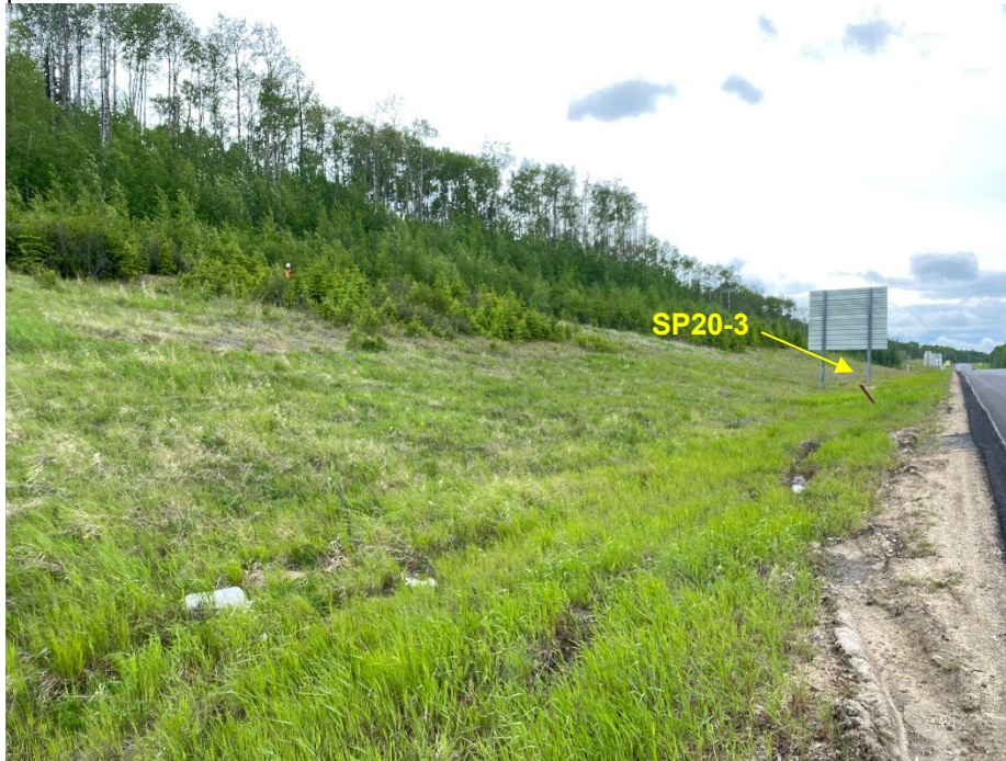
Photo 7: Erosion gully in the south ditch at approximately STA 34+880. SP20-3 casing leaning significantly. Looking west.
