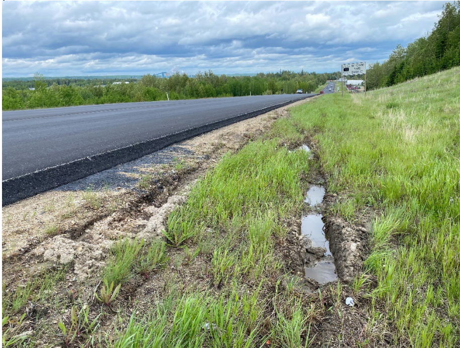
Photo 1: Tire tracks with ponded water in ditch near STA 34+950. Looking east.
