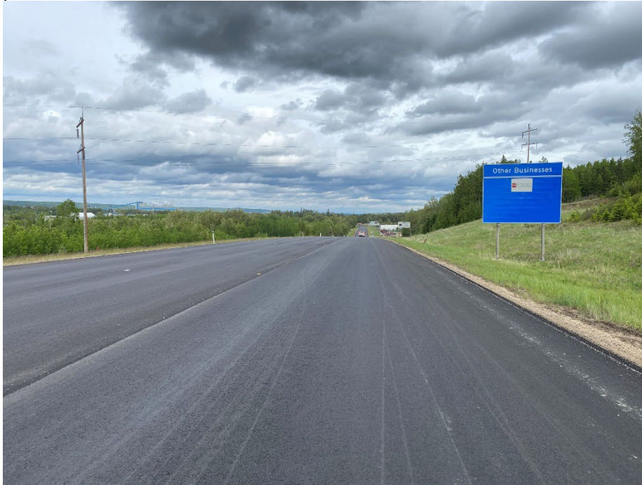
Photo 3: Pavement condition at approximately STA 34+850. Looking east.
