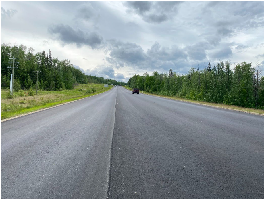
Photo 18: Pavement condition from approx. STA 34+450. Looking west.
