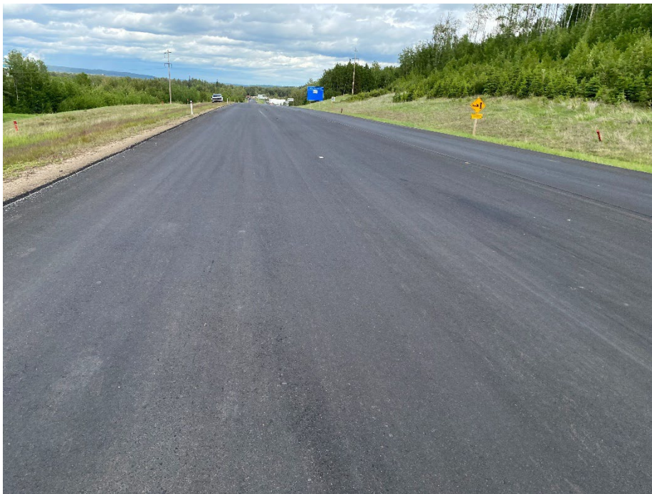
Photo 4: Pavement condition at approximately STA 34+775. Looking east.
