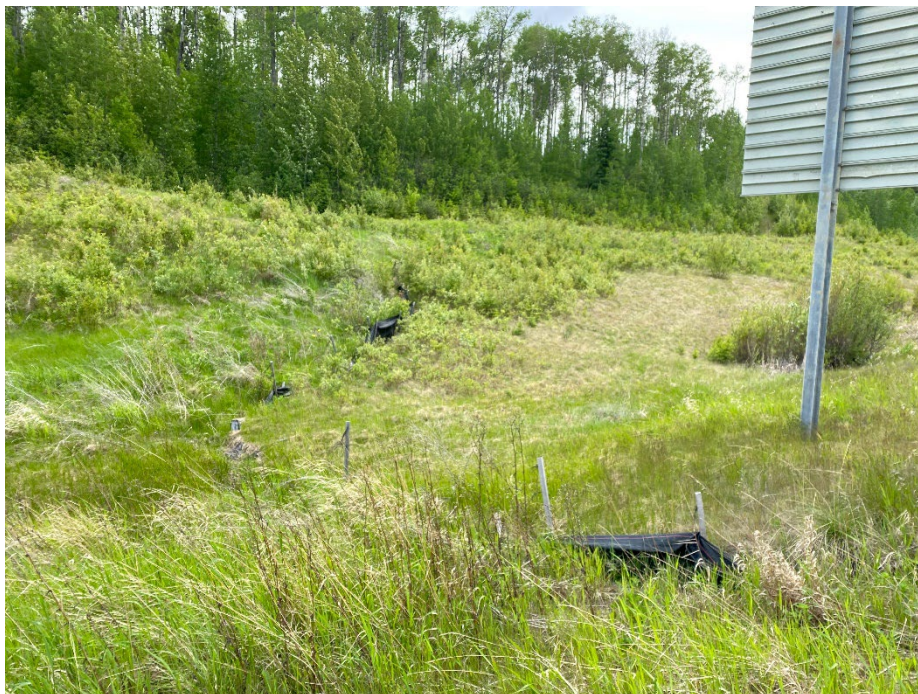
Photo 12: Silt fencing left on south slope at approx. STA 34+675. Looking south.
