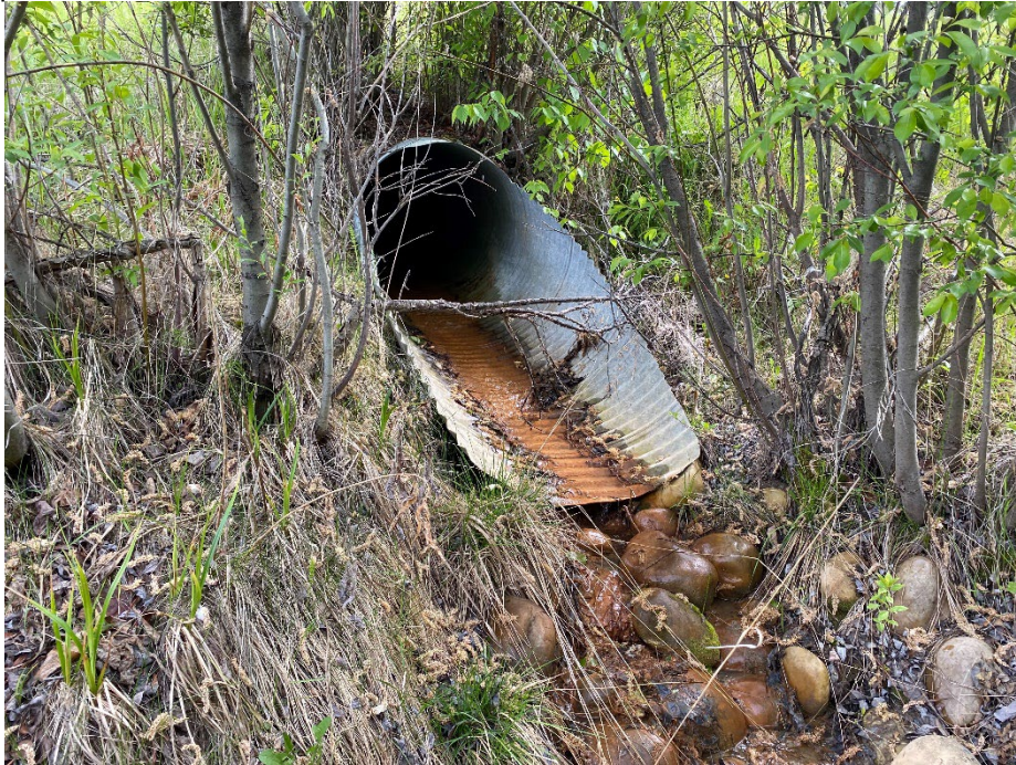
Photo 13: Culvert outlet adjacent to west extent of upper toe berm. Looking southwest.
