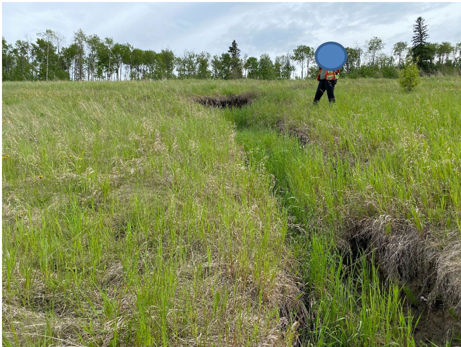
Photo 14: Gully and sinkhole directly upslope from west culvert. Looking south.
