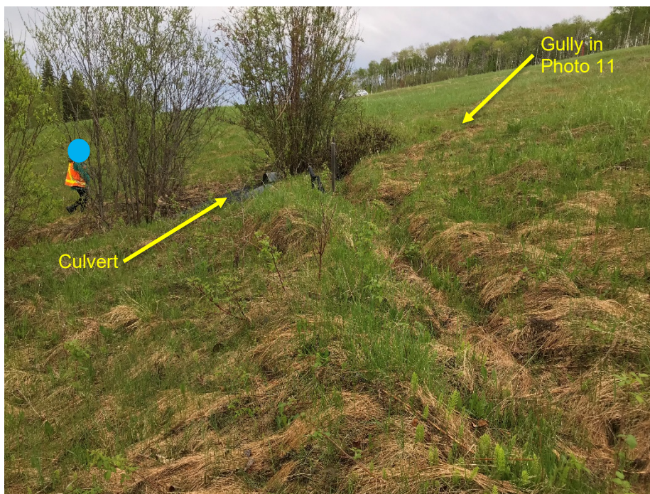
Photo 12: Small scarp west of culvert. Looking east.
