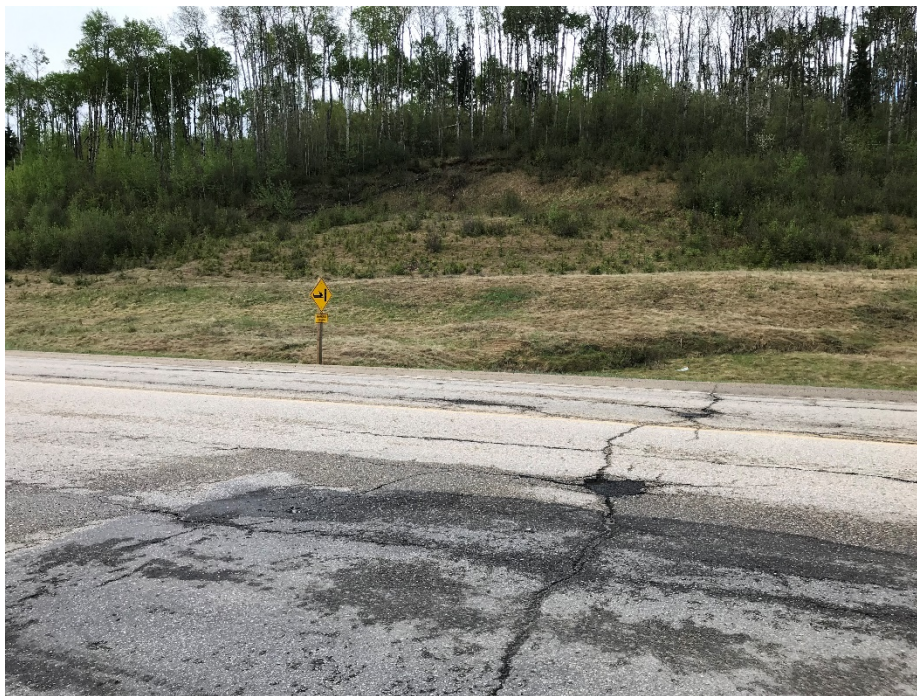
Photo 4: Scarp south of the highway at approximately Sta 34+700. Looking south.
