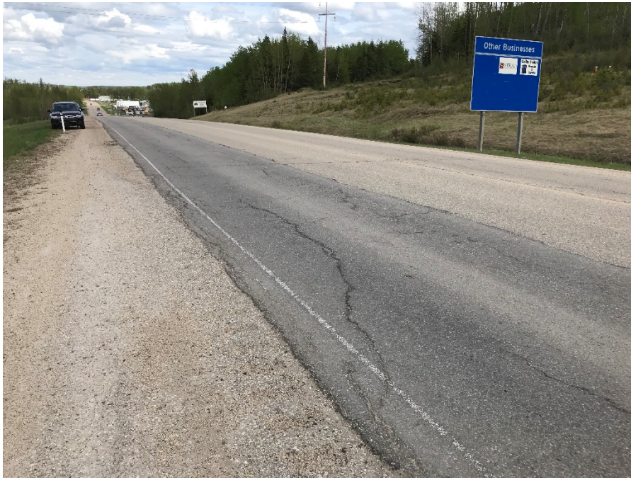
Photo 3: Pavement cracking at about Sta 34+850. Looking east.
