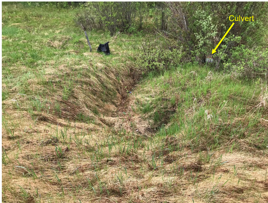
Photo 11: Vegetated gully immediately upslope of culvert in Photo 10. Looking north.
