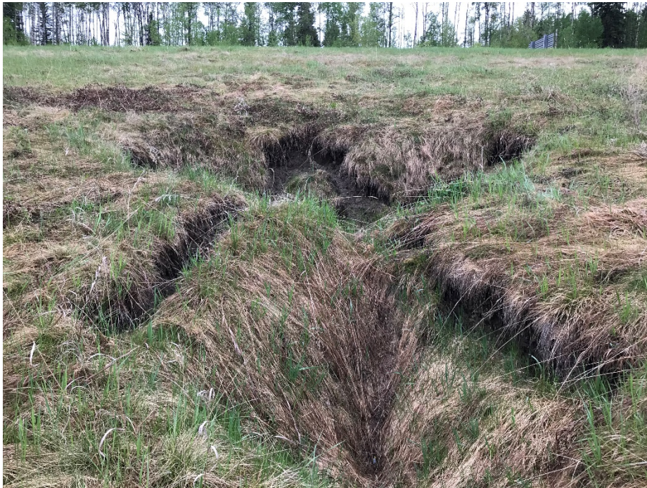
Photo 13: Slump/sinkhole along culvert alignment further upslope of culvert from Photos 10 and 11. Looking south.
