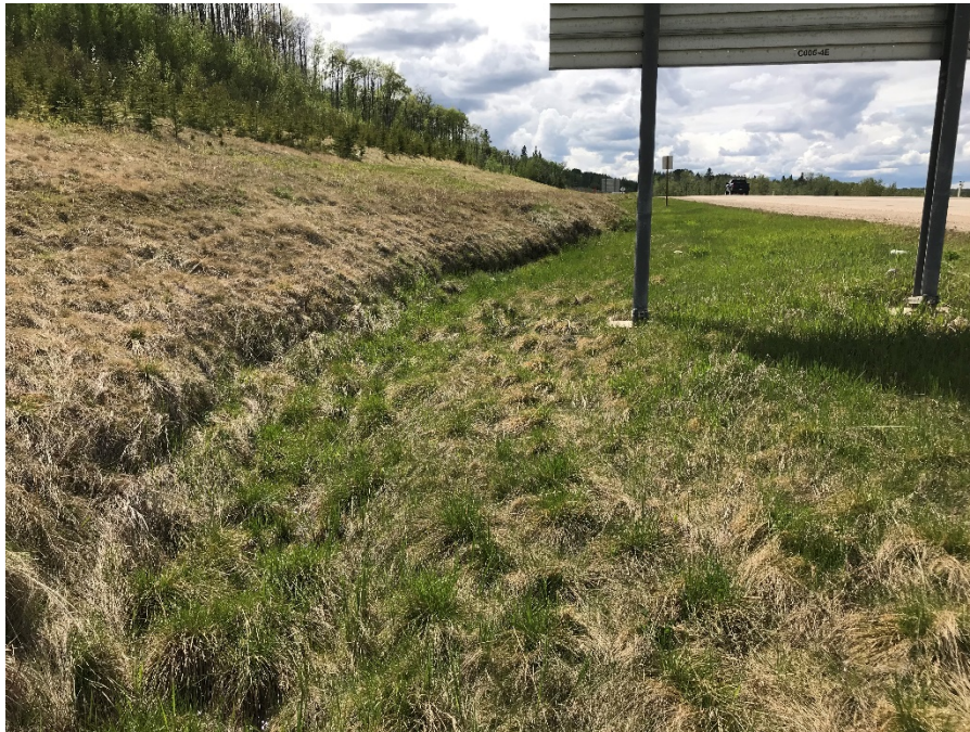
Photo 9: Toe bulging at "other businesses" sign. Looking east.
