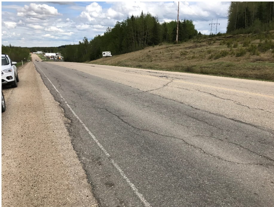
Photo 1: Circular crack observed in 2018 directly under powerline. Looking east.
