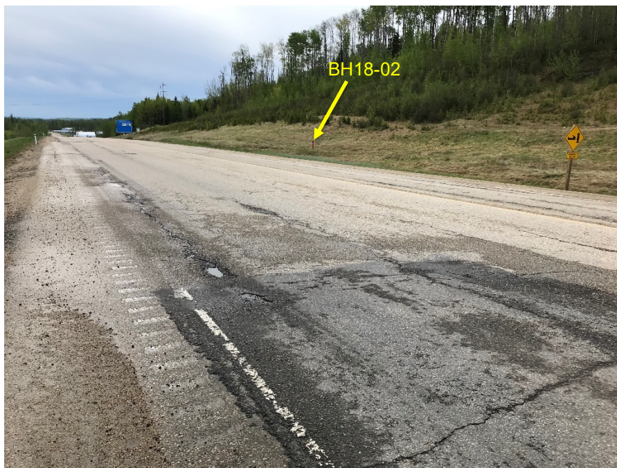
Photo 18: Pavement distress at about Sta 34+700. Looking east.
