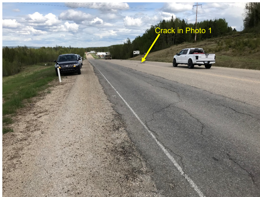
Photo 2: Pavement cracking at about Sta 34875 Looking east.
