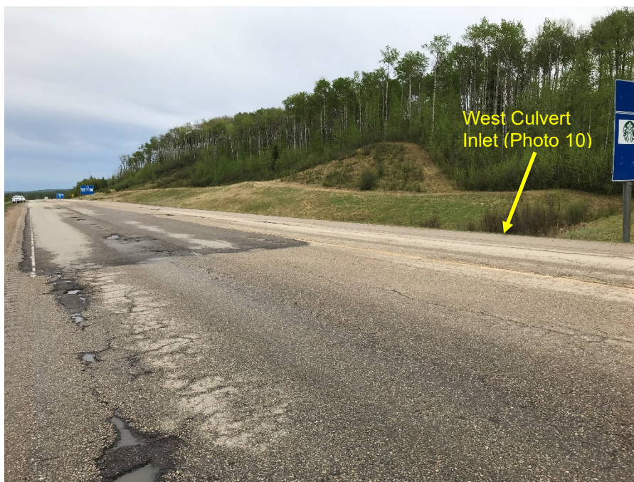
Photo 16: Pavement distress at west culvert alignment (approx. Sta 34+475). Looking west.
