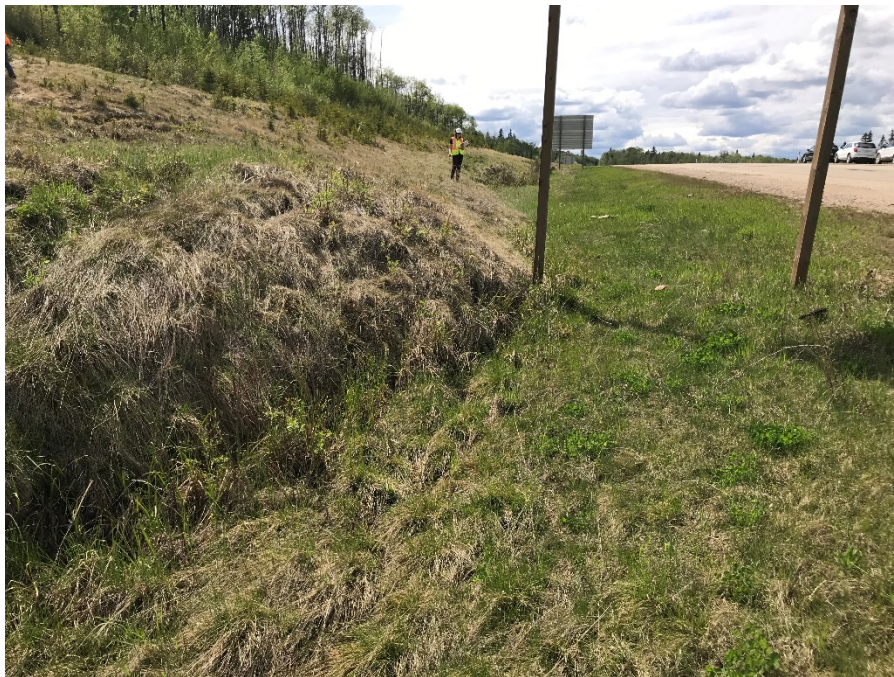
Photo 7: Toe bulge encroaching onto south ditch and signpost. Looking west.
