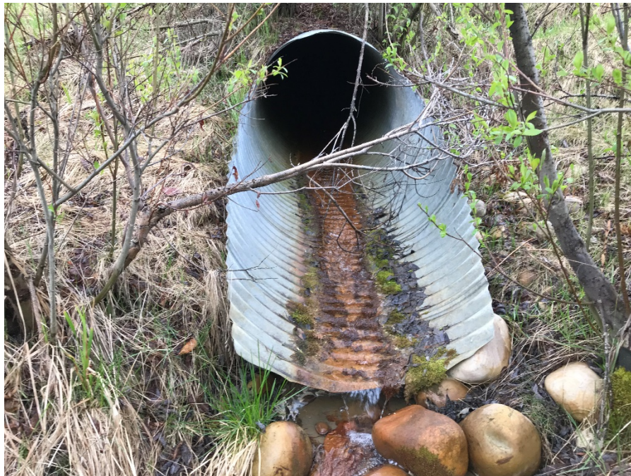
Photo 10: Culvert outlet adjacent to west extents of upper toe berm. Slumping immediately upslope of culvert. Looking south.
