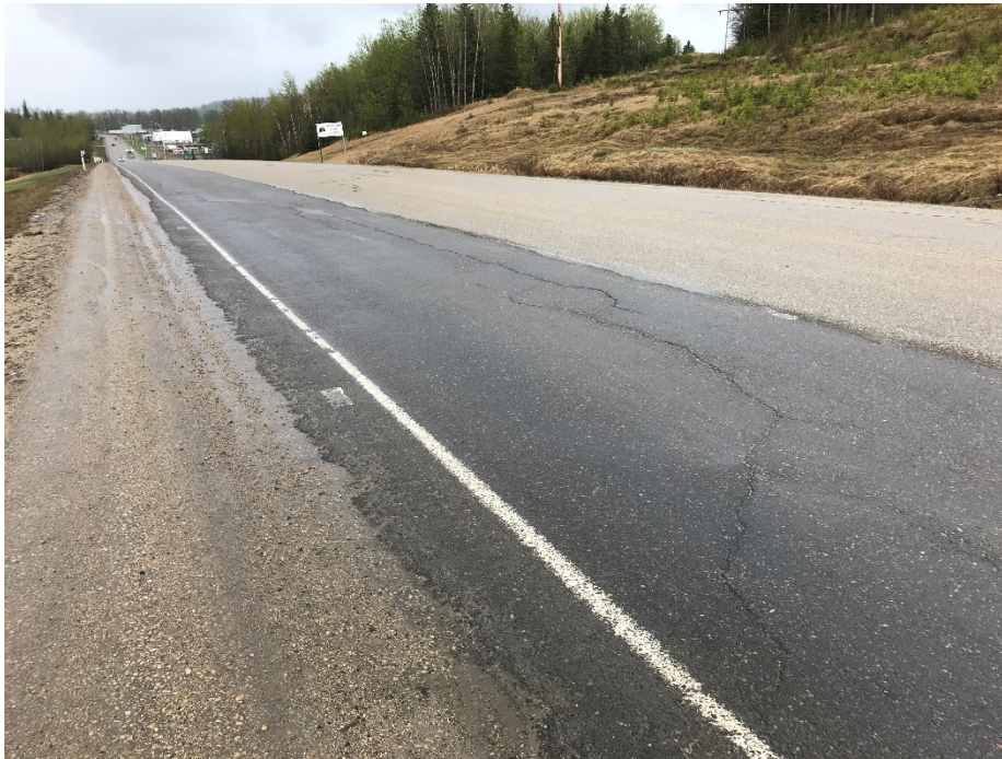
Photo 1: Circular cracks reflecting through 2018 patch. Cracks about 10 mm wide. Looking east.
