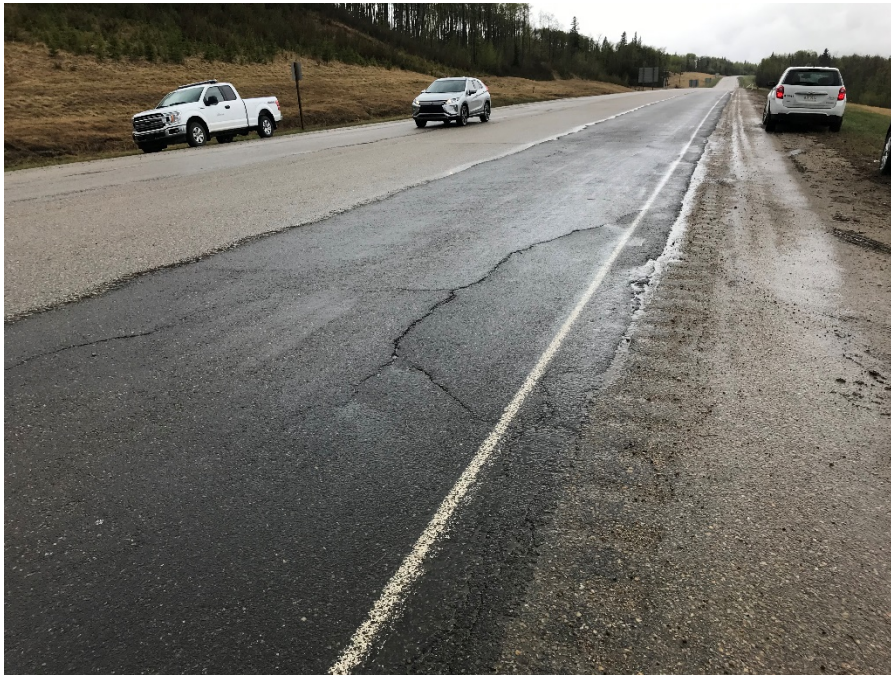
Photo 3: New circular crack up to 10 mm wide reflecting through 2018 patch. Looking west.
