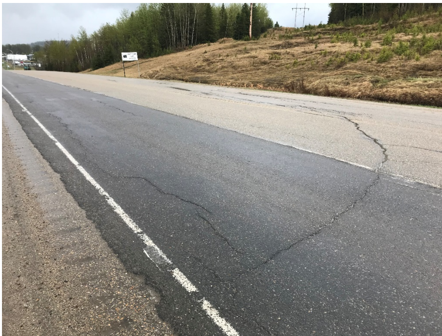
Photo 2: New circular crack up to 10 mm wide reflecting through 2018 patch at about Sta 34900. Looking southeast.
