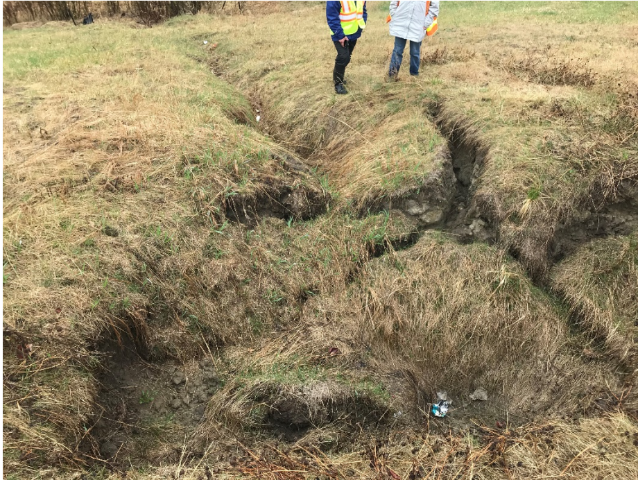
Photo 15: Erosion gully leading from sinkhole in Photo 14. Looking north.
