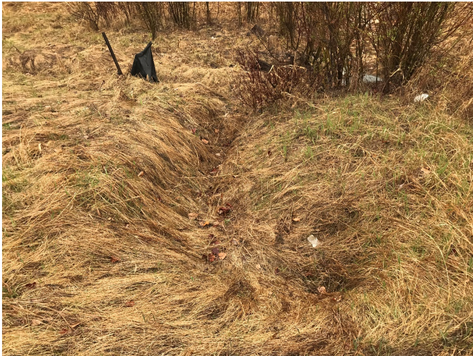
Photo 13: Vegetated gully immediately upslope of culvert in Photo 12. Looking north.
