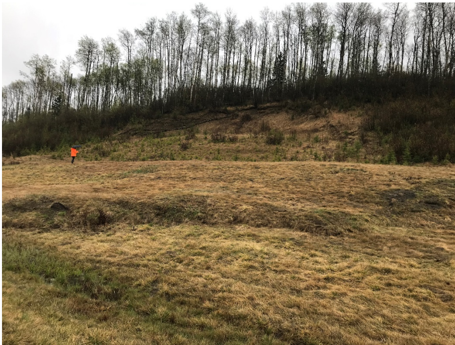
Photo 4: Scarp south of the highway at approximately Sta 34+700. Increased toe bulging. Looking south.
