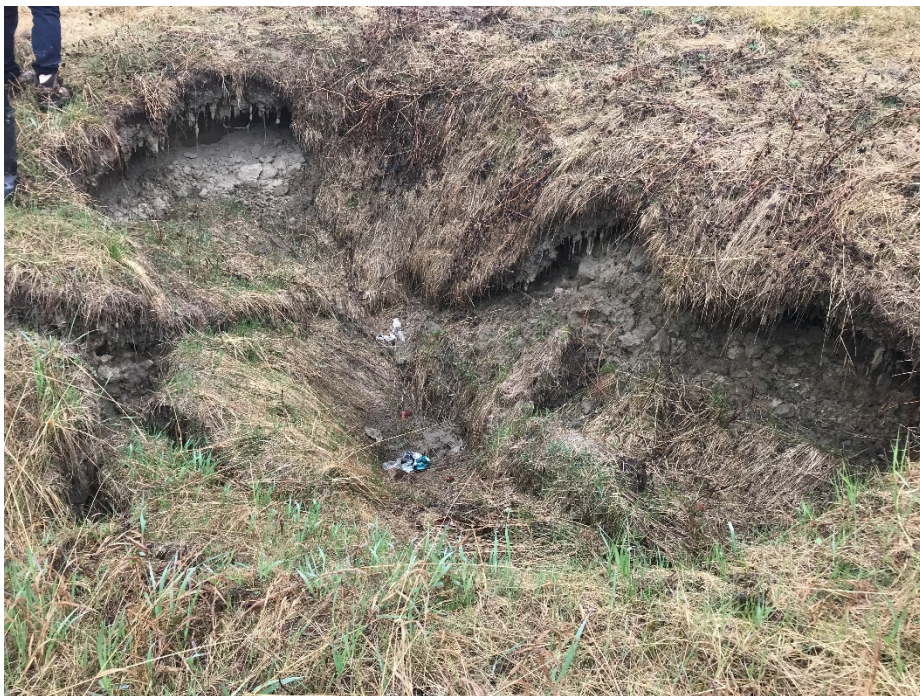
Photo 14: Slump/sinkhole along culvert alignment further upslope of culvert in Photo 12 and 13. Approximately 6 m wide by 2 m deep. Looking south.
