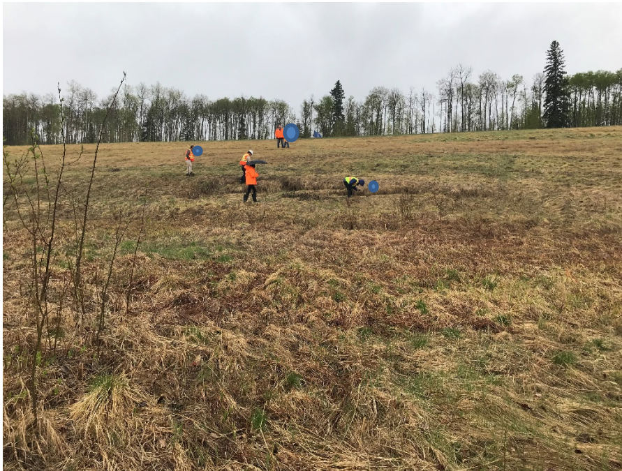
Photo 17: Tension crack/slump about 40 m west of Photo 12. Scarp about 1 m high. Looking south.
