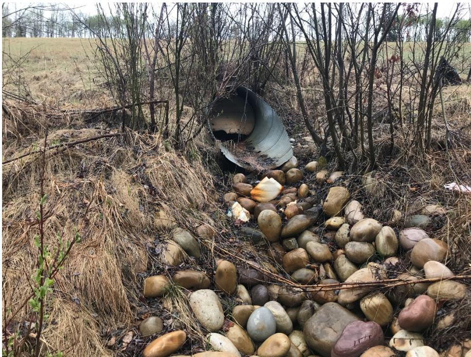
Photo 12: Culvert outlet adjacent to west extents of upper toe berm. Slumping immediately upslope of culvert. Looking south.
