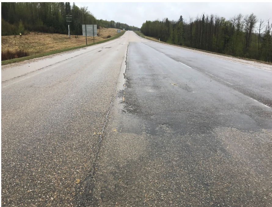
Photo 18: New patch on westbound lane at main slide site near S110-6. No cracks observed. Looking west.
