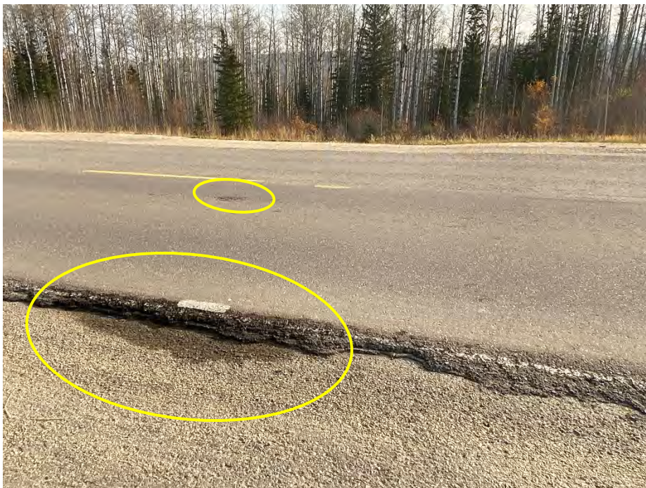
Photo 10: Wet spots on pavement, looking east.
