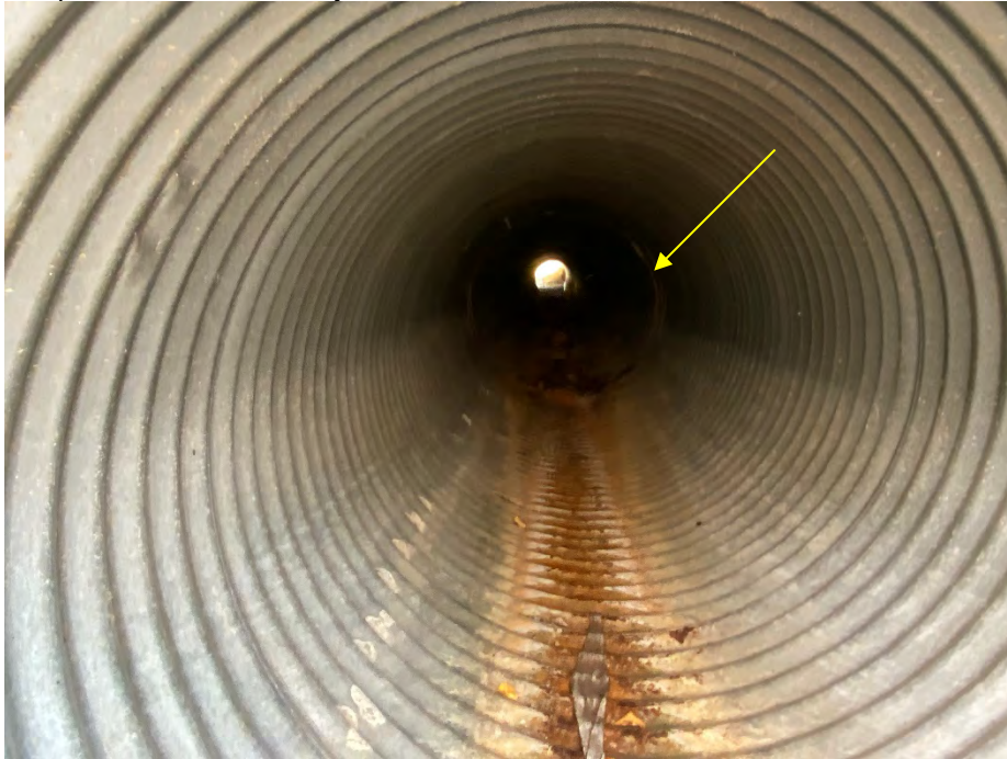
Photo 9: Possible separation between first and second segments of culvert inlet, looking east.
