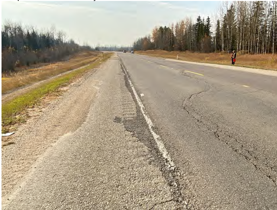
Photo 5: Cracking at the north flank of landslide. Pavement dipping to the east. Looking south.
