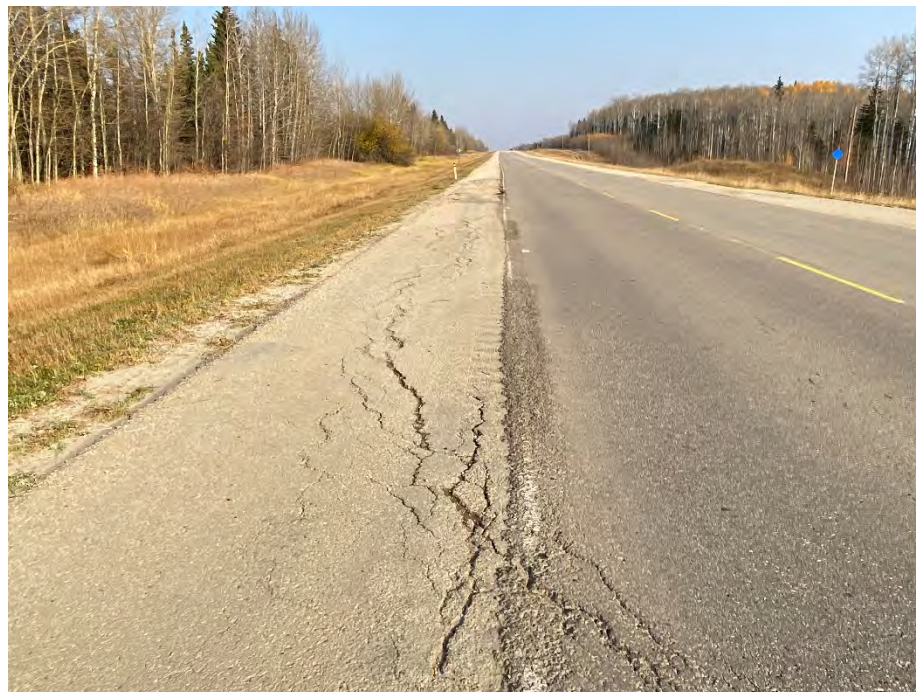
Photo 2: Wider cracks developing on shoulder of SBL. Looking northeast
