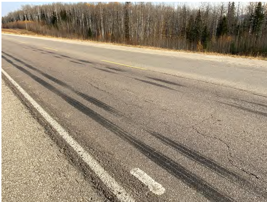
Photo 6: Tire marks and rutting in SBL. Looking northeast.
