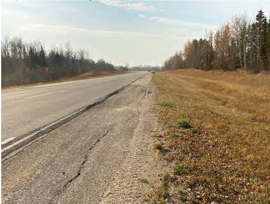
Photo 3: Cracking of SBL, looking southwest. Crack in left corner is approx. 125 mm deep.
