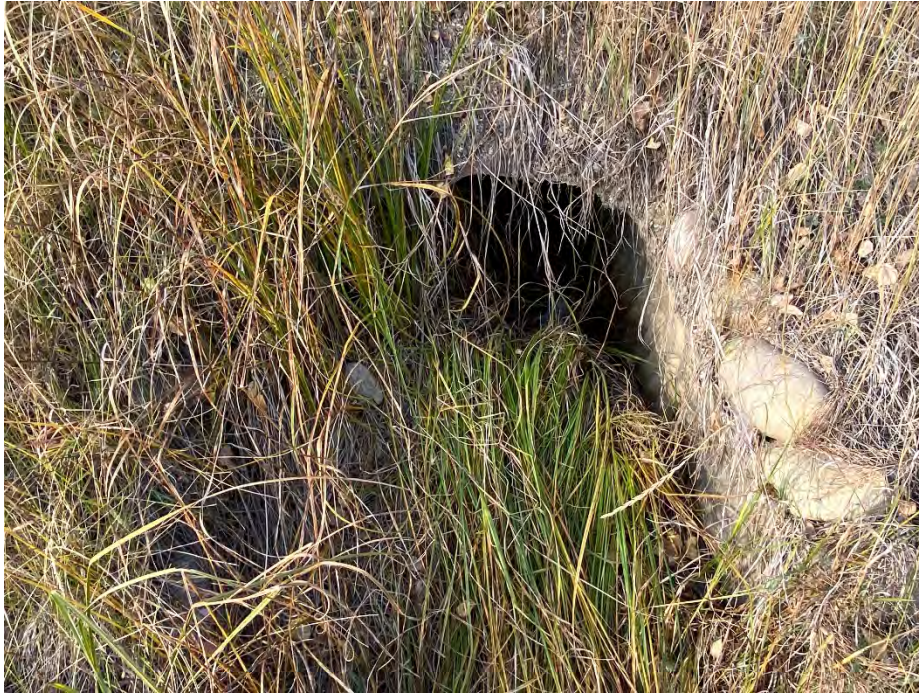
Photo 7: Culvert outlet becoming grown-in. Looking west.
