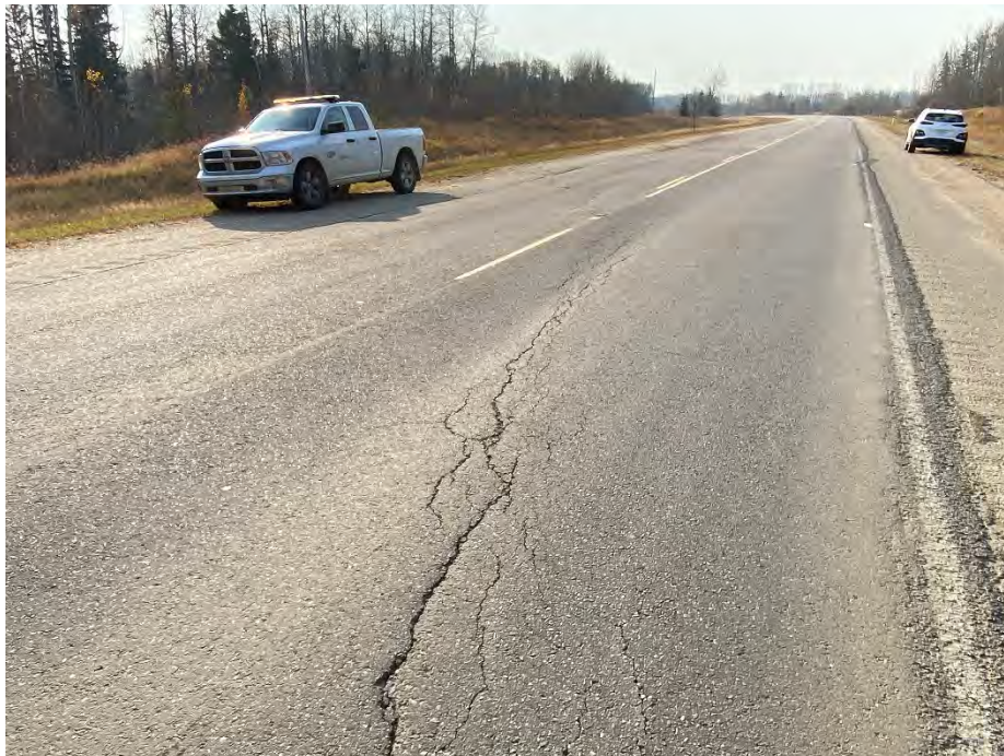
Photo 4: Crack at south flank of landslide. Pavement dipping to the east. Looking southwest.
