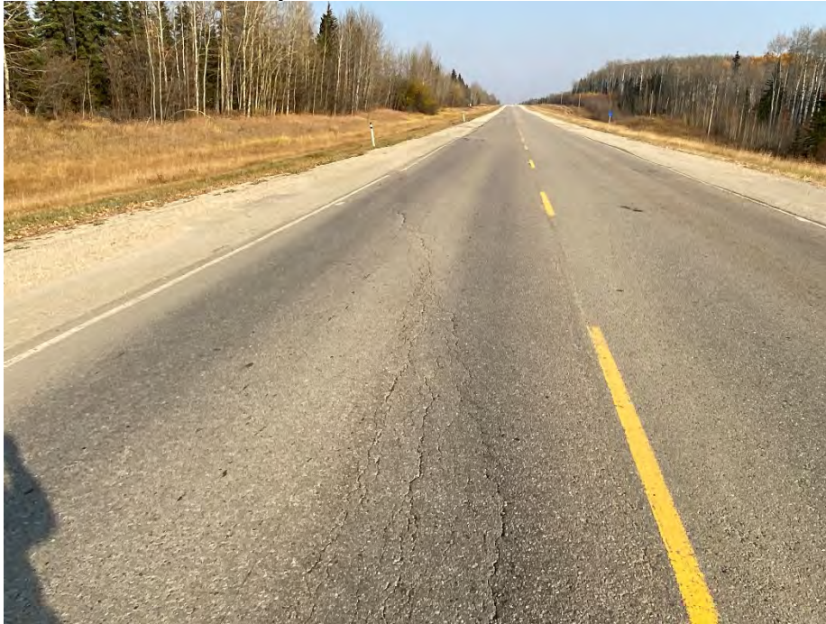
Photo 1: South extent of pavement cracking on Highway 32. Looking northeast.
