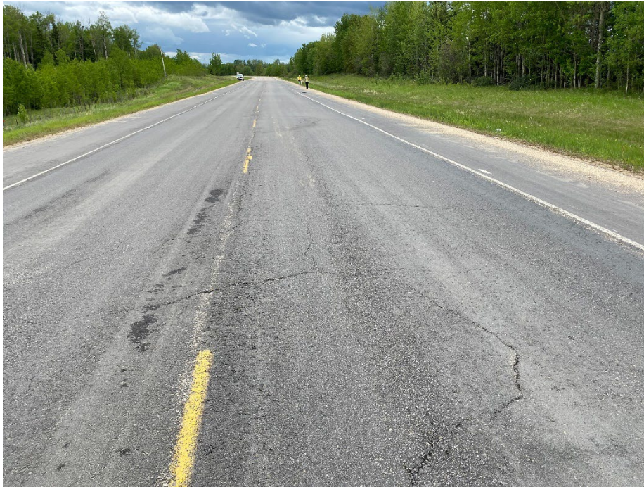
Photo 5: Cracking at the north flank of landslide. Looking south.
