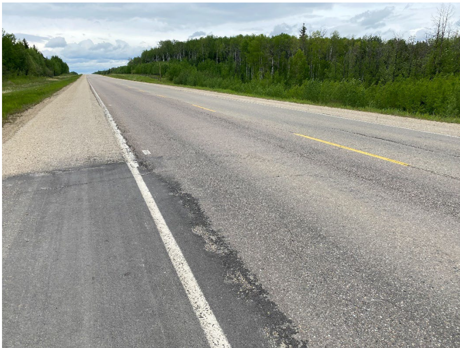
Photo 6: Rutting in SBL north from the pavement patch. Looking northeast.
