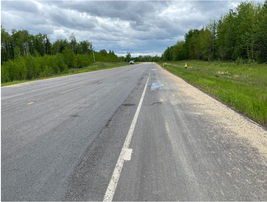
Photo 3: Condition of SBL, looking southwest. Wide cracking repaired.
