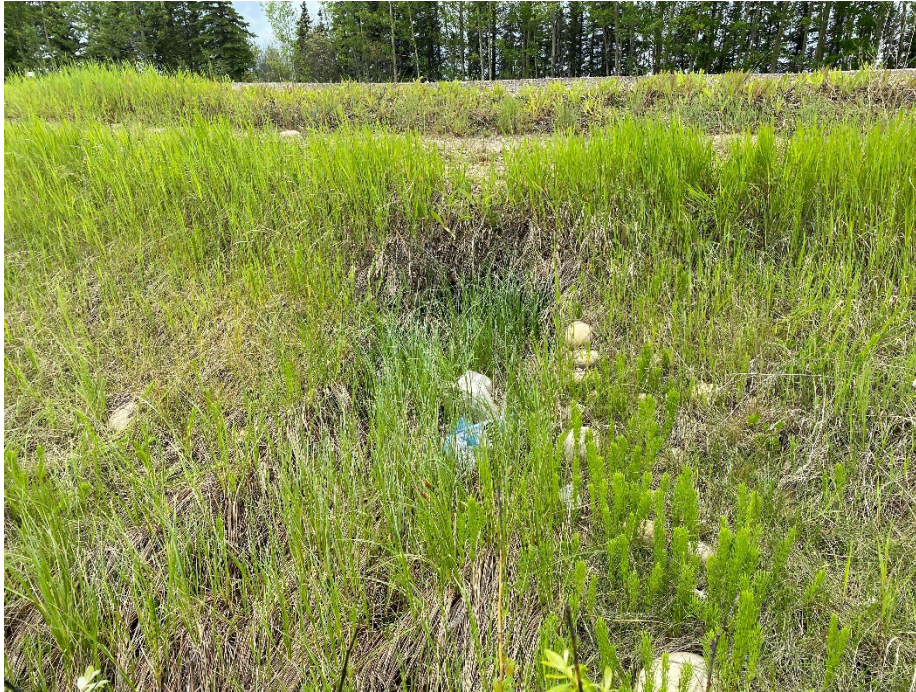
Photo 7: Culvert outlet becoming grown-in. Looking west.
