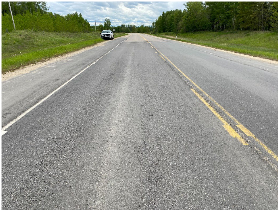
Photo 4: Thin cracks at south flank of landslide. Looking southwest.
