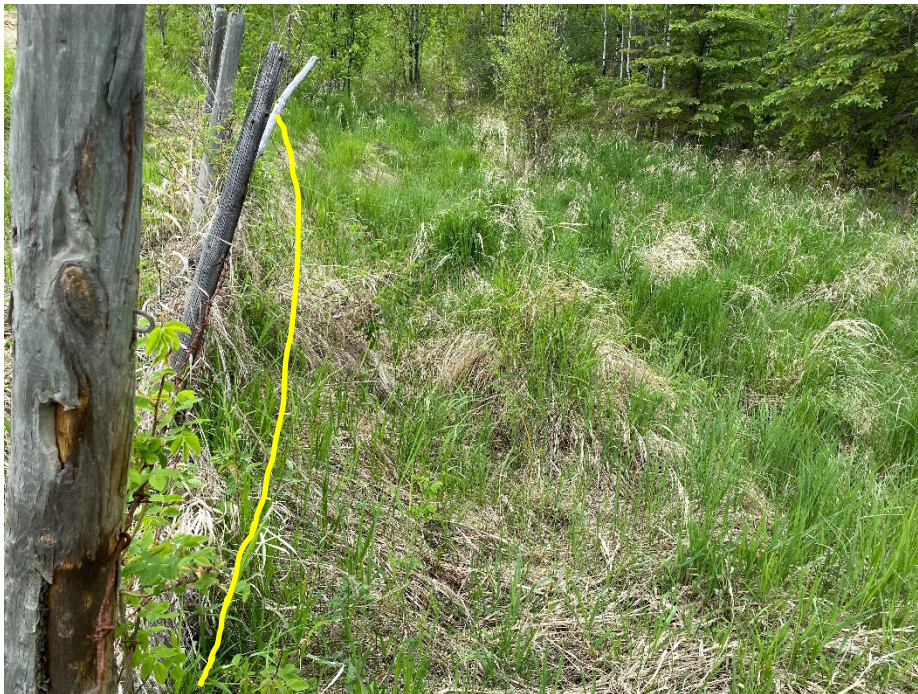
Photo 10: Possible toe bulge and leaning fence on east side of site. Looking northeast.
