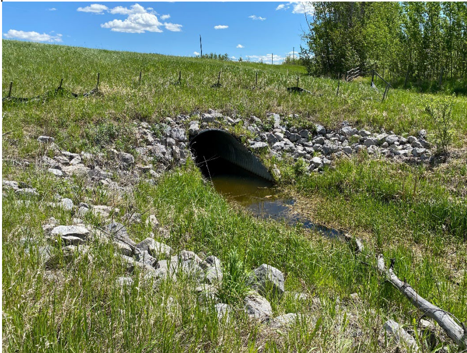
Photo 5: 2120 mm diameter culvert outlet with riprap lining on west side of highway. Looking south.
