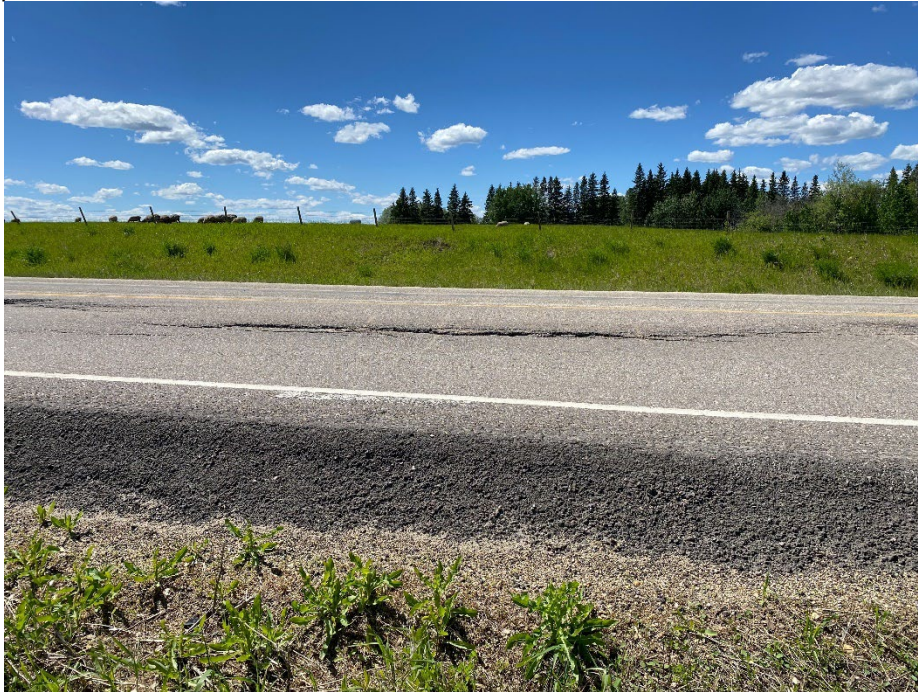
Photo 11: Northbound lane dipping to the east. Looking west.
