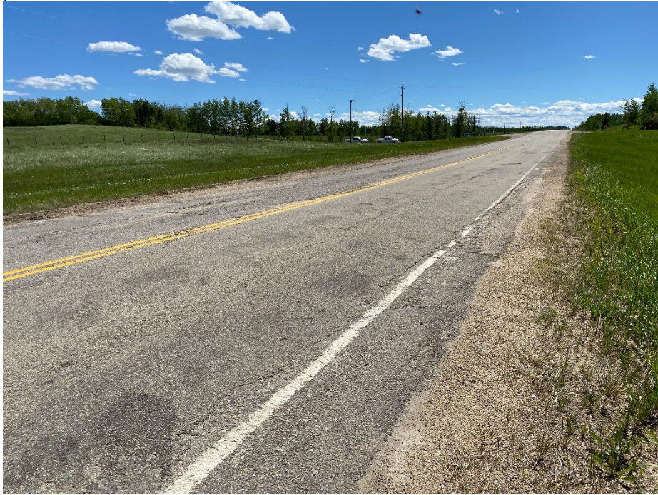
Photo 3: Pavement condition at south end of NC36-1. Looking southeast.
