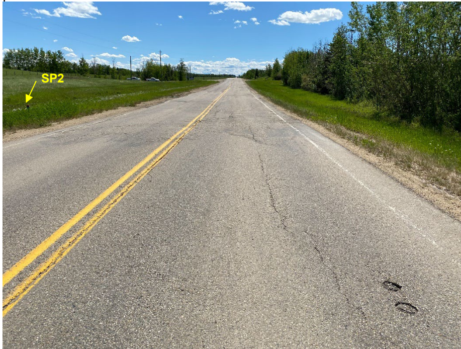
Photo 1: Longitudinal pavement cracks at north end of south bound lane at NC36-1. Looking south.
