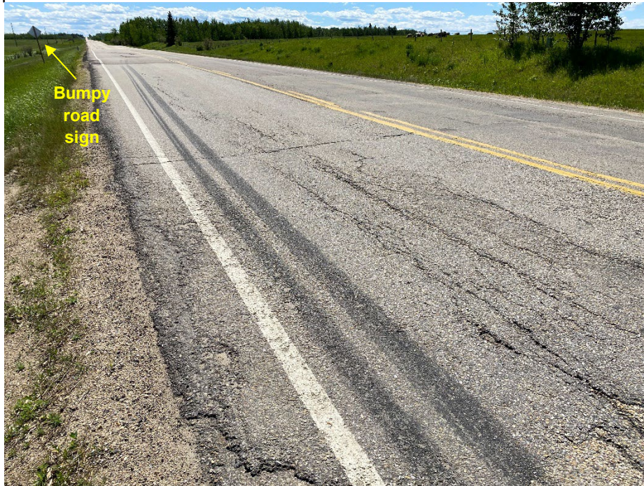
Photo 13: Cracking and tire marks visible north of (after) semi-circular cracking. Looking southwest.
