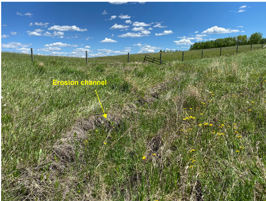
Photo 6: Erosion channel leading from riprap to fence line on east side of highway. Looking southeast.
