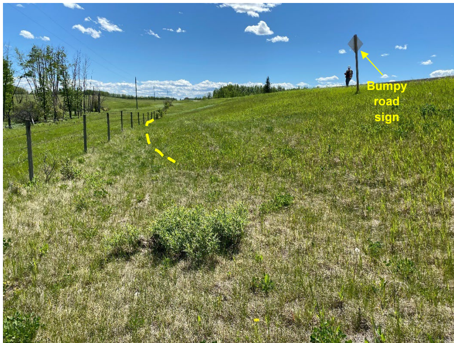
Photo 14: Slight toe bulging at base of embankment. Looking south.
