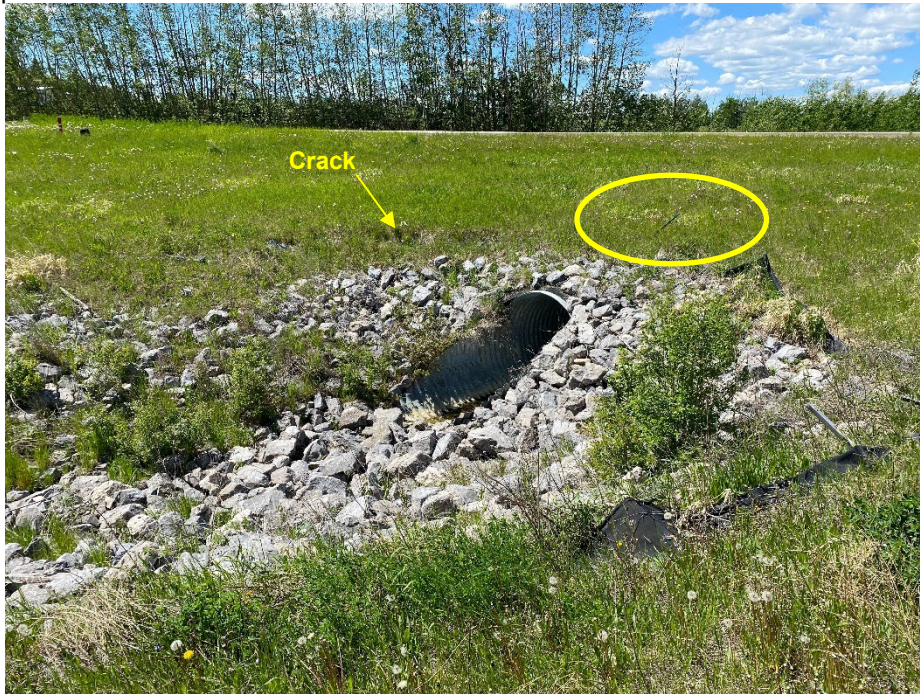
Photo 9: Depression and crack above 2120 mm diameter culvert and riprap, looking northwest.
