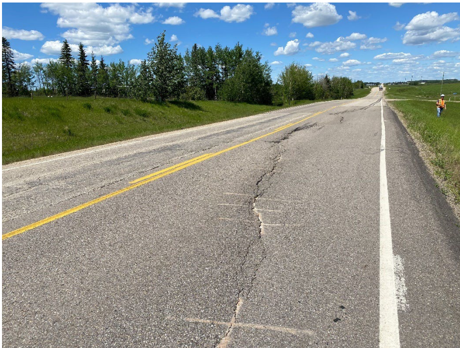
Photo 12: Pavement cracking approximately at south extent of NC36-2. Looking north.
