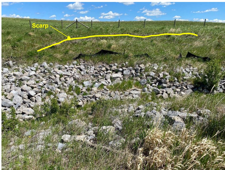
Photo 8: Scarp on east side of riprap lined channel. Looking east.
