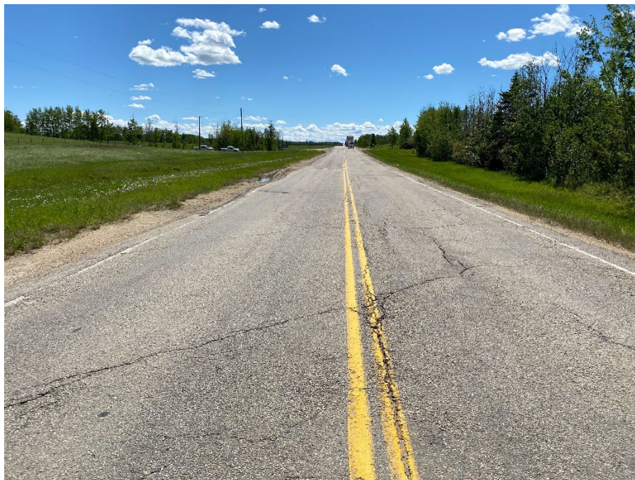
Photo 2: Cracks reflecting through 2018 pavement patch at NC36-1. Looking south.
