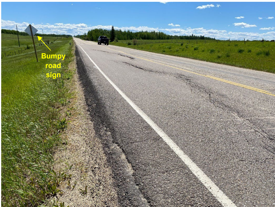
Photo 10: Pavement cracking at approximately north extent of NC36-2. Looking southwest.
