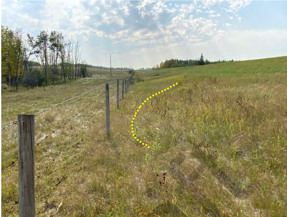
Photo 5: Slight toe bulging at base of embankment. Looking south.
