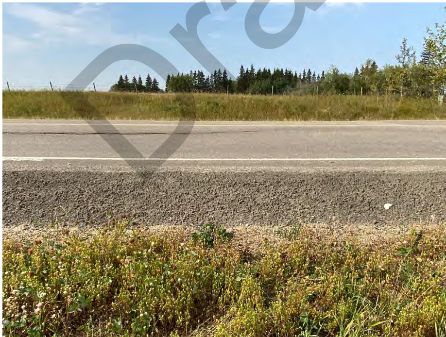
Photo 4: Northbound lane dipping to the east. Looking west.
