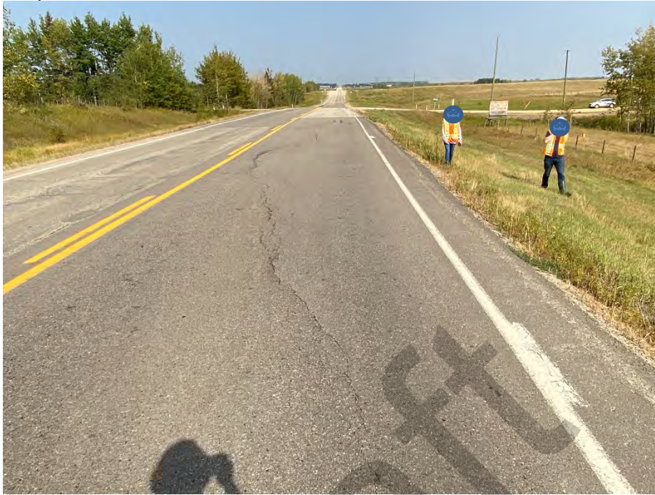
Photo 3: Pavement cracking approximately at south extent. Looking north.
