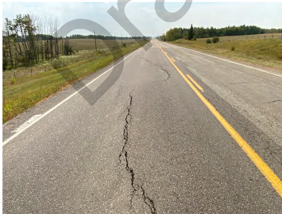
Photo 2: Pavement cracking on northbound lane. Dip towards east. Looking south.
