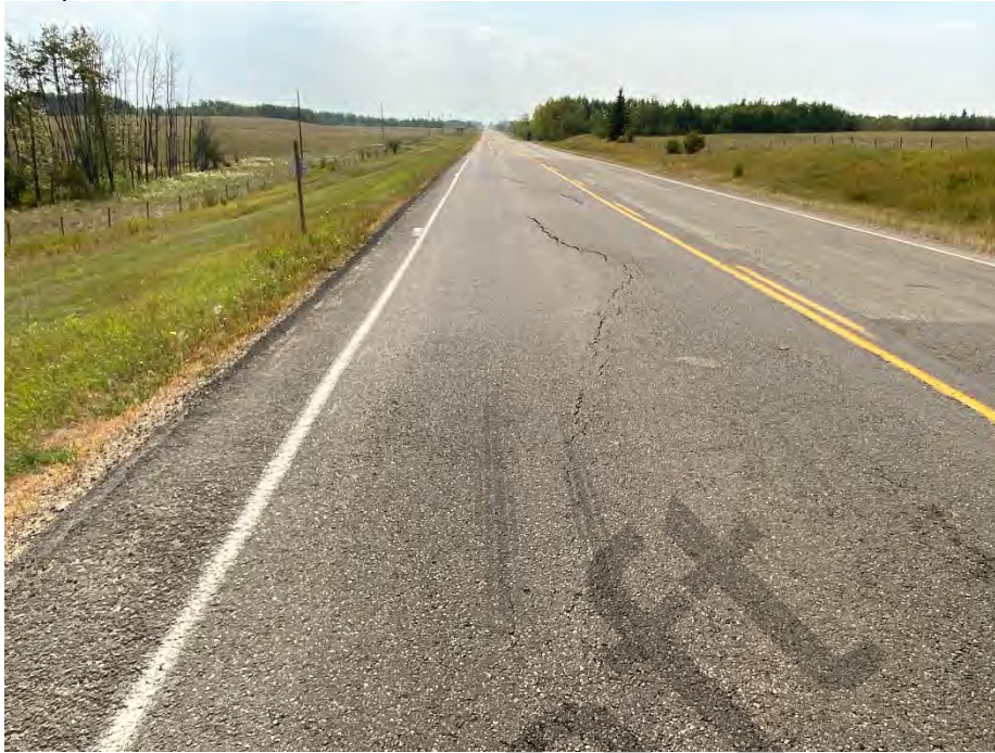
Photo 1: Pavement cracking at north extent. Tire marks visible. Looking south.
