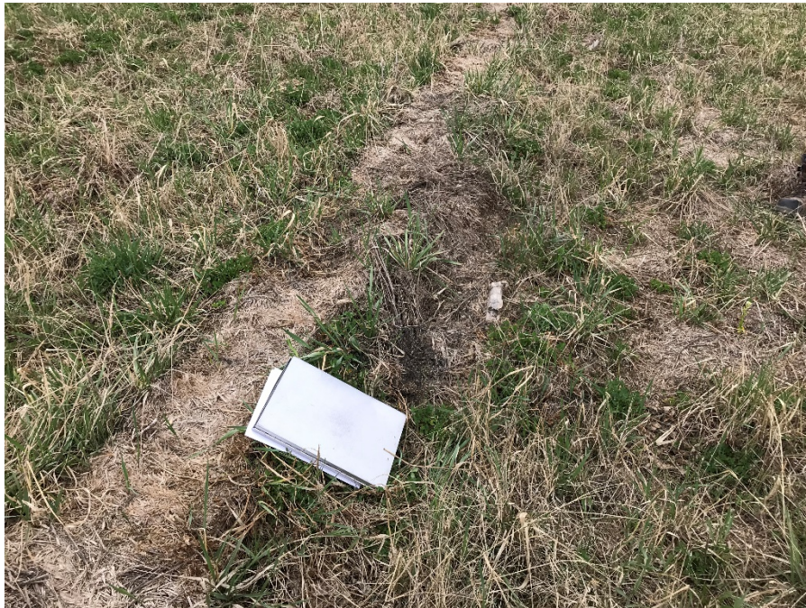
Photo 7: Ground crack more pronounced south of JW-S11.
