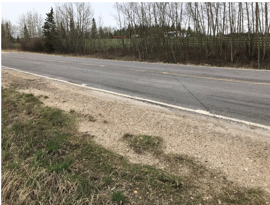
Photo 2: Dip in northbound lane repaired during 2018 patch. Saw cut visible. Looking west.
