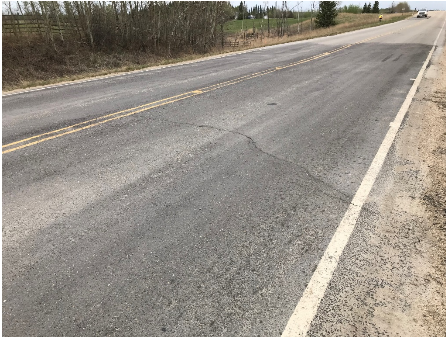
Photo 1: Old pavement crack reflected through 2018 patch. on northbound lane. Looking north.
