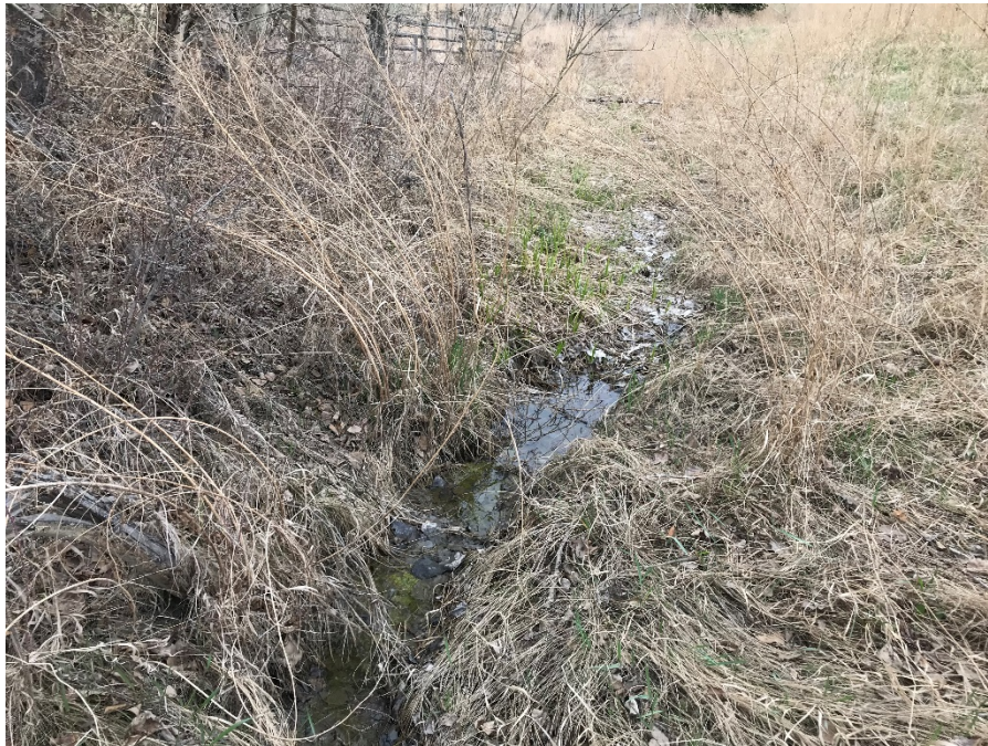
Photo 9: Erosion gully with flowing water in west ditch. Looking north.
