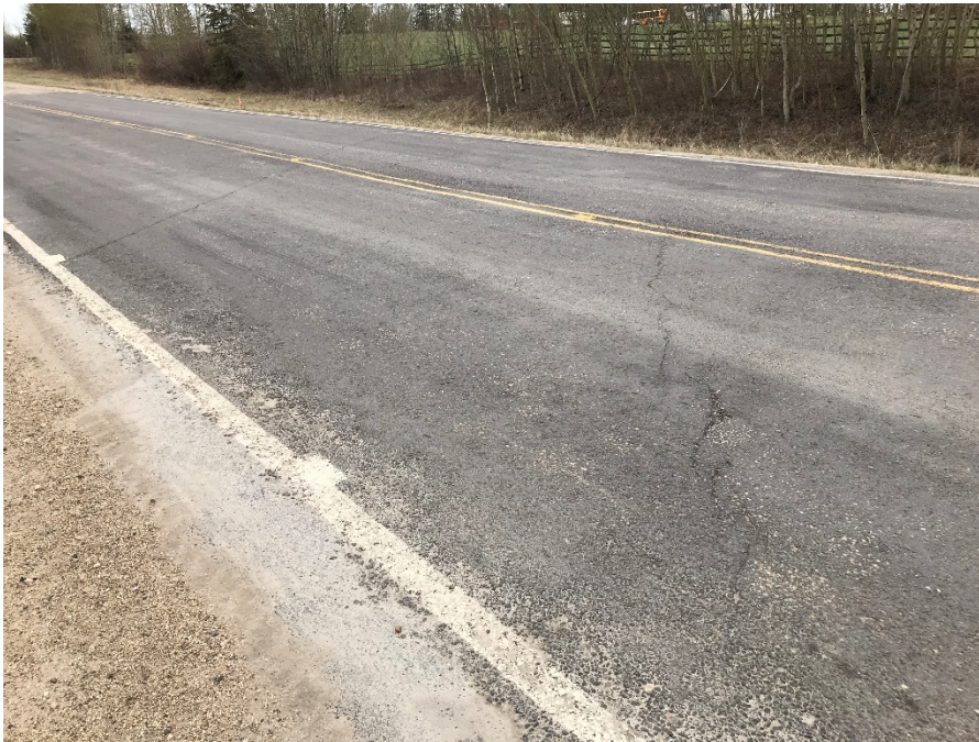
Photo 3: Crack reflecting through 2018 patch. Looking southwest.
