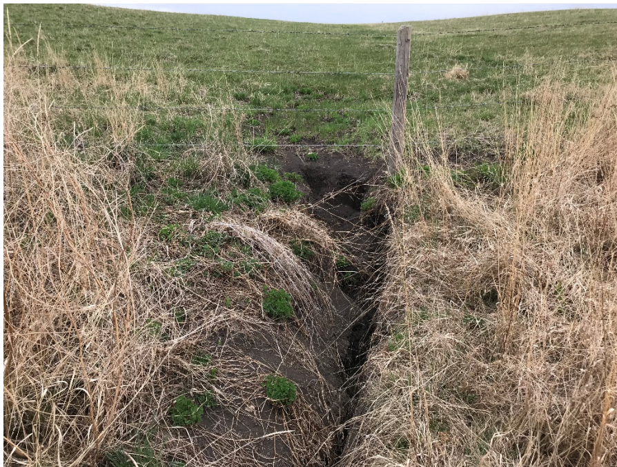
Photo 6: Erosion channel leading from rip rap to fence line. Looking east.
