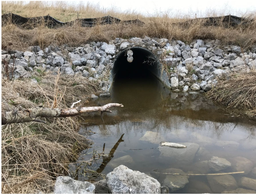
Photo 5: New 2120 mm diameter culvert outlet with riprap lining west of highway. Looking east.
