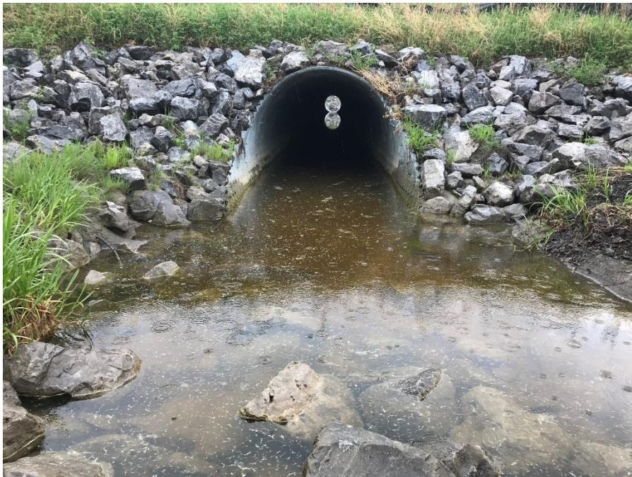
Photo 4: New 2120 mm diameter culvert outlet with riprap lining west of highway. Looking east.
