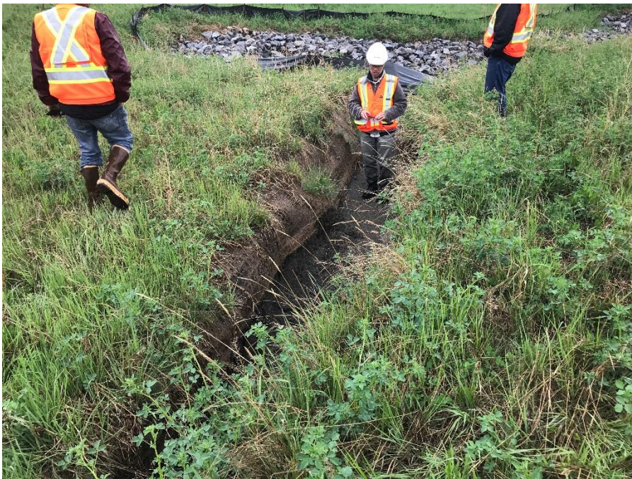
Photo 6: View of east slope. Erosion channel leading to rip rap. Looking south
