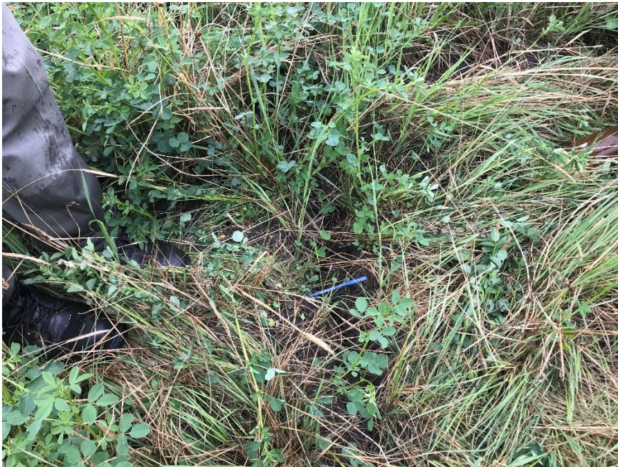
Photo 5: Erosion approximately 150 mm wide at northeast side of riprap channel.
