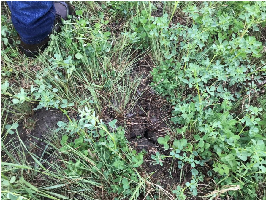
Photo 7: Ground crack south of JW-S11
