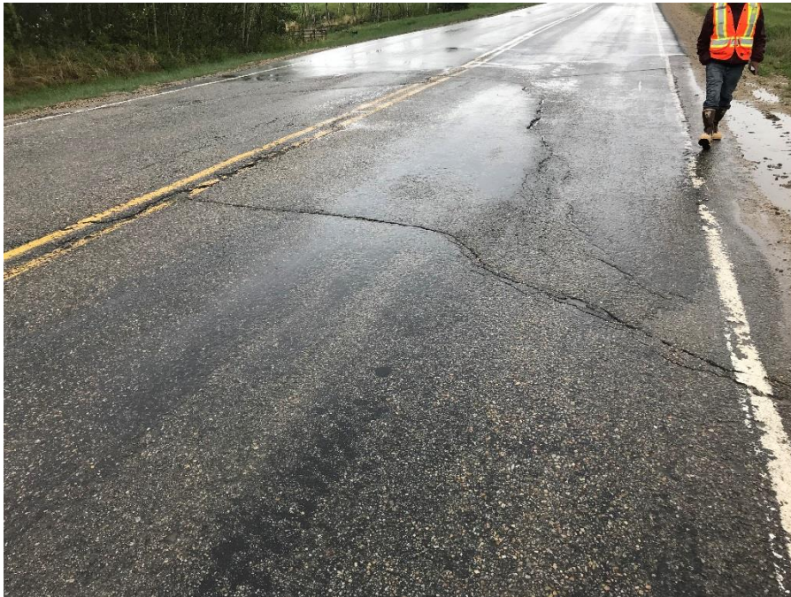
Photo 1: Pavement cracking on northbound lane. Looking north.
