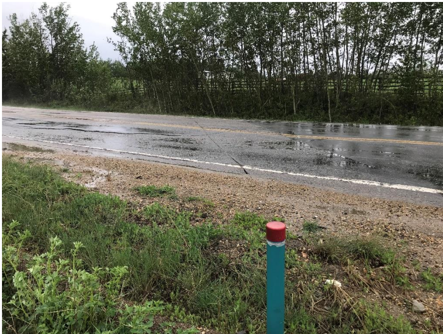
Photo 2: Dip in northbound lane unchanged. Saw cut visible. Looking west.
