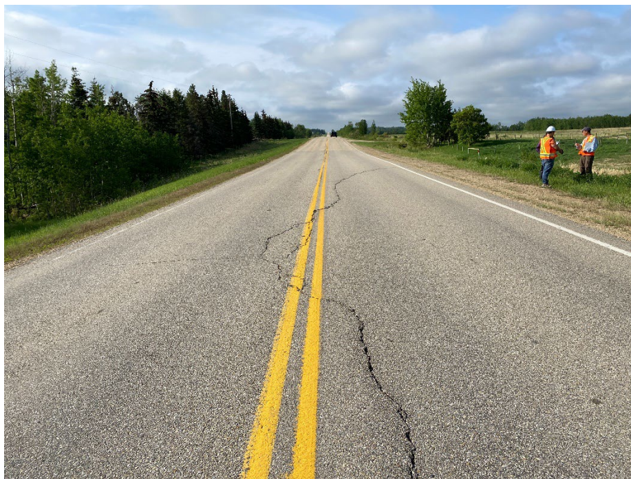
Photo 2: Approximately midway of semi-circular crack near SI-1R. Looking south.
