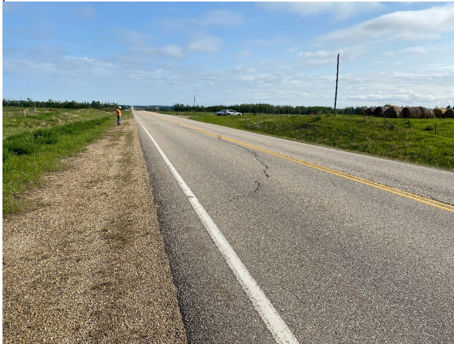
Photo 1: South limits of semi-circular crack. Looking north.
