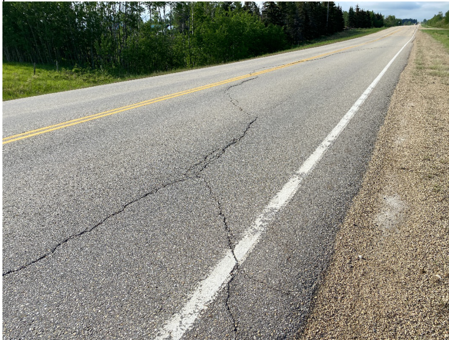
Photo 3: North limits of semi-circular crack. Looking southeast.
