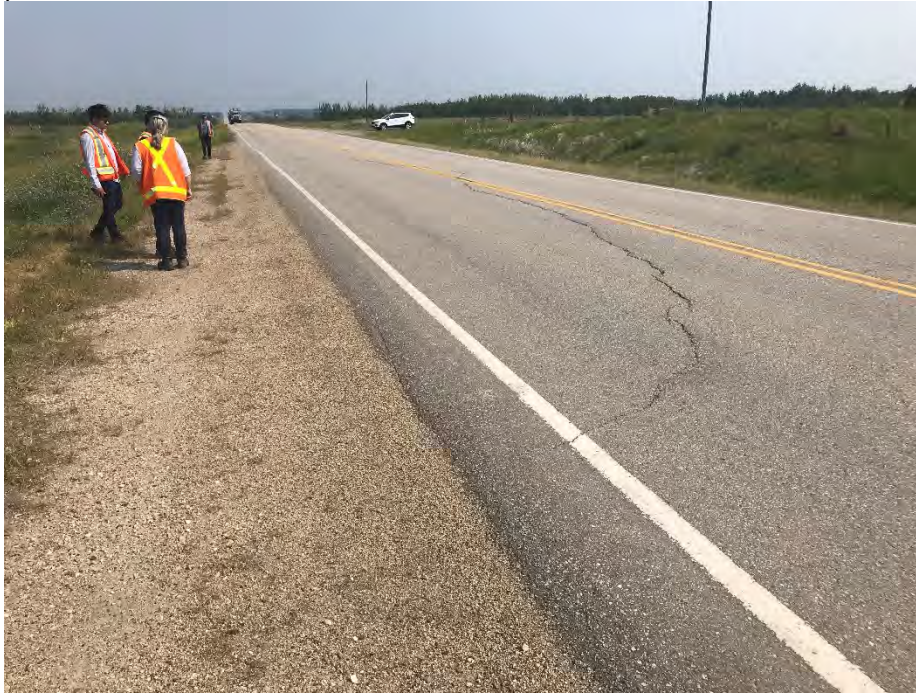
Photo 1: South limits of semi-circular crack. Looking north.
