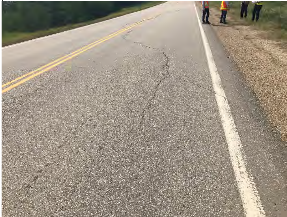
Photo 3: North limits of semi-circular crack. Looking south.
