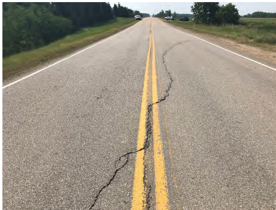
Photo 2: Approximately midway of semi-circular crack near SI-1R. Looking south.
