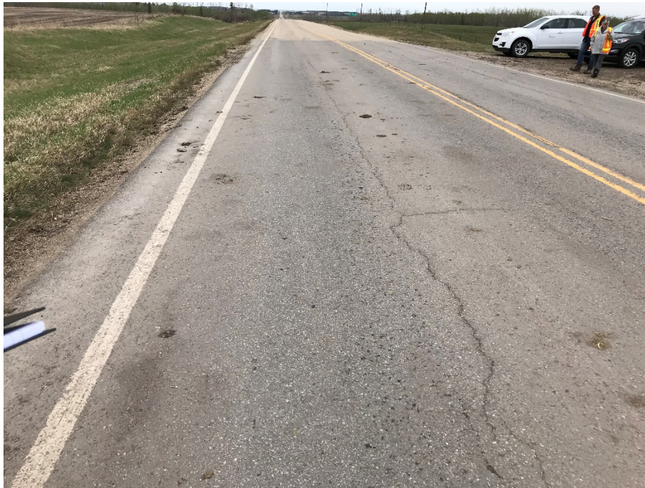
Photo 1: New pavement cracking reflected through recent patch on southbound lane in front of access road. Looking north.
