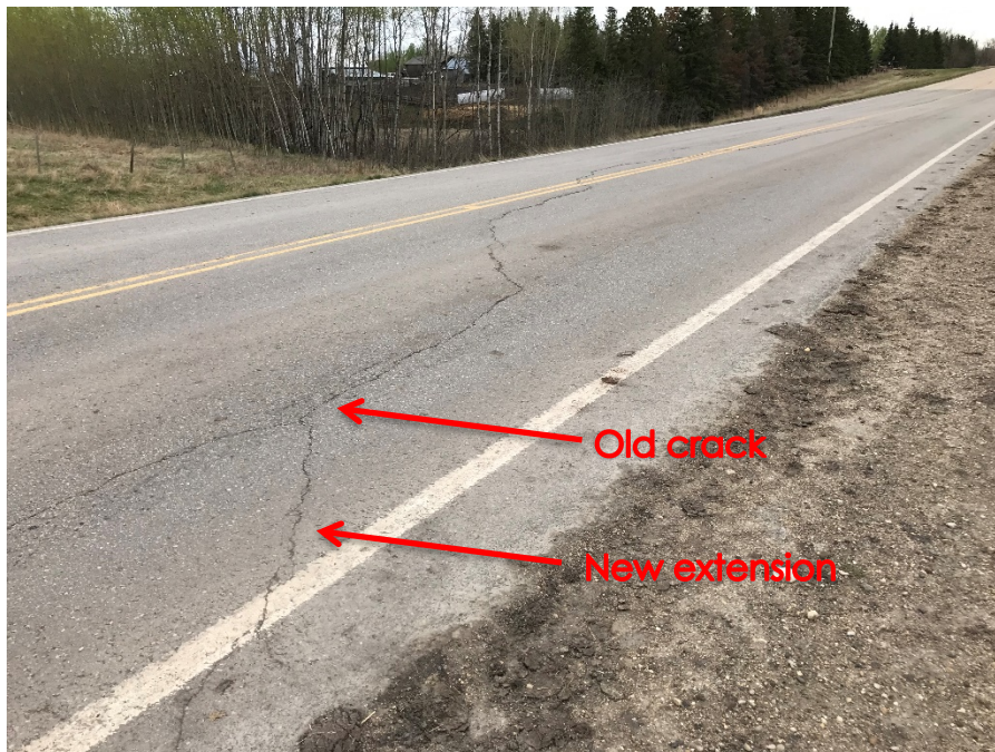
Photo 2: New extension of circular crack on southbound lane near S110-1. Looking southeast.
