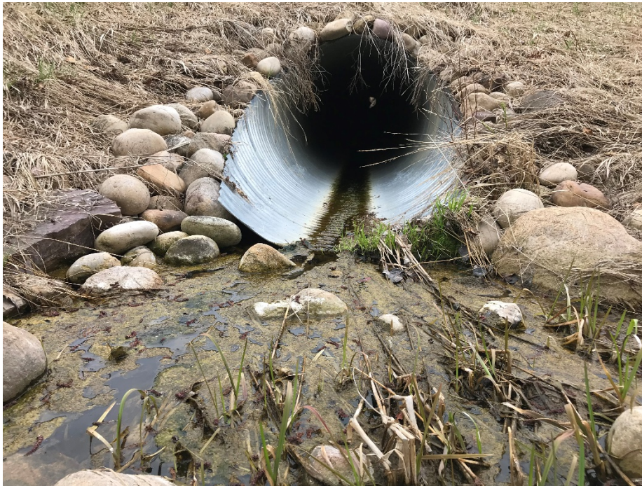
Photo 5: The 1200 mm diameter culvert is in good condition. Slow draining at outlet. Looking south.
