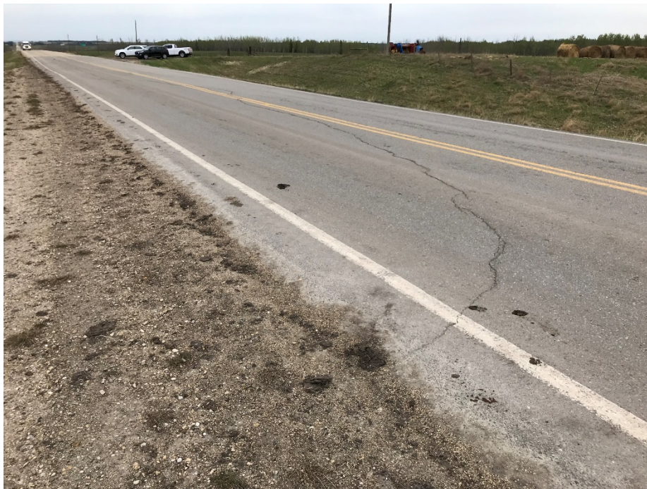
Photo 3: Circular crack near S110-1. Looking northeast.
