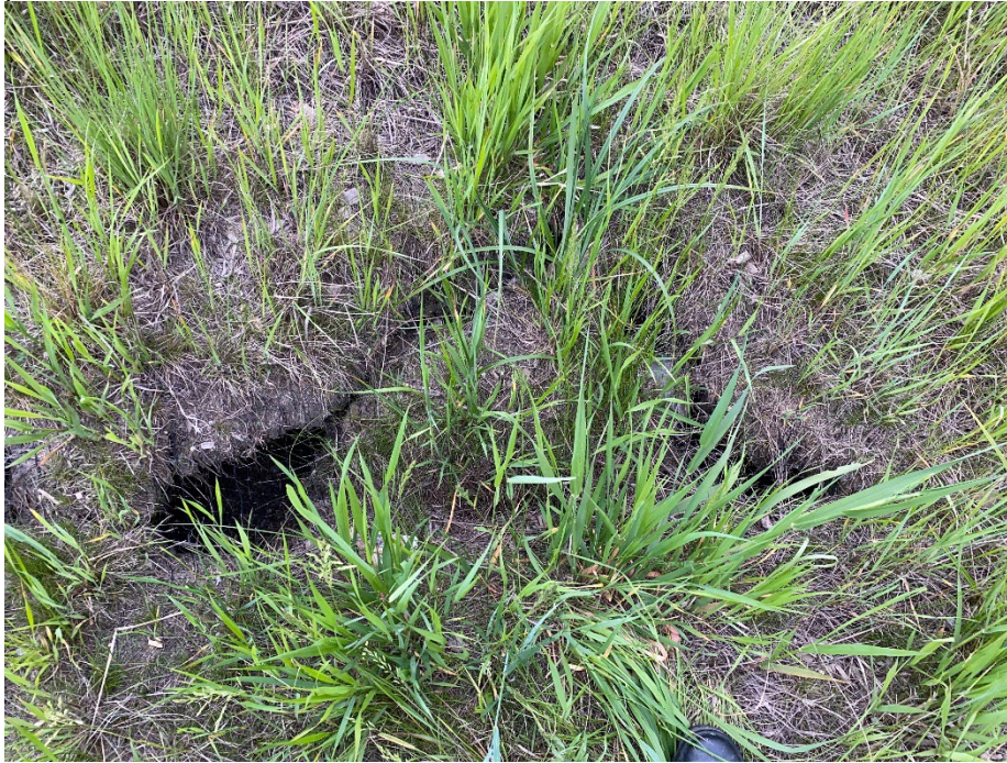
Photo 5: Depression in west embankment slope along pile wall alignment, near SI19-03. Looking east.
