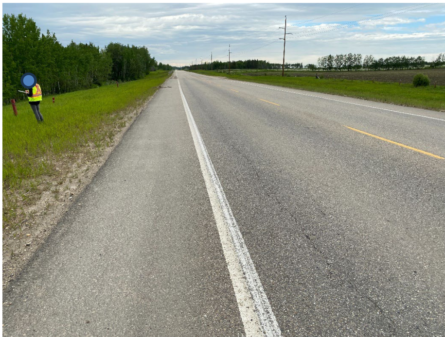
Photo 2: Highway condition within repair zone, looking north.
