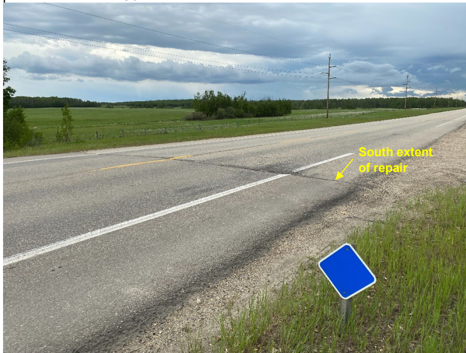
Photo 1: Bump at south extent of highway repair in SBL. Looking southeast.
