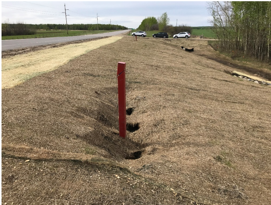
Photo 4: Depression at SI19-02. Looking south.
