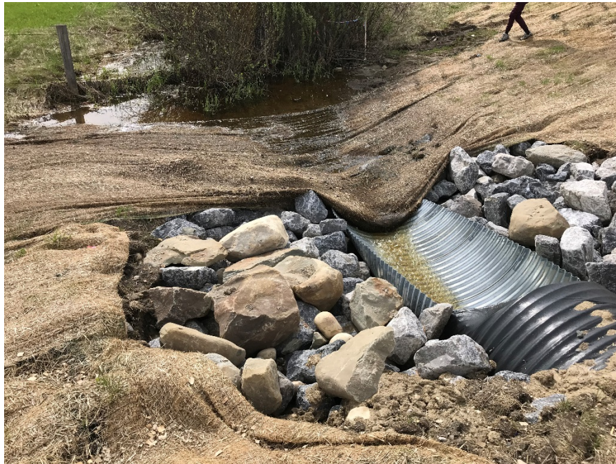
Photo 7: Erosion matting displaced at culvert inlet. Looking southeast.
