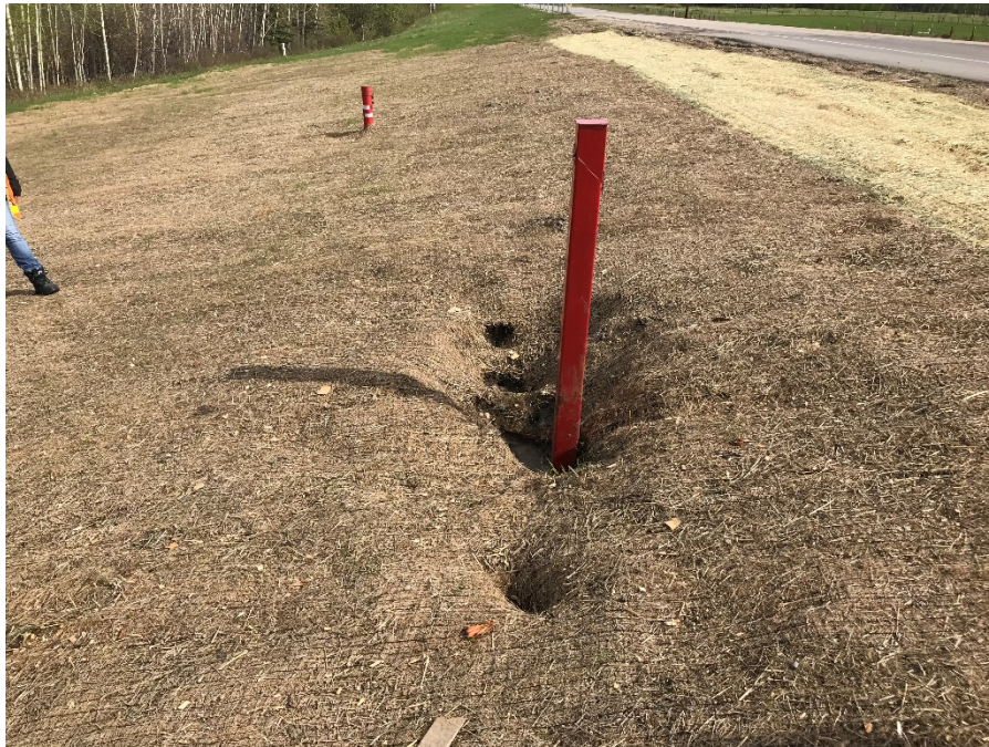
Photo 5: Depression at S119-03. Looking north.
