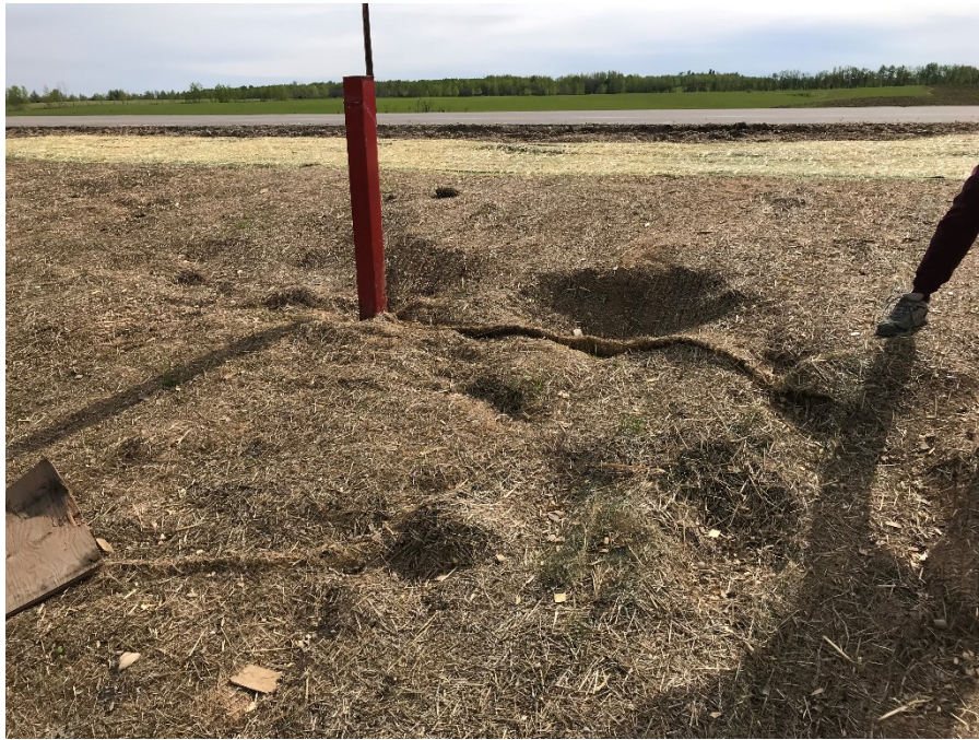
Photo 3: Depression at SI19-01. Looking east.
