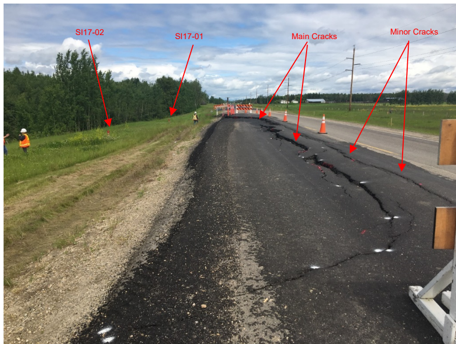
Photo 7: Pavement cracking from Call-Out Inspection. Looking north. Photo taken July 11, 2019.
