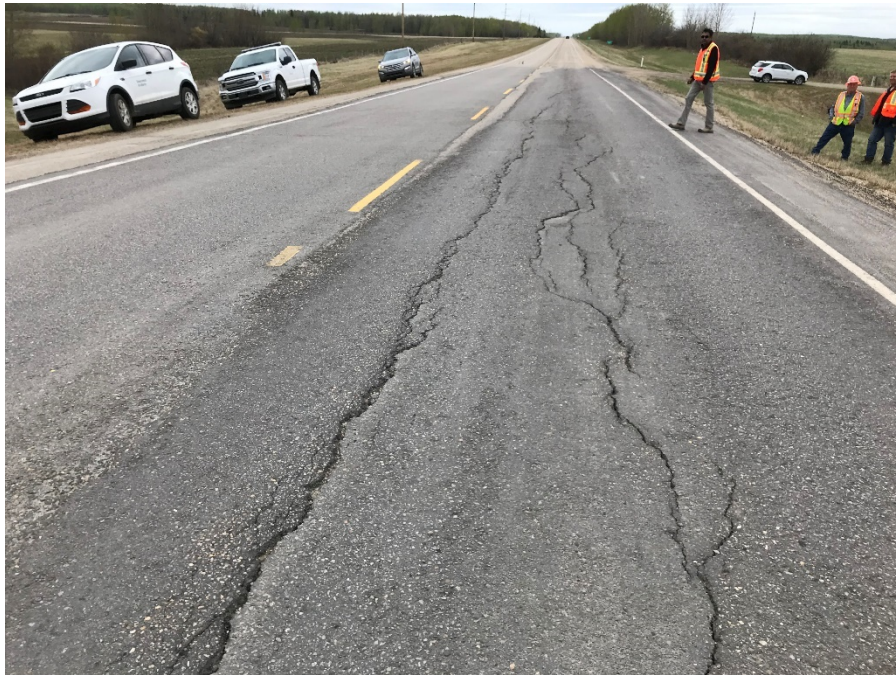
Photo 3: Pavement cracking along southbound lane. Looking south. Photo taken May 14, 2019.
