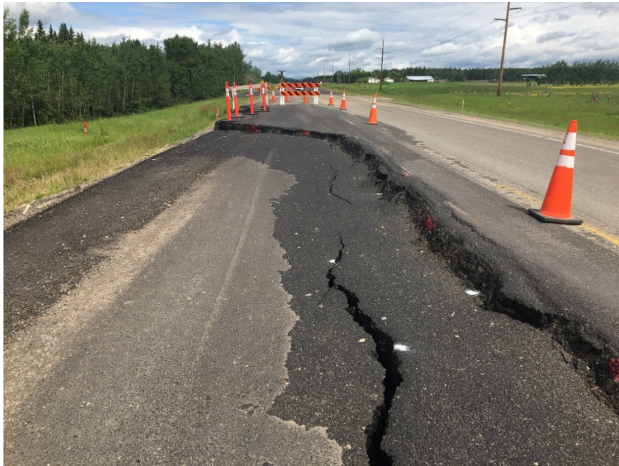
Photo 9: Looking toward north at pavement cracks. Grade drop was obvious. Photo taken July 11, 2019.
