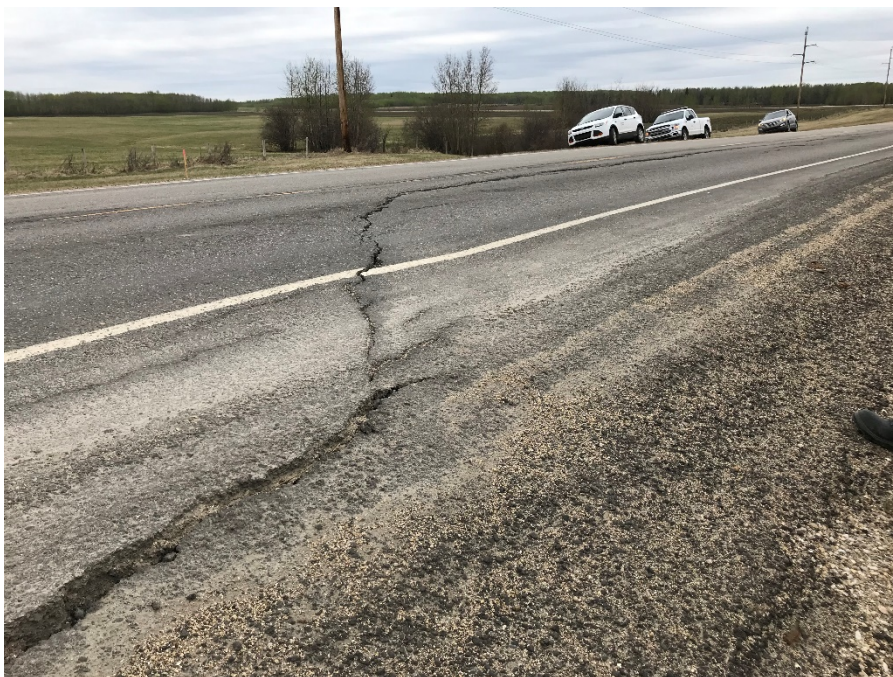
Photo 2: Semi-circular pavement crack along southbound lane. Looking southeast.
