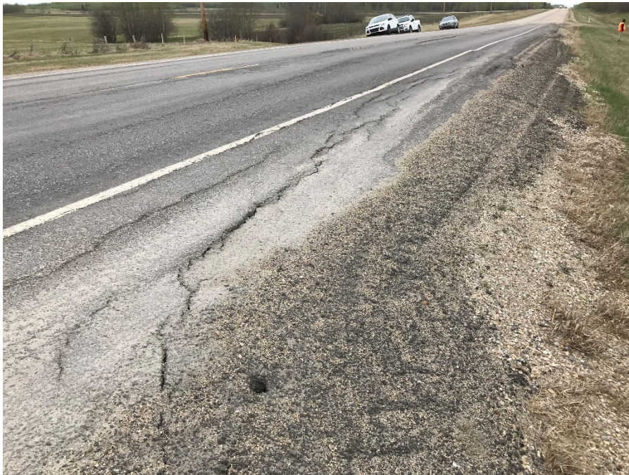
Photo 1: Cracks reflecting through Highway 22 patch along west shoulder. Looking south.
