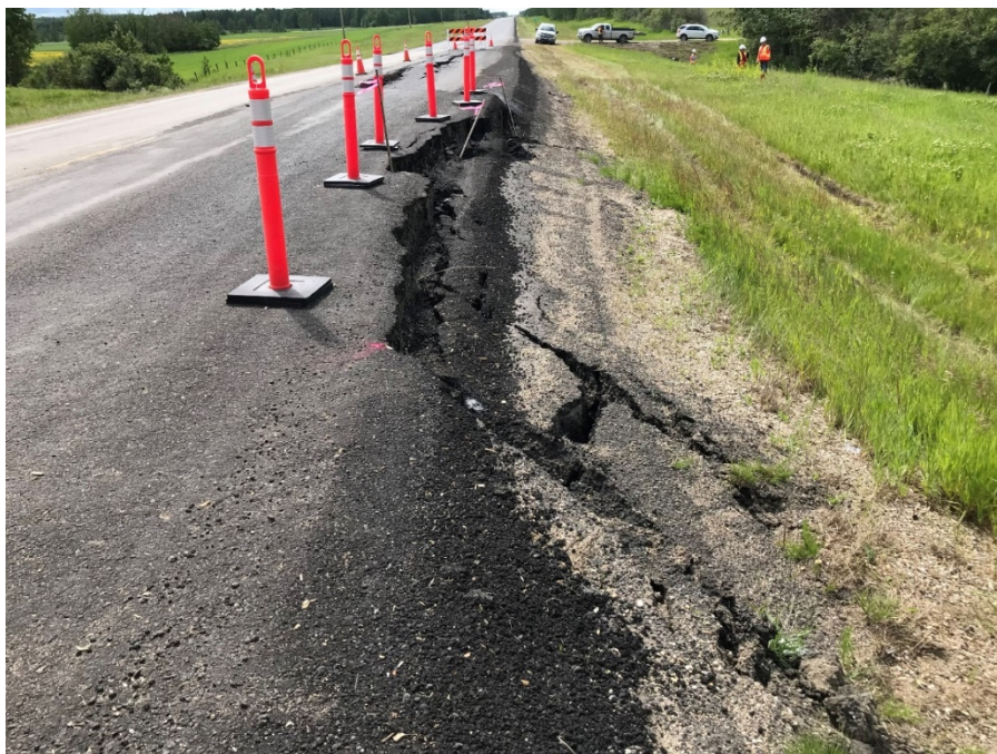
Photo 8: Overall site and pavement cracks, looking south. Grade drop was evident. Photo taken July 11, 2019.
