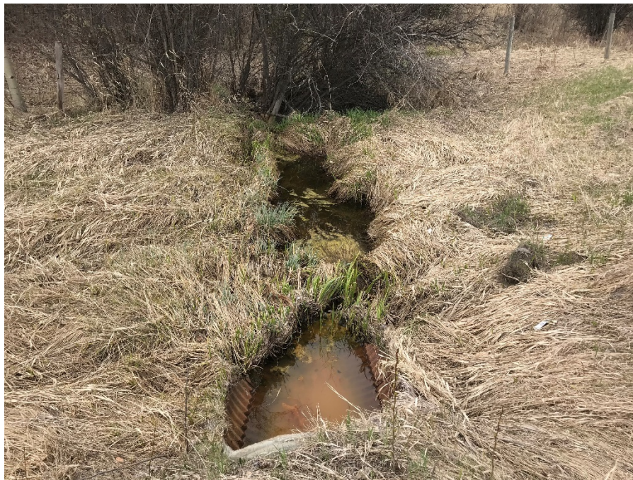
Photo 4: Standing water at the culver outlet on the west ditch. Creek partially blocked. Looking northwest. Photo taken May 14, 2019.
