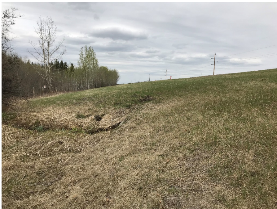
Photo 6: Scour hole around culvert inlet. Culvert rusted through. Looking northwest. Photo taken May 14, 2019.
