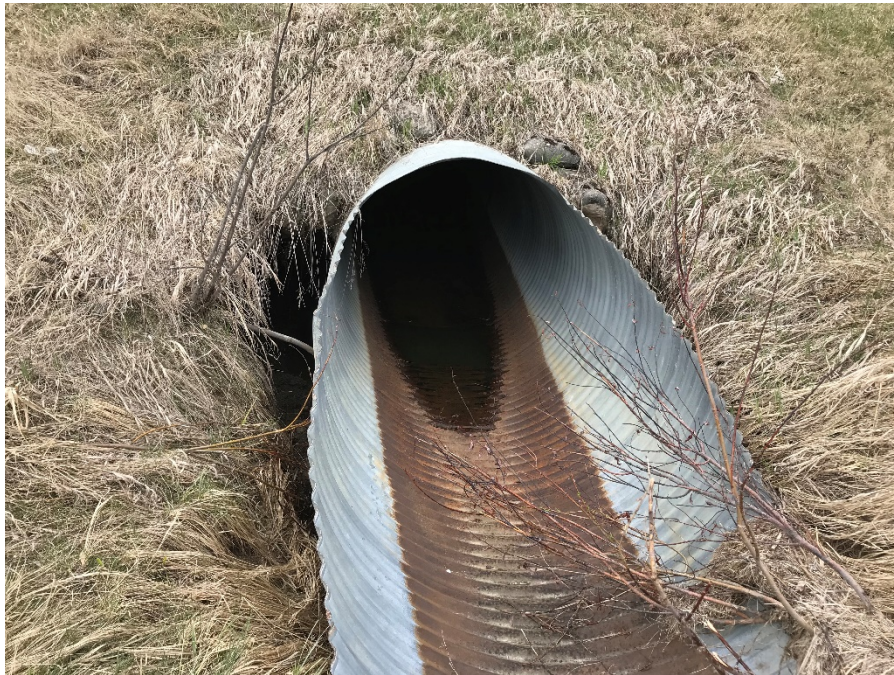
Photo 5: Standing water at the culvert outlet on the west ditch. Looking northwest. Photo taken May 14, 2019.
