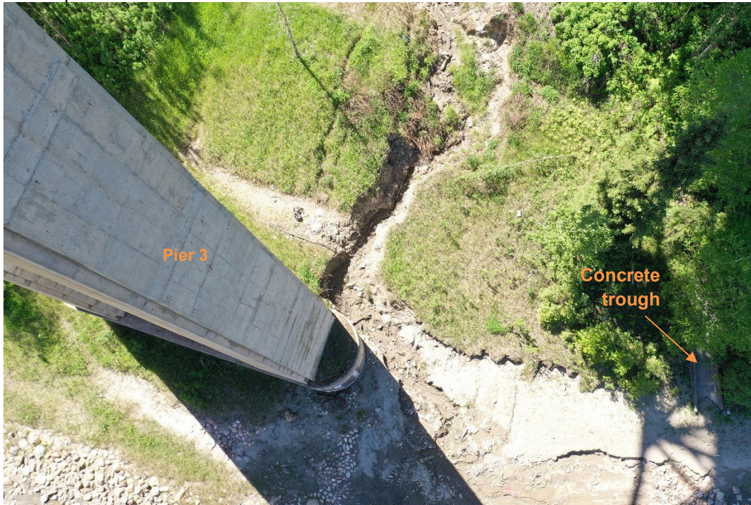
Photo 7: Erosion gully next to west pier at river level, facing southwest.
