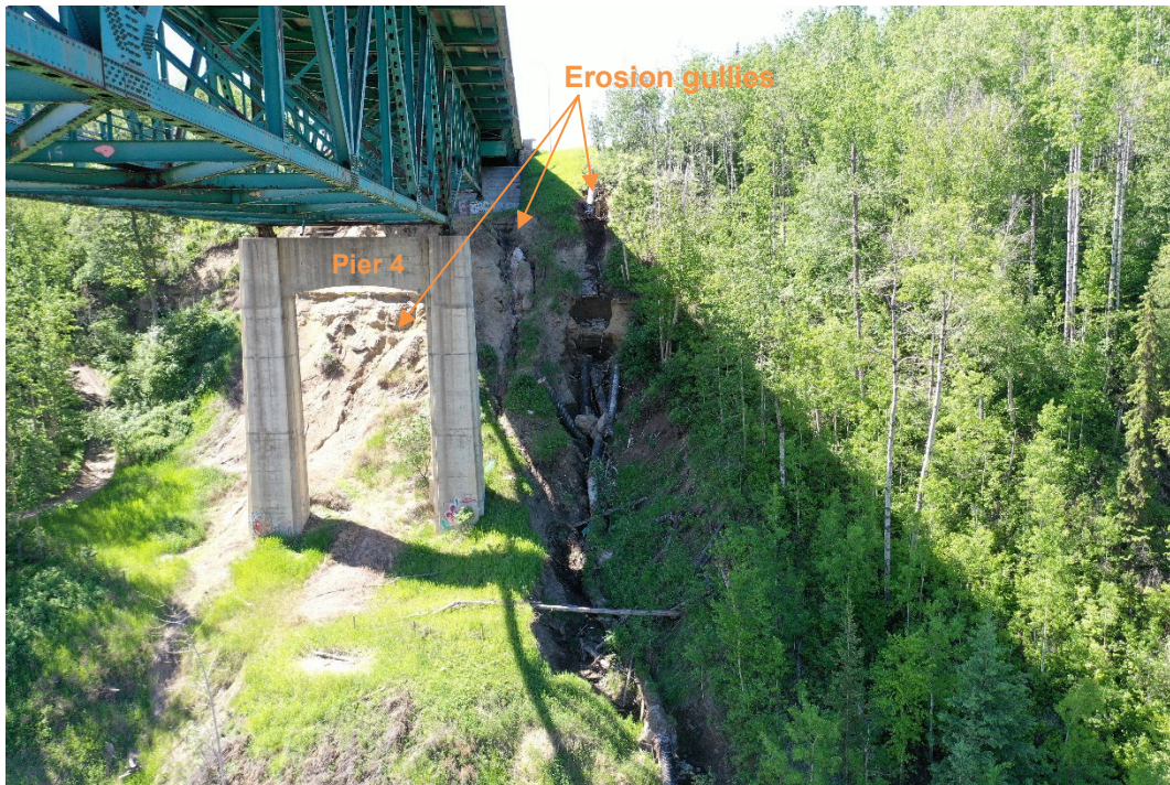
Photo 6: Broken culvert and gully on the north side of the west abutment. Looking west.
