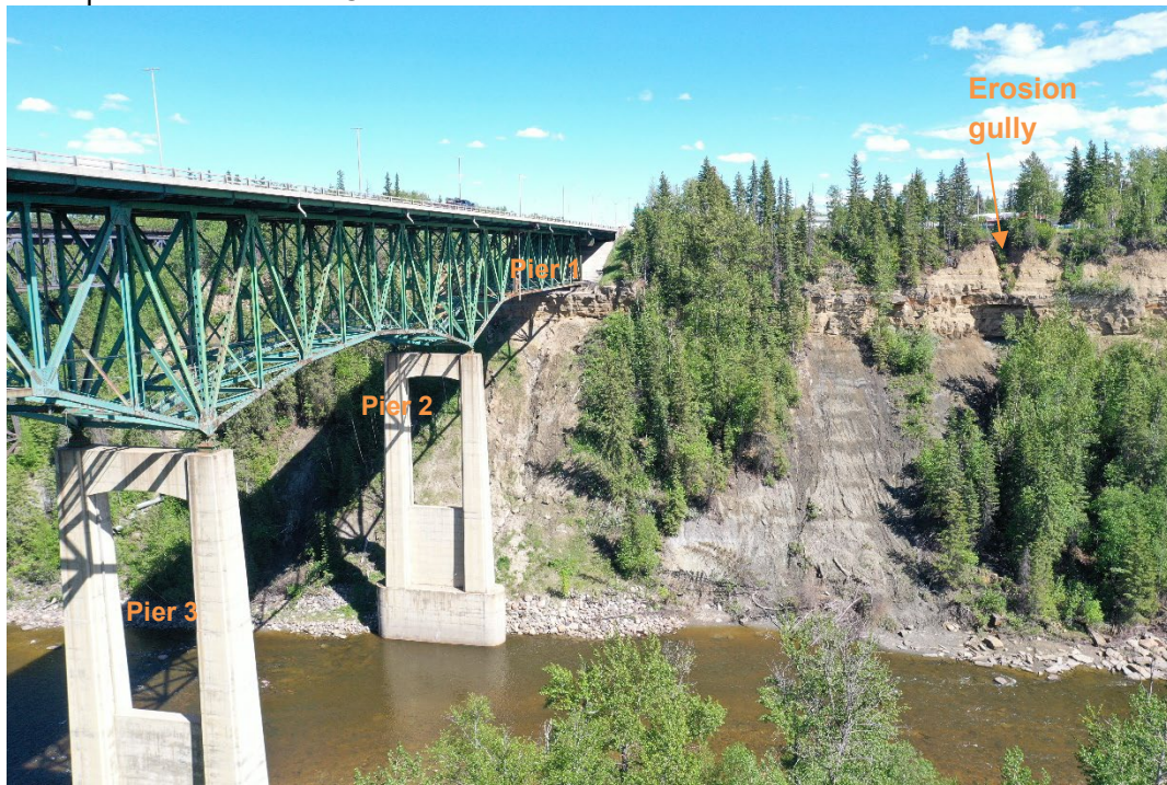
Photo 1: Gullies downslope of east abutment and on east slope, facing northeast.
