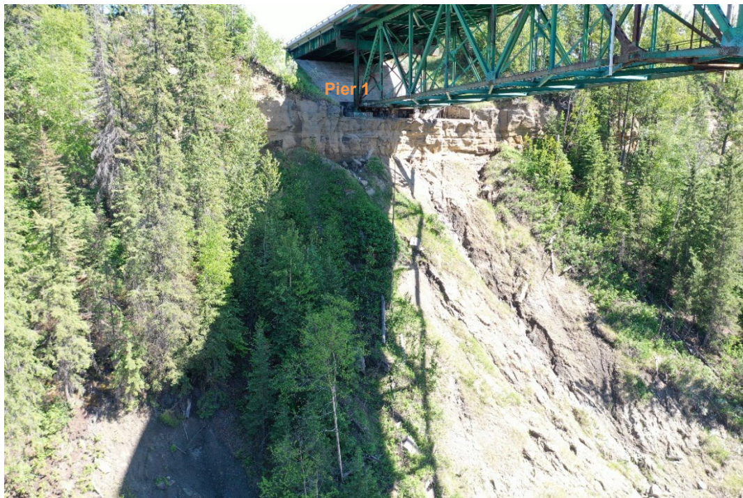
Photo 2: Gullies downslope of east abutment, facing southeast.
