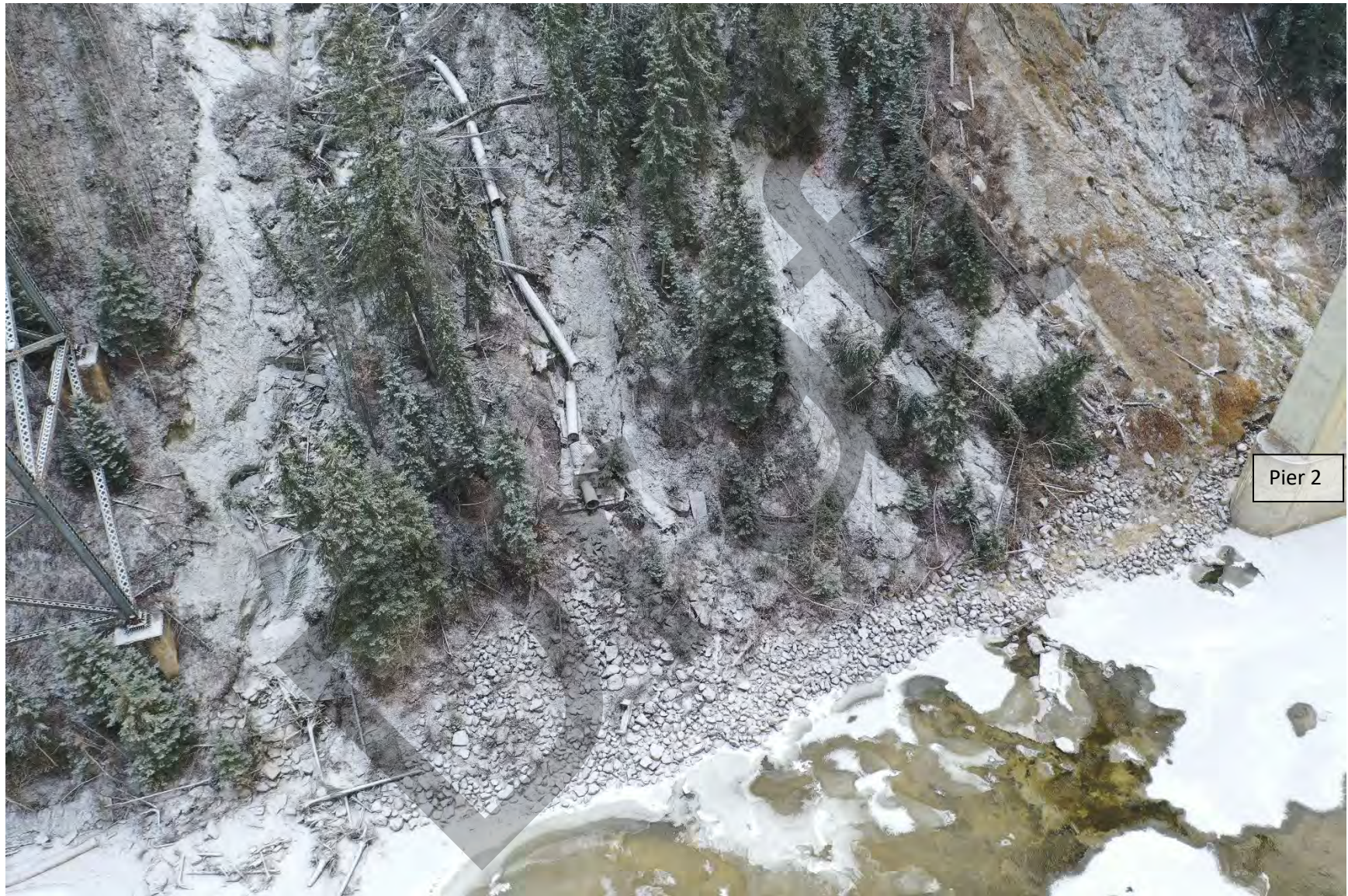
Photo 7: Slope north of east abutment, showing displaced broken culvert sections
