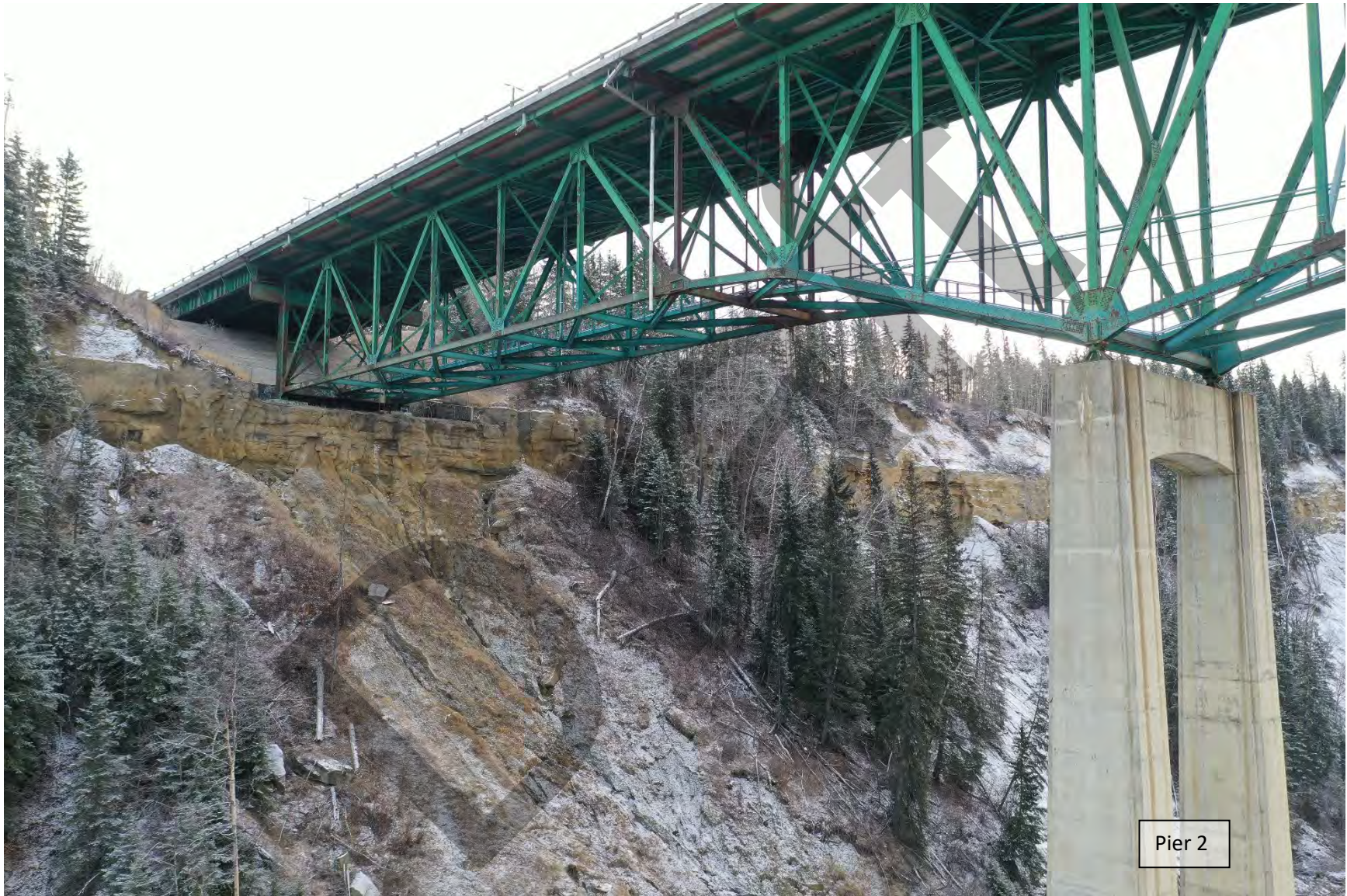
Photo 6: Gullies downslope of east abutment, facing southeast
