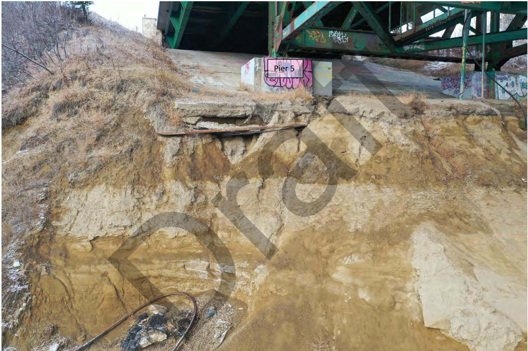
Photo 16: Erosion at west abutment slope, showing abutment undermining
