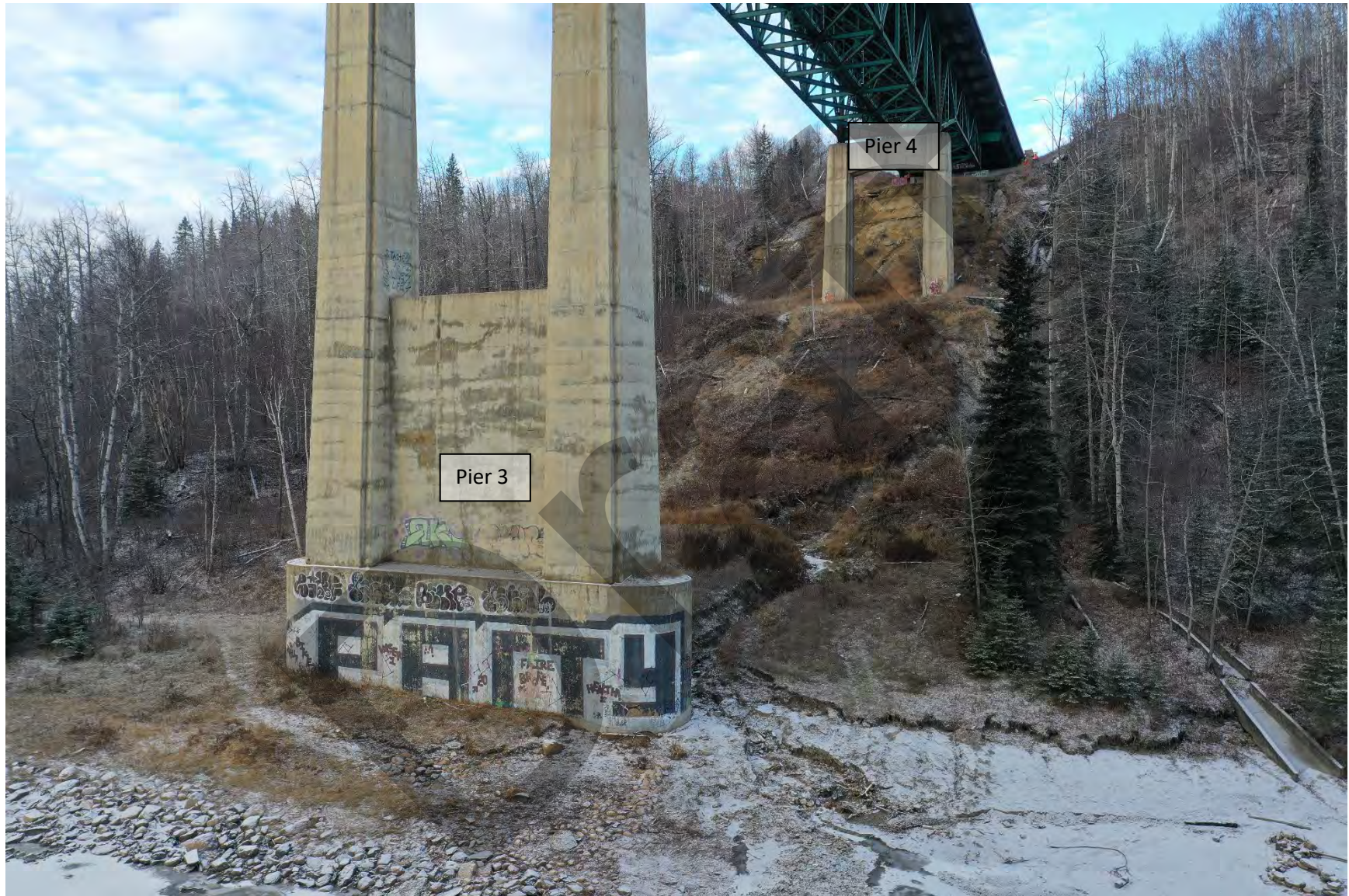
Photo 13: Erosion gullies next to west pier at river level, facing west
