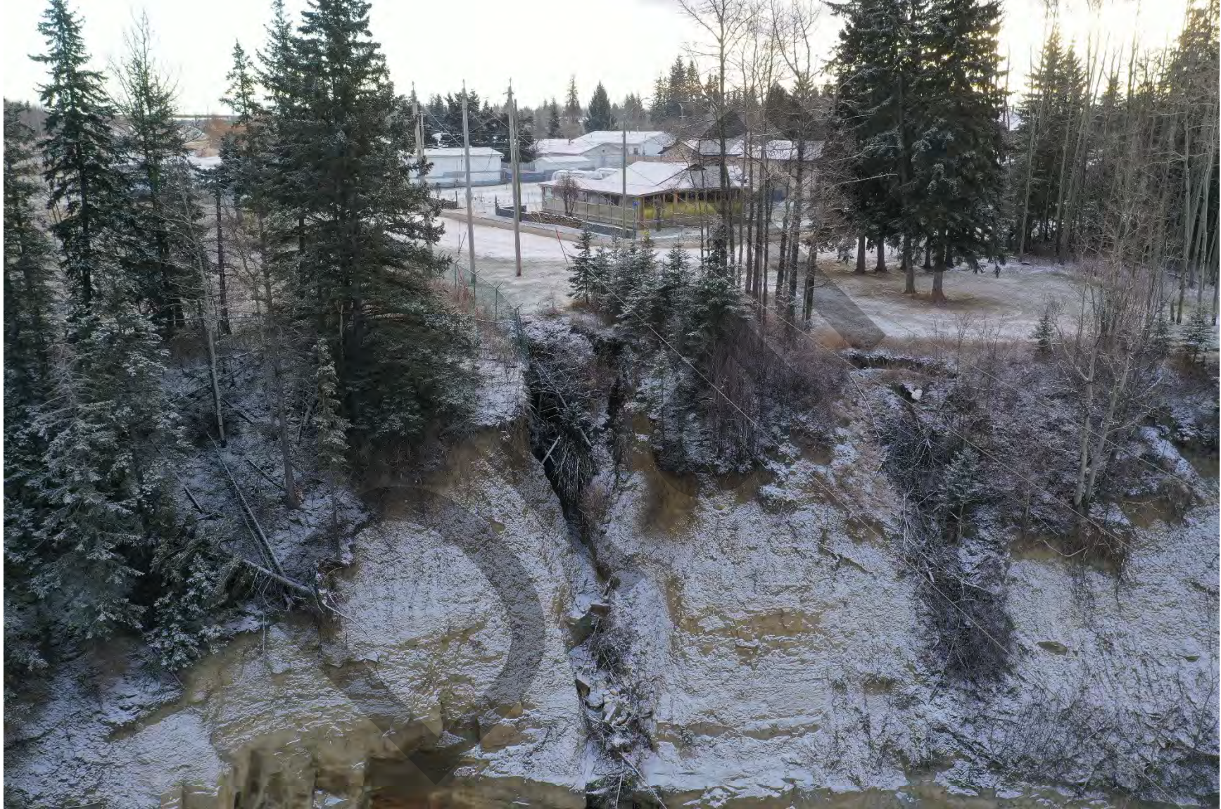
Photo 9: Erosion gully south of east abutment
