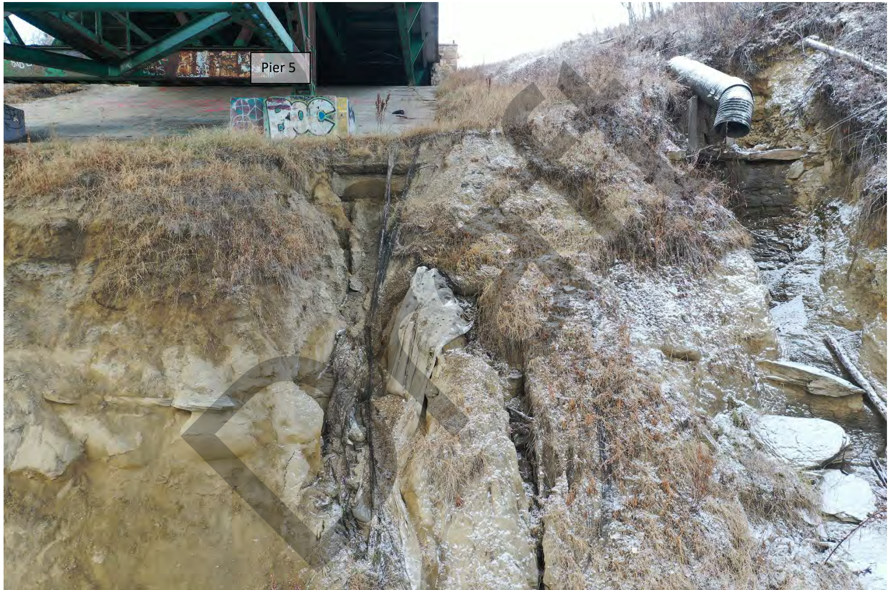
Photo 14: Erosion gullies and broken culvert on north side of west abutment
