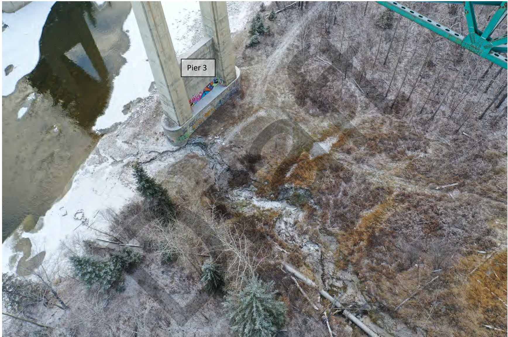
Photo 12: Erosion gullies next to west pier at river level, facing southeast
