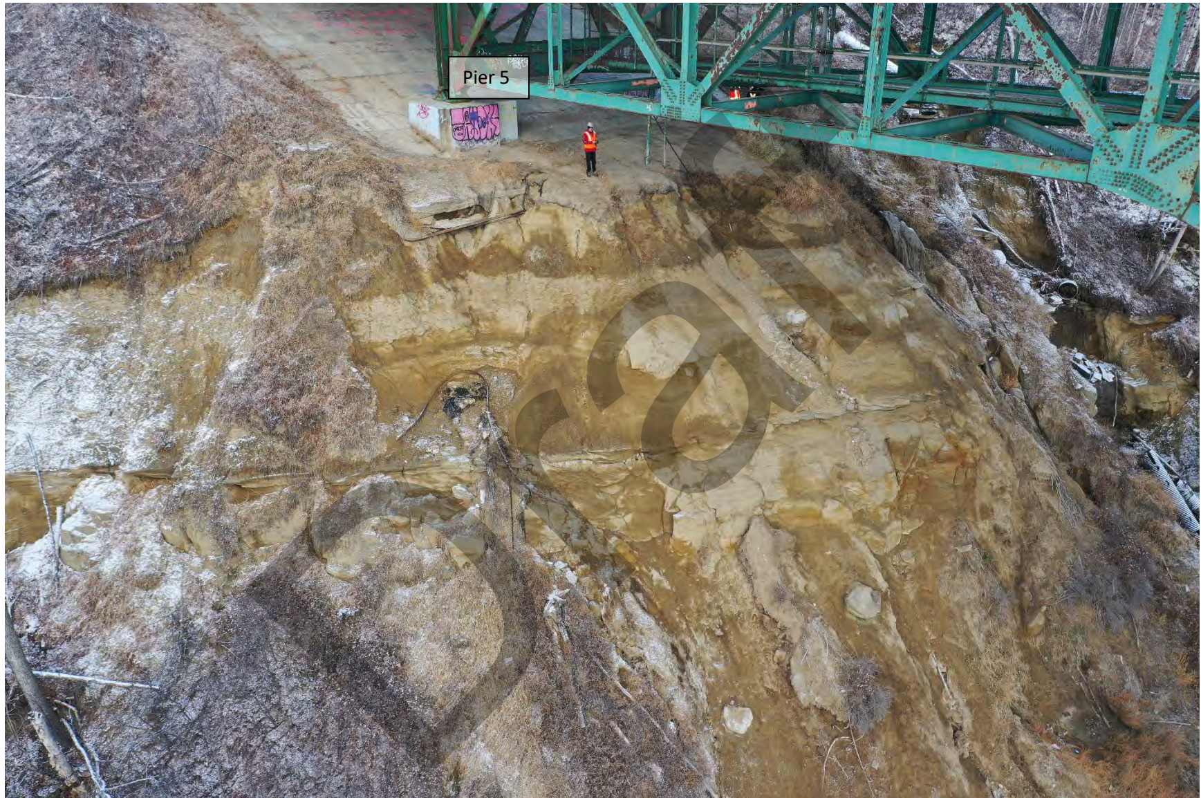
Photo 15: Erosion at west abutment slope, showing abutment undermining and exposed utility cables, facing northwest
