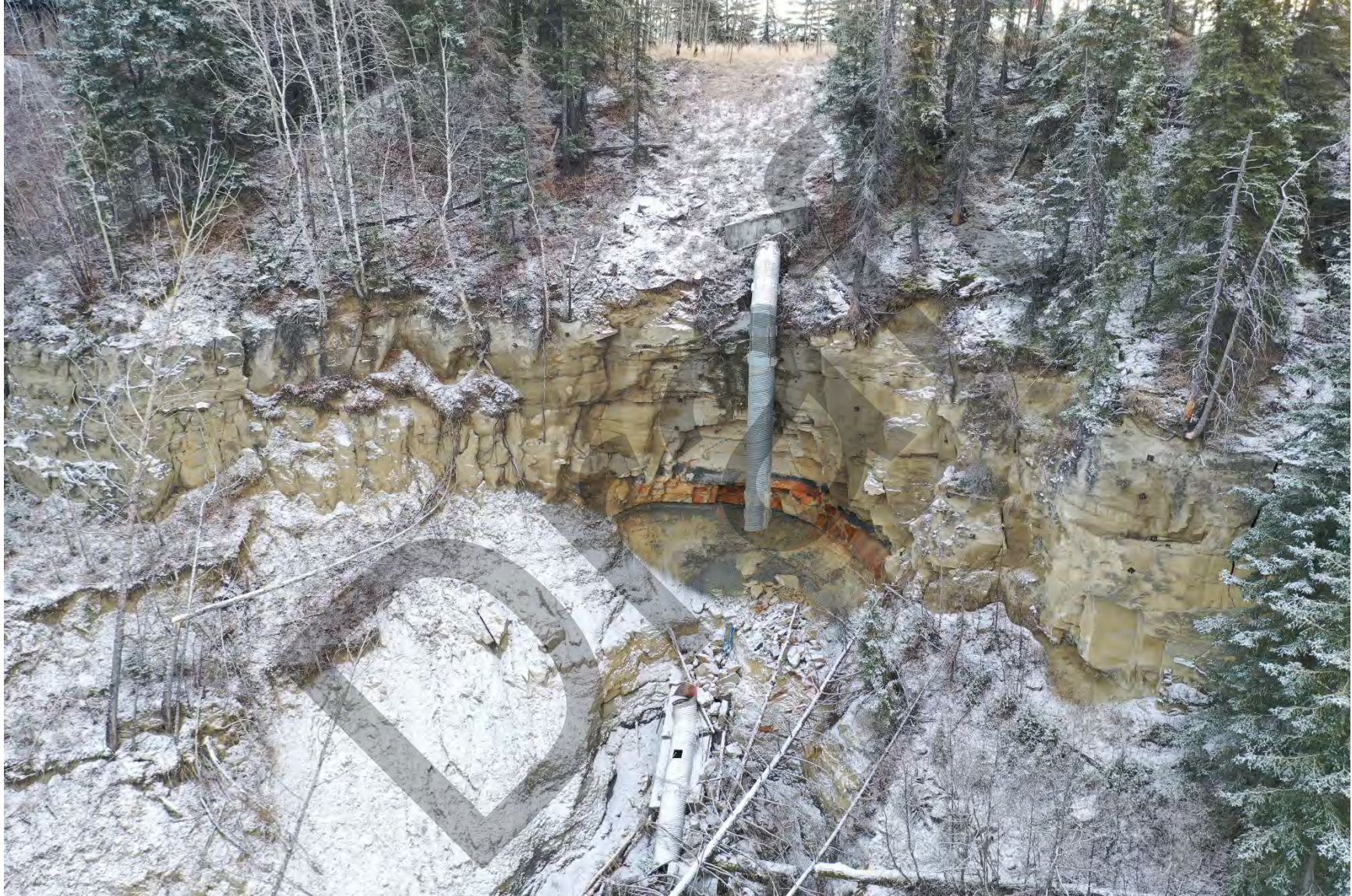
Photo 8: Culvert north of east abutment, showing broken sections and evidence of scour
