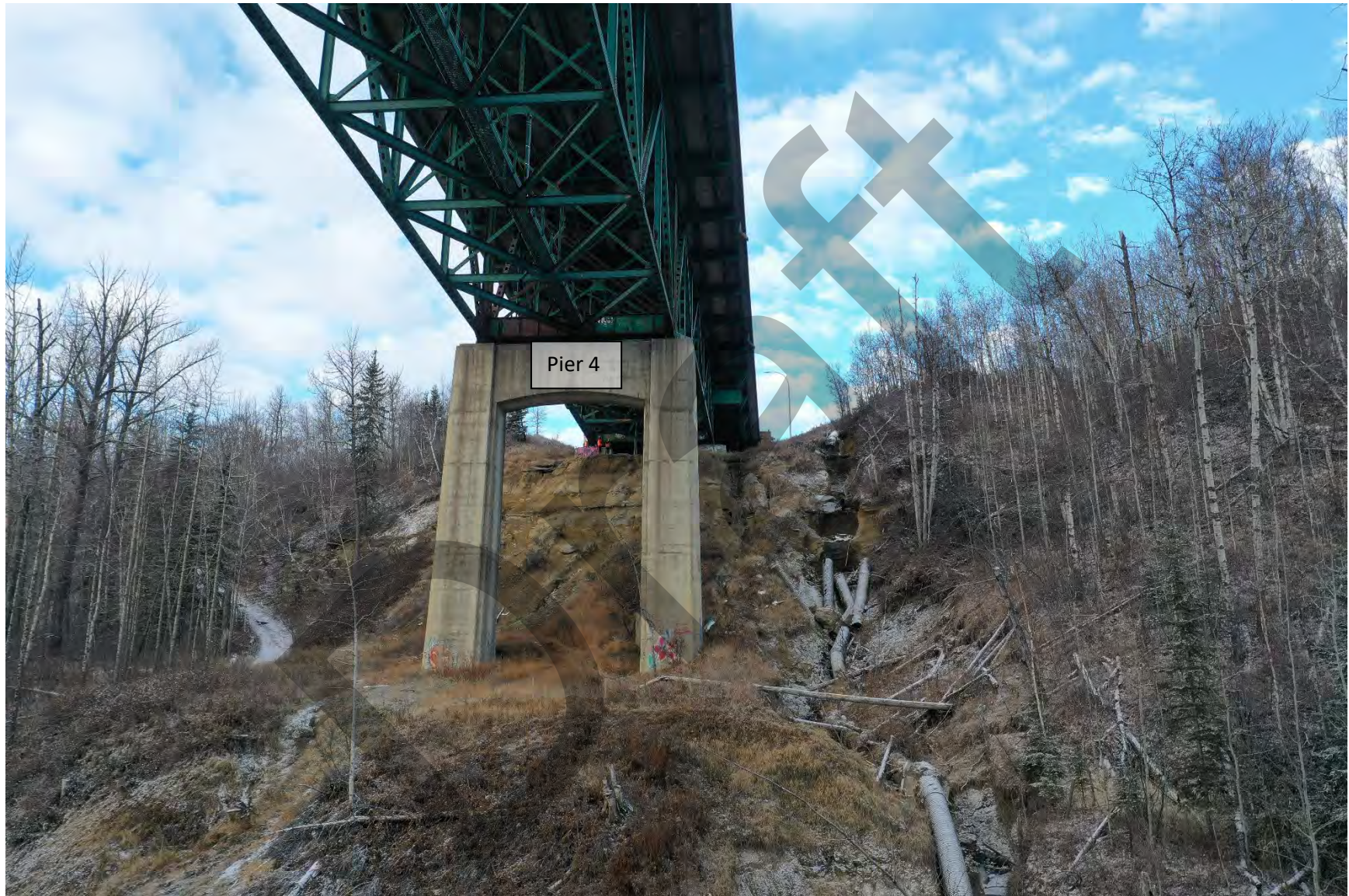
Photo 18: West abutment slope, facing west, showing broken culvers and fallen trees
