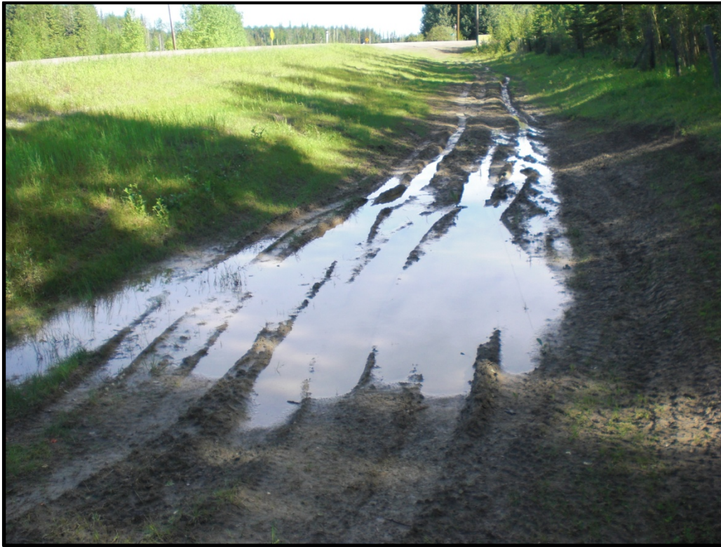
PHOTO 10: Standing water in east ditch, ~100 m south of intersection; facing north.
