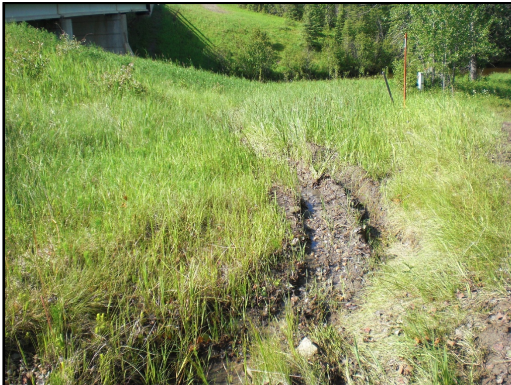
PHOTO 8: South end of erosion gully, west side of north bridge abutment. Note seepage and standing water.
