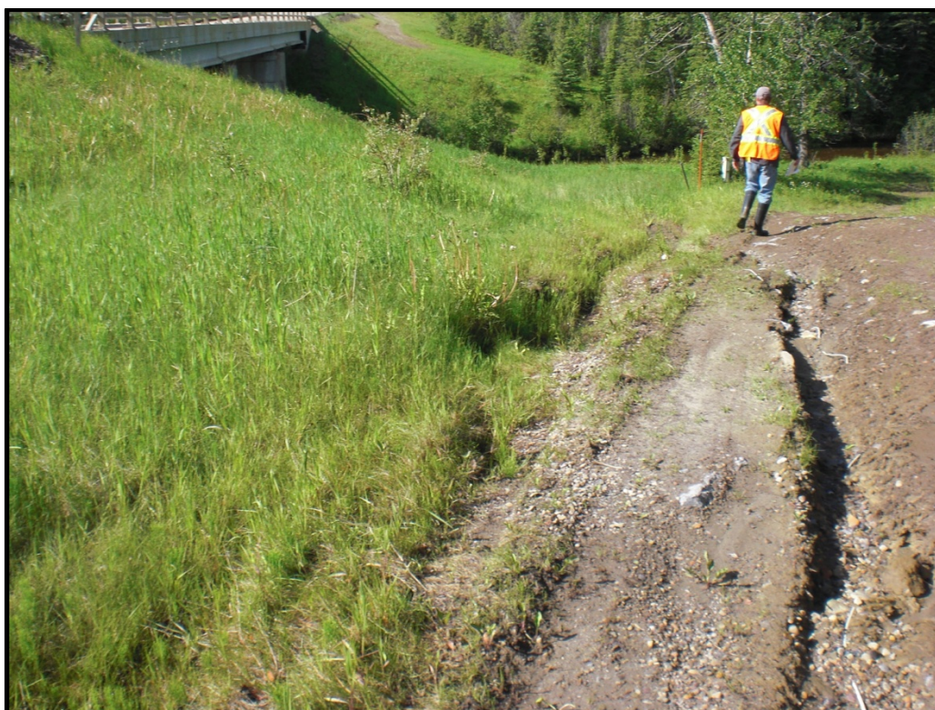
PHOTO 7: Erosion gully, west side of north bridge abutment.
