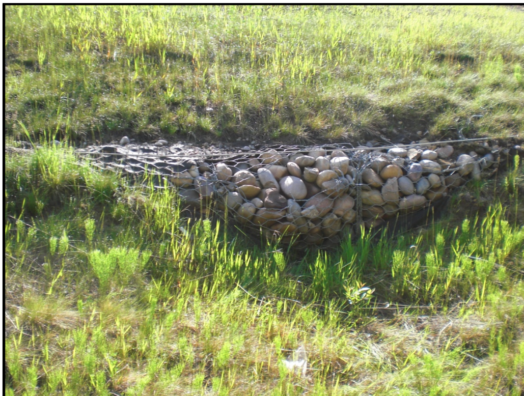
PHOTO 6: Hole in upper gabion wall.
