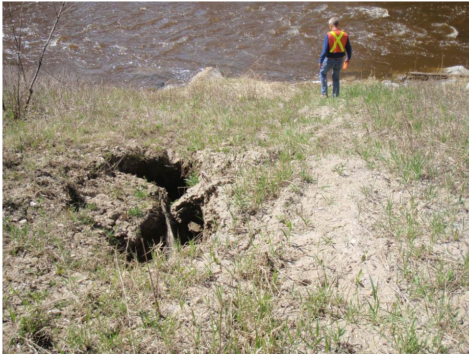
Photo 7 – Sinkhole downslope (south) of the culvert inlet, second sinkhole to right appears to have filled in (May 17, 2011).
