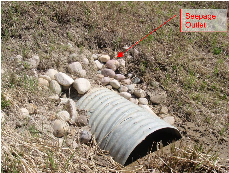
Photo 8 – Culvert outlet near NE bridge quadrant. Note seepage location above and to the right (east) of the culvert and sedimentation at outlet (May 17, 2011).
