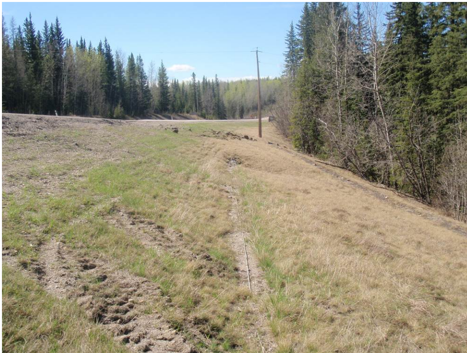
Photo 2 – Looking south at repaired side slope; note rutting near wooden power pole (May 17, 2011).
