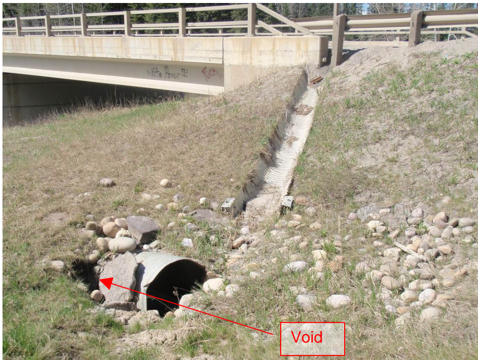
Photo 6 – Culvert inlet and half round down drain at NE bridge quadrant (May 17, 2011).
