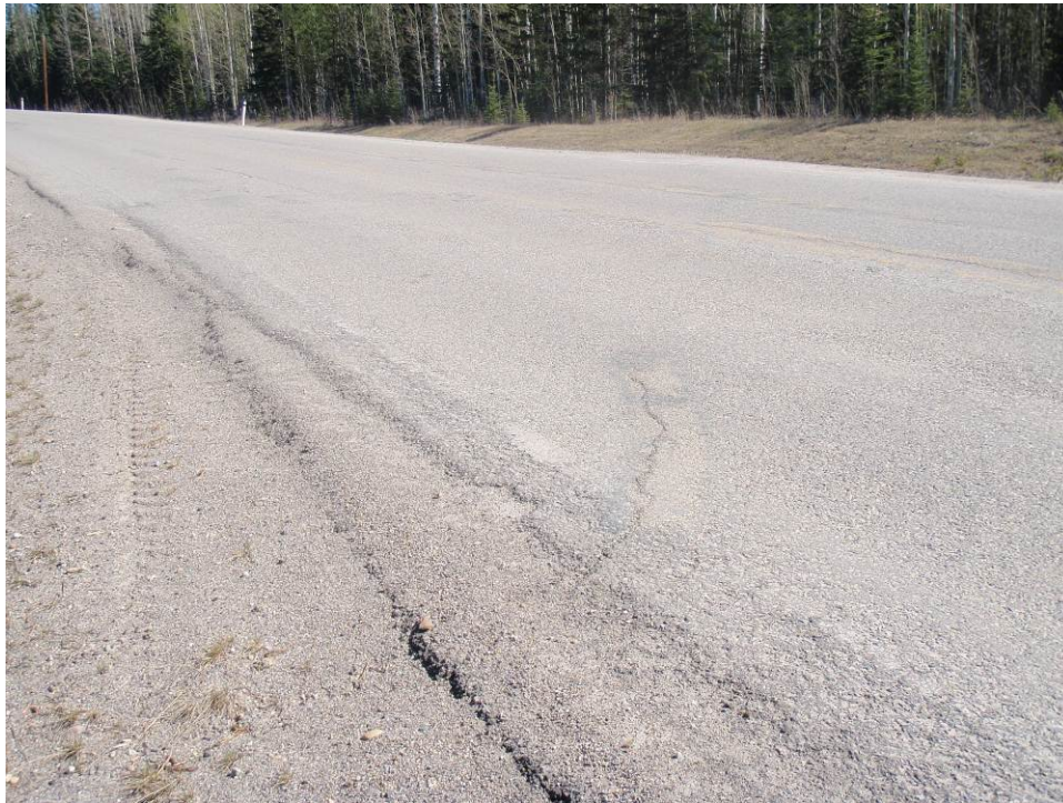
Photo 3 – Crack in south patch area (looking north) (May 17, 2011).
