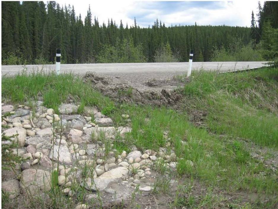
Photo 8 – Accumulated debris on rock apron upstream of guardrail and bypassing ditch flow, June 12, 2008.
