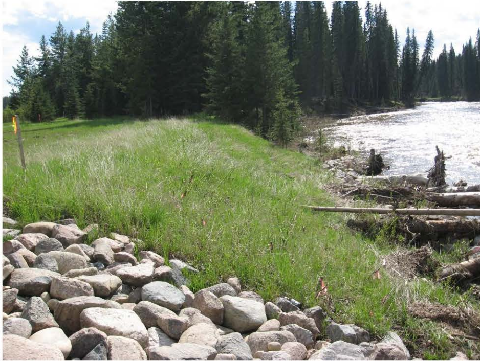
Photo 5 – Looking southwest at repaired slump area at south end of site, June 12, 2008.
