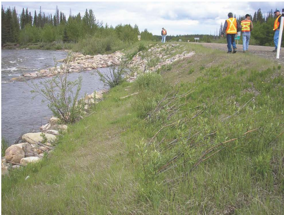
Photo 4 – Looking east (downstream) toward Vane 6 – this had been the slumping section between Spurs 3 and 4, June 12, 2007.
