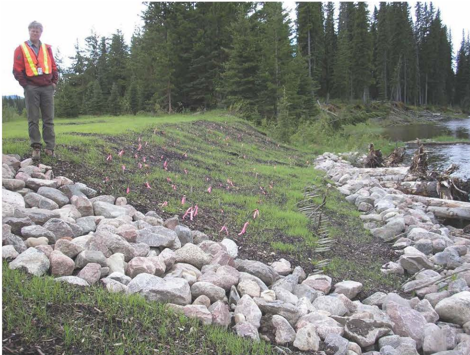
Photo 4 – Looking southwest at repaired slump area at south end of site, June 12, 2007.
