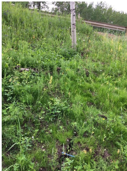
Photo 2: Tension crack near eastern remediation limits. Looking south
