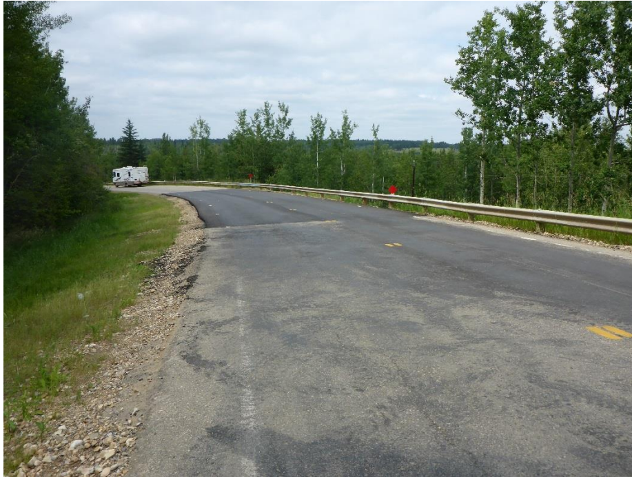
Photo 1: Highway 16A recently patched. Looking north.
