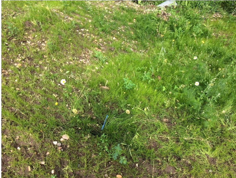
Photo 3: Tension crack upslope from sub-drain. Looking down.
