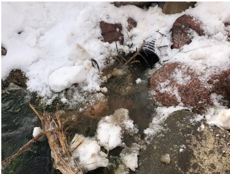
Photo 2: Water flowing out of trench drain outlet on north side of west abutment.
