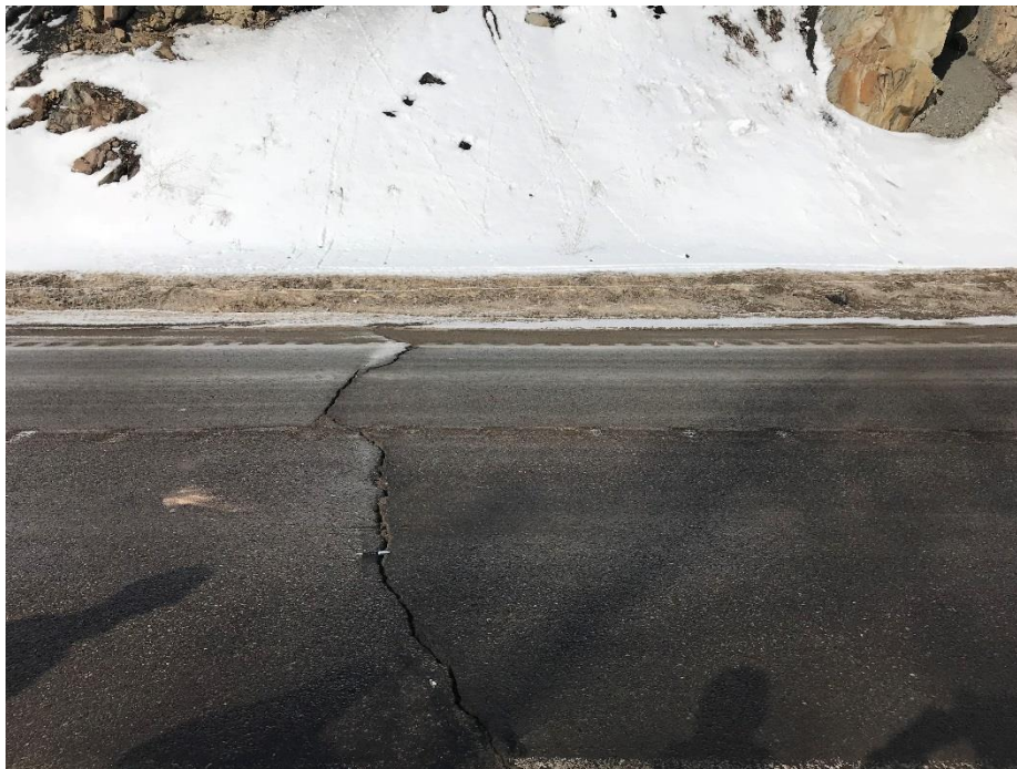
Photo 1: Crack sealed in May 2016 re-opened in 2017. Slight heaving observed. Crack up to 40 mm wide. Looking north
