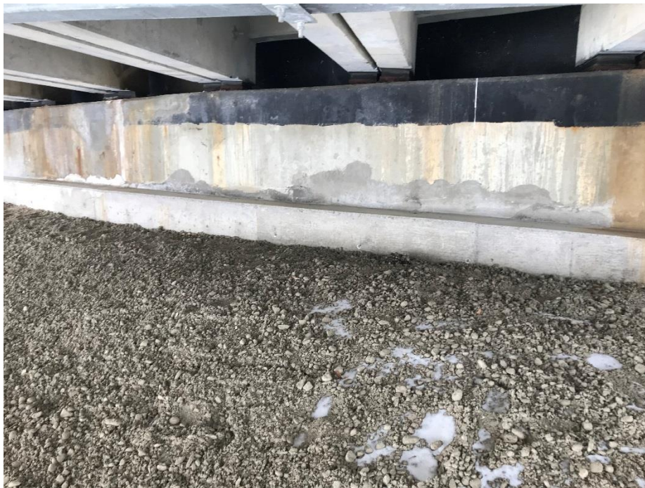
Photo 3: Fill placed over previously observed fill settlement location. Exposed H-piles backfilled. Looking west.
