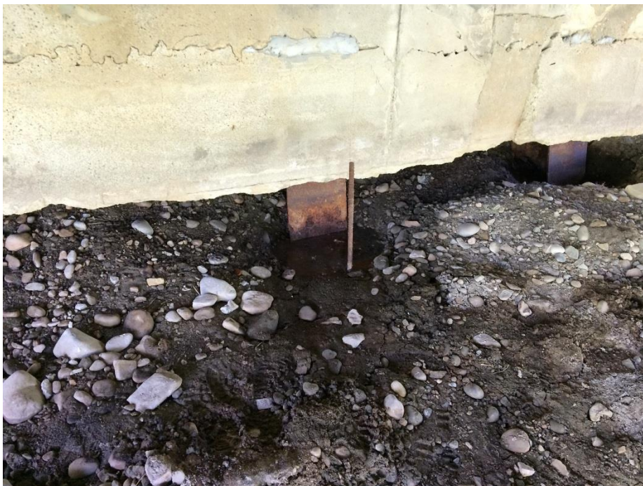
Photo 6: Ponded water at exposed piles. Looking west.
