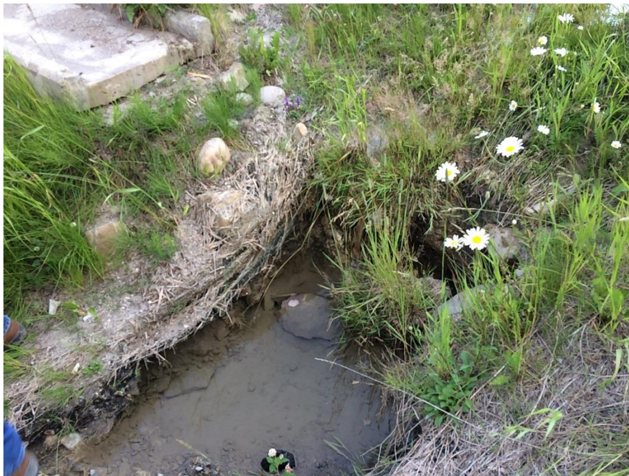
Photo 3: Scour hole at the base of the concrete spillway on the north side of the west abutment.
