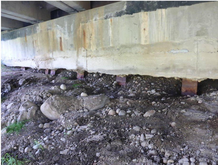
Photo 5: Erosion and fill settlement on west bridge abutment. Looking west.
