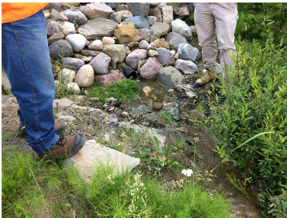
Photo 4: Water flowing through the subdrain installed in 2014.
