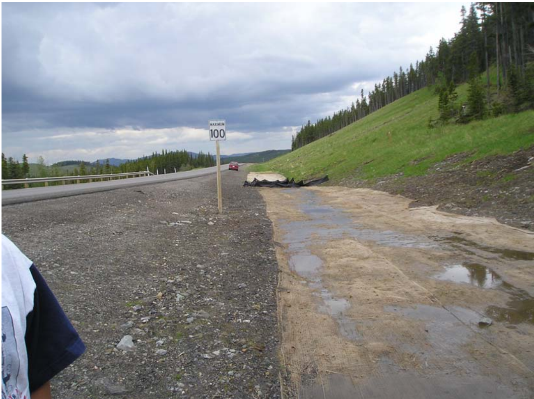
Photo 4 – Ponded water in east ditch (looking north). June 1, 2005
