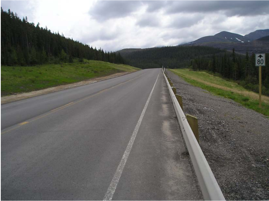
Photo 1 – Previous slide area looking south.
