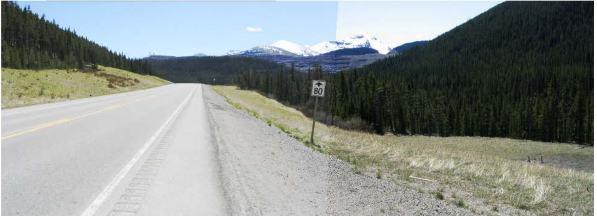
PHOTO 1 - PAVEMENT DISTRESS AREA (LOOKING SOUTH)
