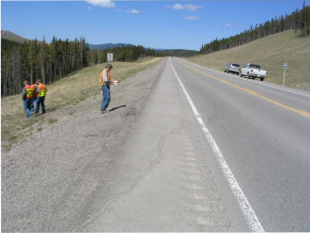
PHOTO 2 - PAVEMENT CRACKS (LOOKING NORTH)
