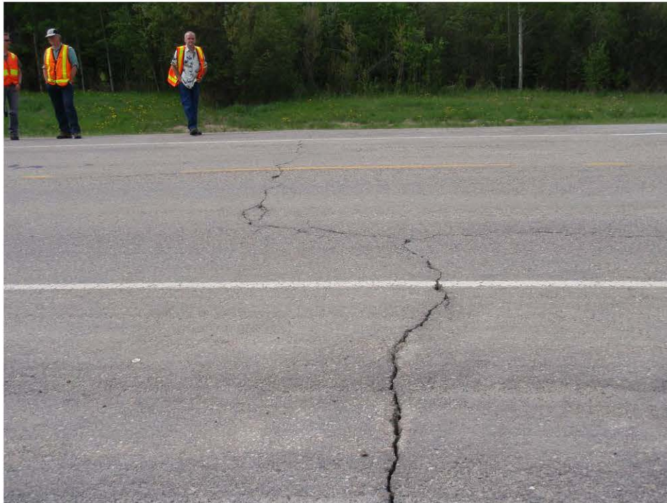
Photo 1 – Looking at crack that formed over Dip 1 (June 15, 2009).
