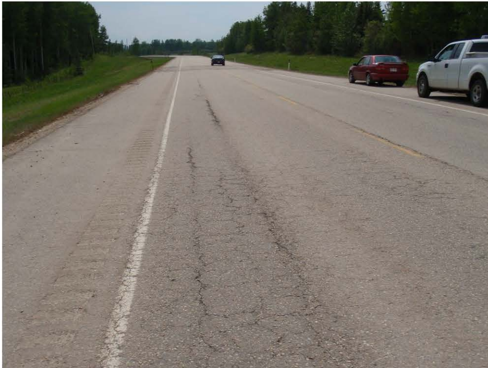
Photo 3 – Looking at pavement fatigue near Dip 2.
