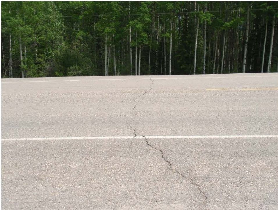
Photo 4 – Looking at transverse crack over Dip 2.
