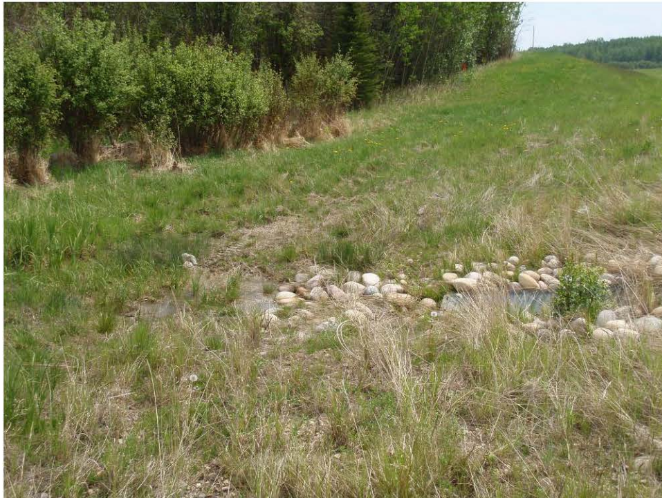
Photo 7 – Ponding water at outlet of culvert at Dip 3.
