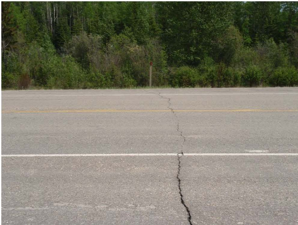
Photo 6 – Transverse crack just north of culvert at Dip 3.
