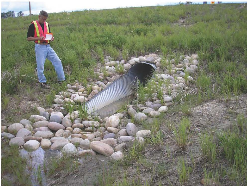
Photo 5 – Ponding water at outlet of culvert at Dip 3, June 11, 2007.
