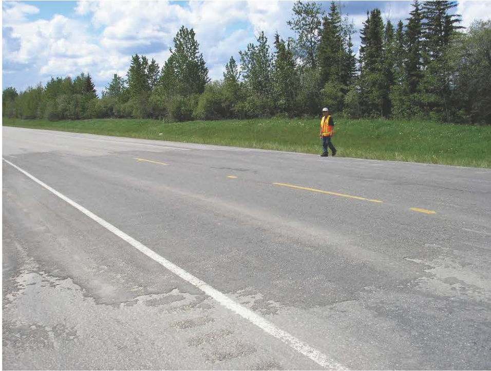
Photo 1 – Looking northeast at patch over Dip 1, June 11, 2007.
