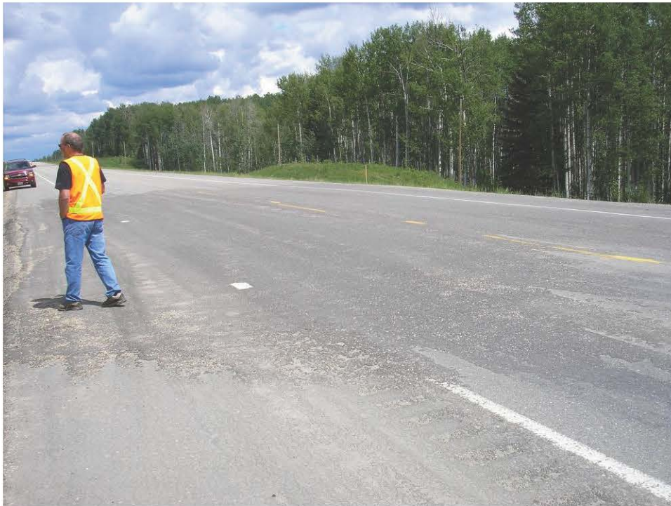
Photo 2 – Looking north at patch over Dip 2, June 11, 2007.
