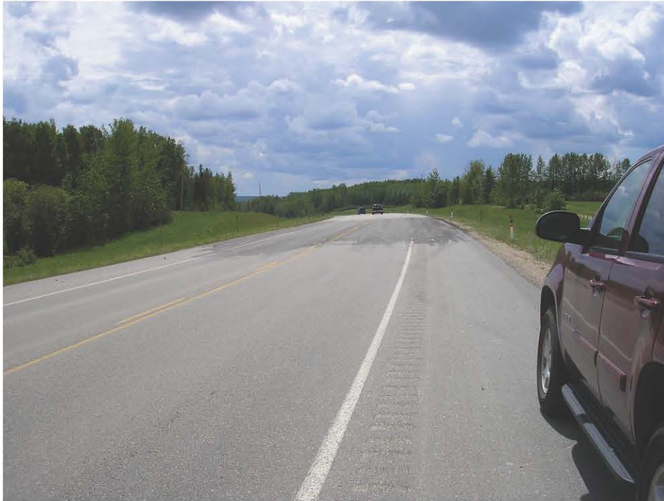
Photo 3 – Looking south at patch over Dip 3, June 11, 2007.
